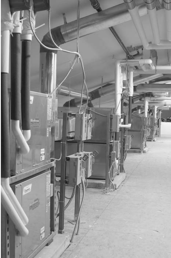
A ground source heat pump, utilizing the local Missoula aquifer, provides the heating and cooling needs for Orchard Gardens. Each unit has individual controls for heating and cooling. © Mark Fritch.
