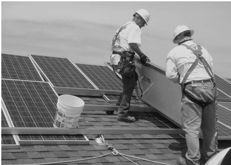
FIGURE 3.11. Installation of photovoltaic panels on the Nuevo Amencer Apartments in Pajaro, CA. Photo courtesy of Pamela Cepe
