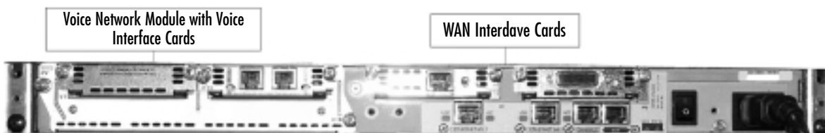
Figure 4.16 Cisco 2611, Rear View
