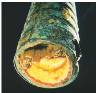
▲ FIGURE 18.22 Scale formation. The interior of this water pipe has been coated with \text{CaCO}_3 and other insoluble salts deposited from hard water.
