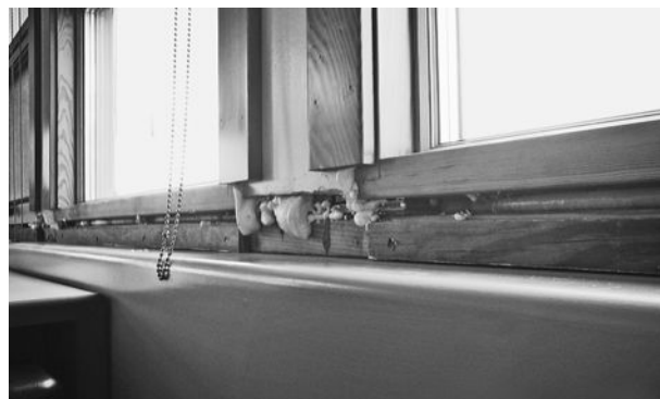
Figure 7-19 This image shows the gap between the window frame and the adjacent rough-opening framing that was discovered during Commissioning as having been left unsealed. The gap size works well, though, when proper sealing of this opening is installed. A gap too small cannot be properly sealed and will be a significant source of infiltration. Image courtesy Brian Toevs.
