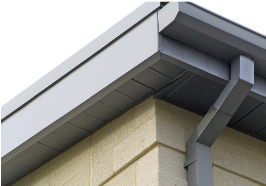
Figure C-3 The exterior of this building in the northeast U.S. appears to be well constructed; however, upon further inspection, the thermal envelope has failed where the exterior walls meet the roof. In this case, the attic space above the ceiling (inside the thermal envelope) has been as cold as 36°F during winter months. The infrared images depicted in Figures C-4 through C-6 reveal thermal bridging conditions, problems that are common due to lack of proper envelope detailing and/or installation during construction. The commissioning process can help project teams avoid such problems. Image courtesy of Brian Toevs.
