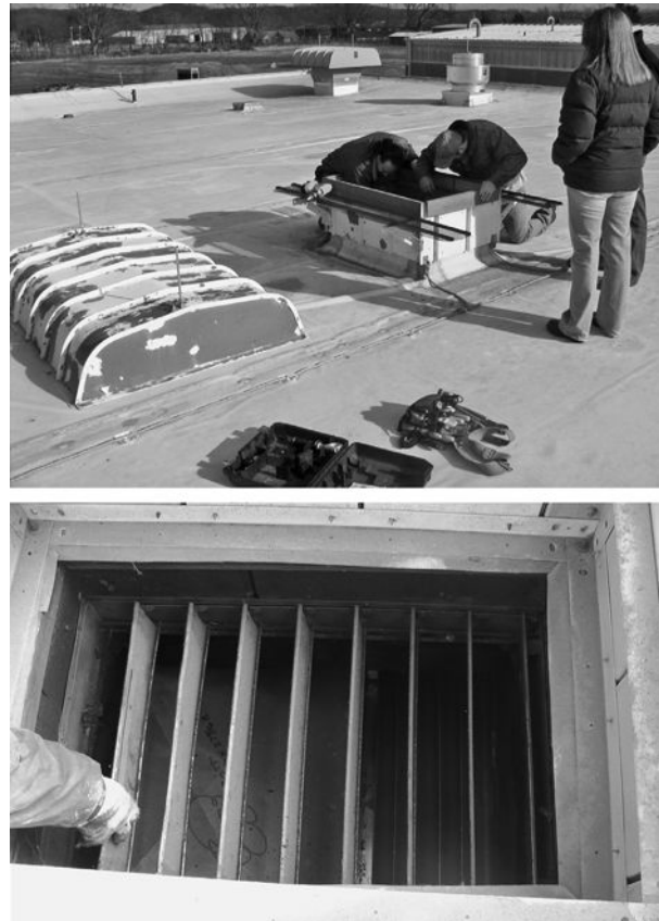
Figure 8-3 Top image: Functional testing of a new makeup-air unit tied to this existing hood and roof opening for outside air intake resulted in no airflow, but we could not understand why. Everything else we tested and checked on the system worked fine, but from below we could not see up into this roof opening. We wanted to uncover the mystery, so we removed the hood without knowing what we would find.
