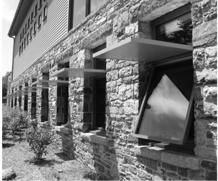
Figure 6-22 Exterior light shelves shade the lower vision glass from high-altitude direct solar penetration in the summer, while bouncing daylight through the upper daylighting glass deeper into the space. Image courtesy of Todd Reed.
