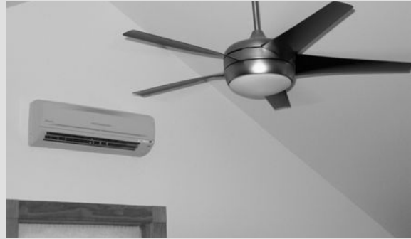
Figure 5-19 Ceiling fans are a viable, adaptive thermal comfort strategy that increases airflow and enables temperature set points to be higher in the cooling season. The use of ceiling fans during the heating season to circulate warm air at the ceiling is a persistent energy myth. This practice does not save energy nor does it enable lower heating season temperature settings. Image courtesy of Marcus Sheffer.
