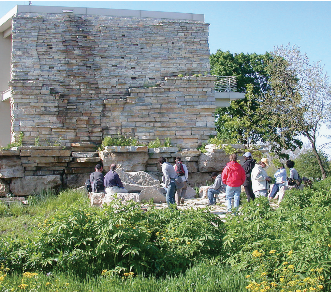
Figure C-14 Water passes through the roof scupper at the rear of the Peggy Notebaert Nature Museum, contributing artfully to the beauty of the project's cliff wall and educational garden. Image © Conservation Design Forum, Elmhurst, IL, www.cdfinc.com .
