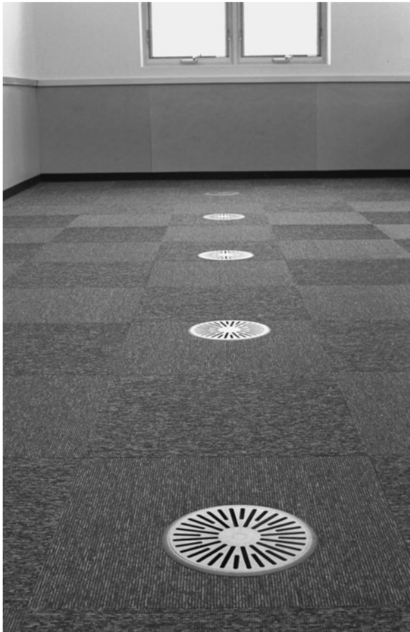
Figure 7-18 Floor diffusers for underfloor air distribution (such as these manufactured by Krantz) serve as metering devices that afford occupants individual thermal-comfort control. Image ©2001 Jim Schafer.
