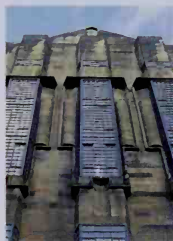
Mackintosh built the west wing of the Glasgow School of Art, housing the library, in 1907–9.
