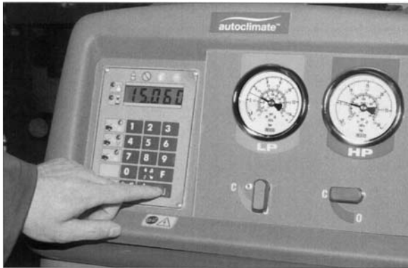
Figure 5.17 Record the weight of refrigerant recovered
