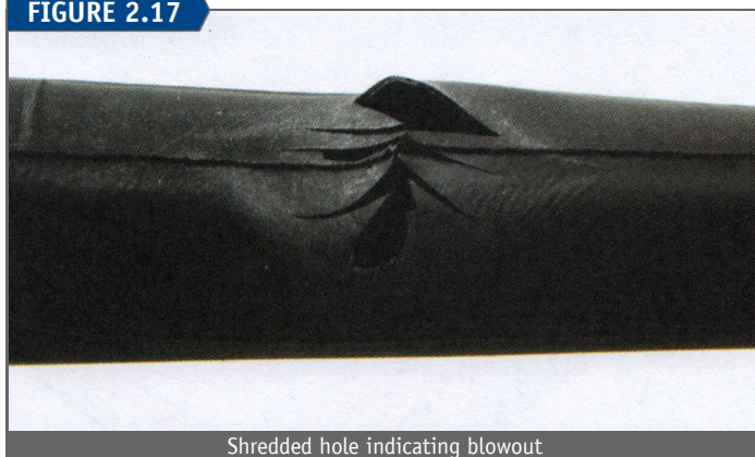
Shredded hole indicating blowout
