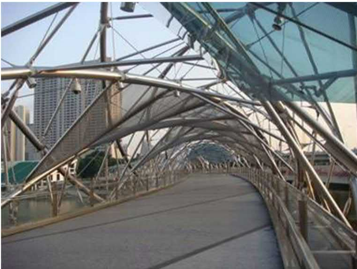
FIGURE 3.19 Spiral metal walkway.
