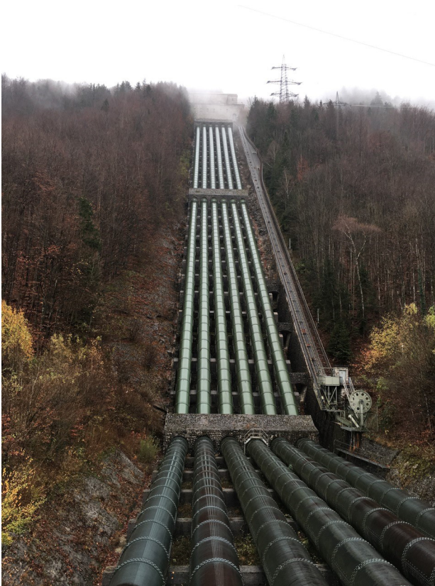
The hydroelectric power facility in Walchensee near the Austrian-German border. Courtesy of Miranda Schreurs.
