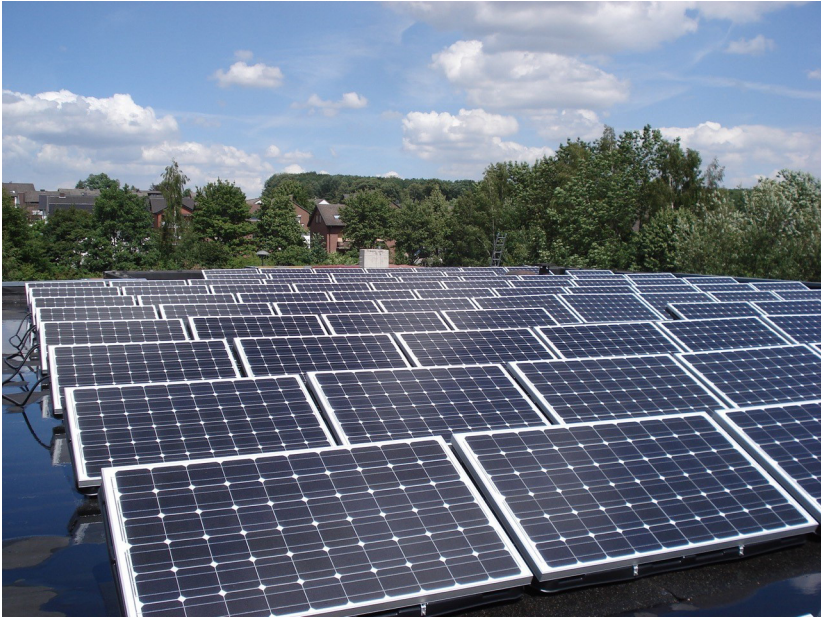
Solar photovoltaics in Germany. Courtesy of Alois Plüster.
