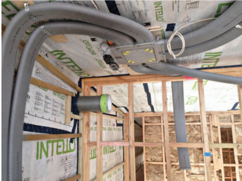
Manifold and ducts run interior of the airtightness layer. Only one penetration of the airtightness layer is necessary (Photo: Murray Durbin).
