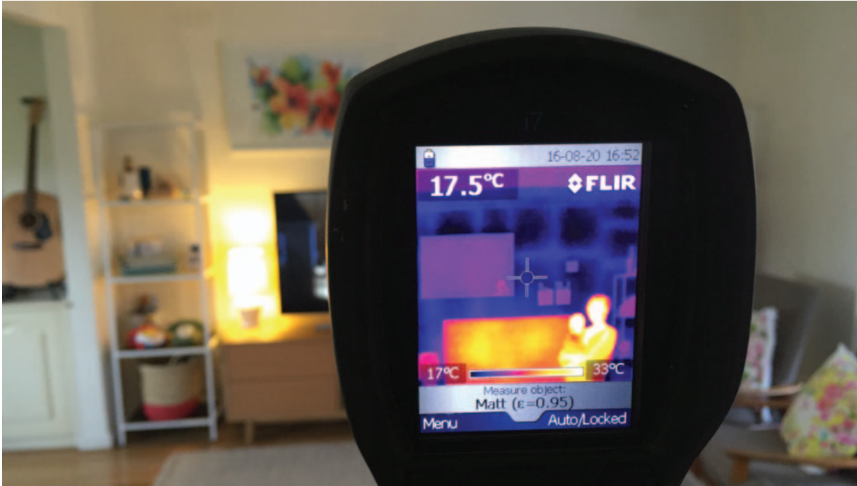
Infrared photo showing radiant heat emitted from occupants and appliances, and heat loss through the uninsulated wall.
