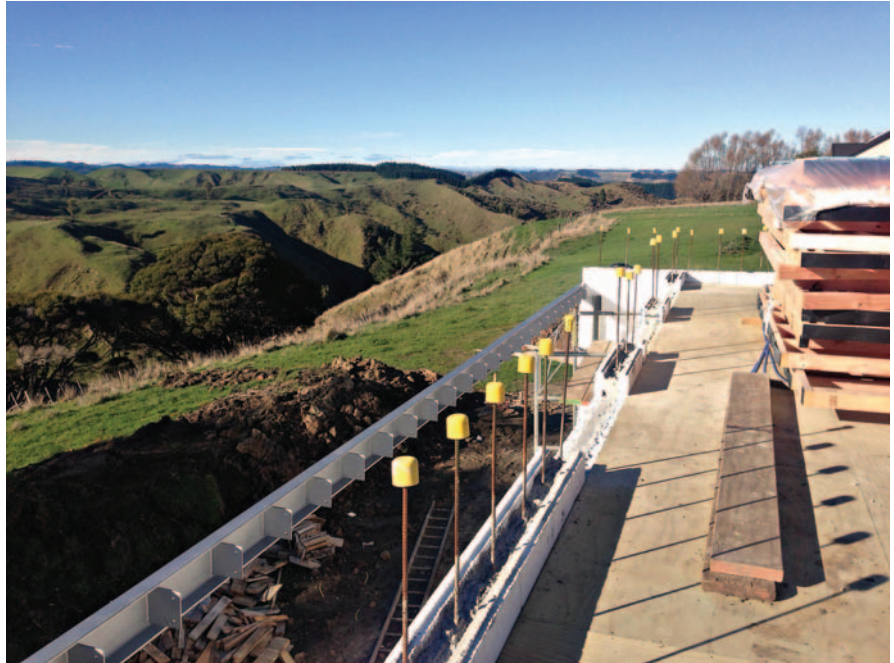
Insulated concrete form blocks are filled with concrete (Photo: ecoBuild Developments Ltd).
