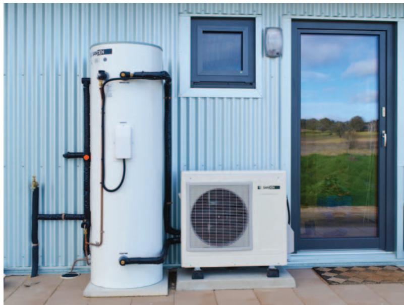
Domestic hot water heat pump and storage tank (Photo: Faud Abdi).
