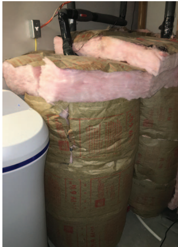
Example of retrofitted hot water tank and hot water pipe insulation (Photo: John Loveless).
