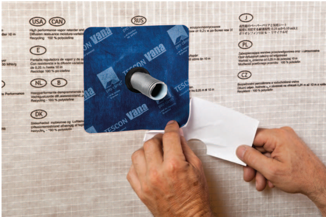
Sealing pipes and ducts to the airtightness layer (Photo: pro clima Moll bauökologische Produkte GmbH).
