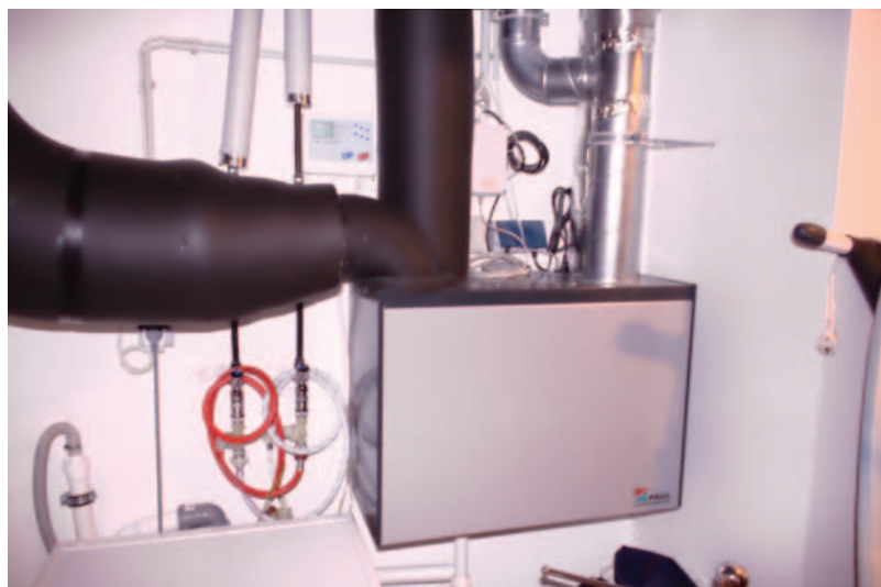
Heat recovery ventilation unit installed in the basement of this terraced house.
