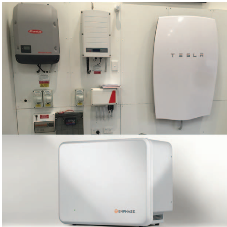
Example of a DC storage system (top) showing a Tesla Power Wall, inverter, power meter, switchboard and web box (Photo: Energy Matters), and an Enphase AC storage unit (bottom) (Photo: Enphase Energy).
