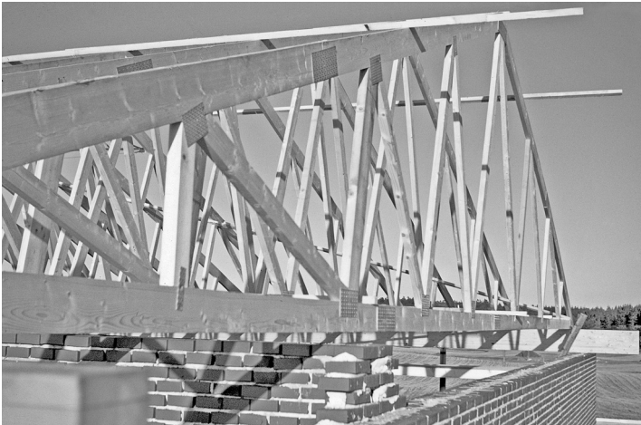
Fig. 3.2 Trusses with punched metal plate connectors spanning from façade to façade. The members carrying the roof covering are not shown
