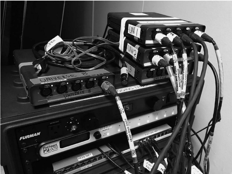
FIGURE 12.13 Rack-mounted Ethernet/DMX data distribution station.
