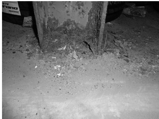
FIGURE 14-26d Corroded steel column base (Courtesy of Jason Vigil, P.E., S.E.)
