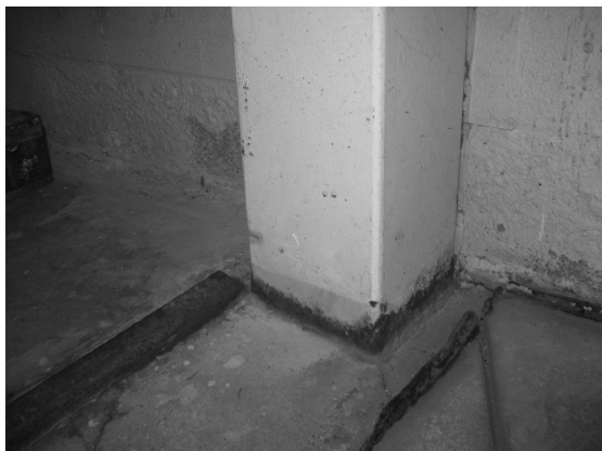
FIGURE 14-26e Corroded HSS column base (Courtesy of Jason Vigil, P.E., S.E.)
