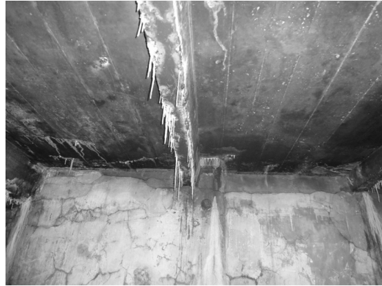
FIGURE 14-26b Corroded steel beam (Courtesy of Jason Vigil, P.E., S.E.)
