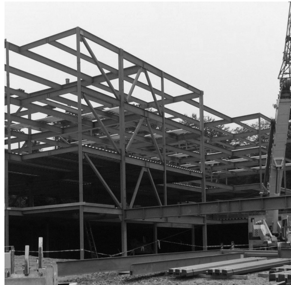
FIGURE 1-21c Braced frames: Single diagonal and Chevron braces in a steel building under construction (Photo by Abi Aghayere).
