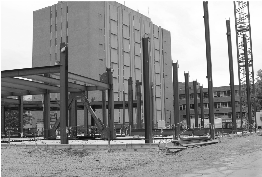
FIGURE 1-21a Braced frame and columns in a multi-story steel building under construction (Photo courtesy of Obinna Otti)
