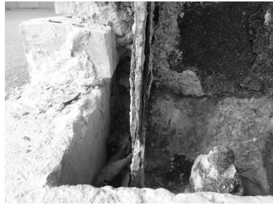
FIGURE 14-26h Corroded steel column in exterior wall (Courtesy of Jason Vigil, P.E., S.E.)
