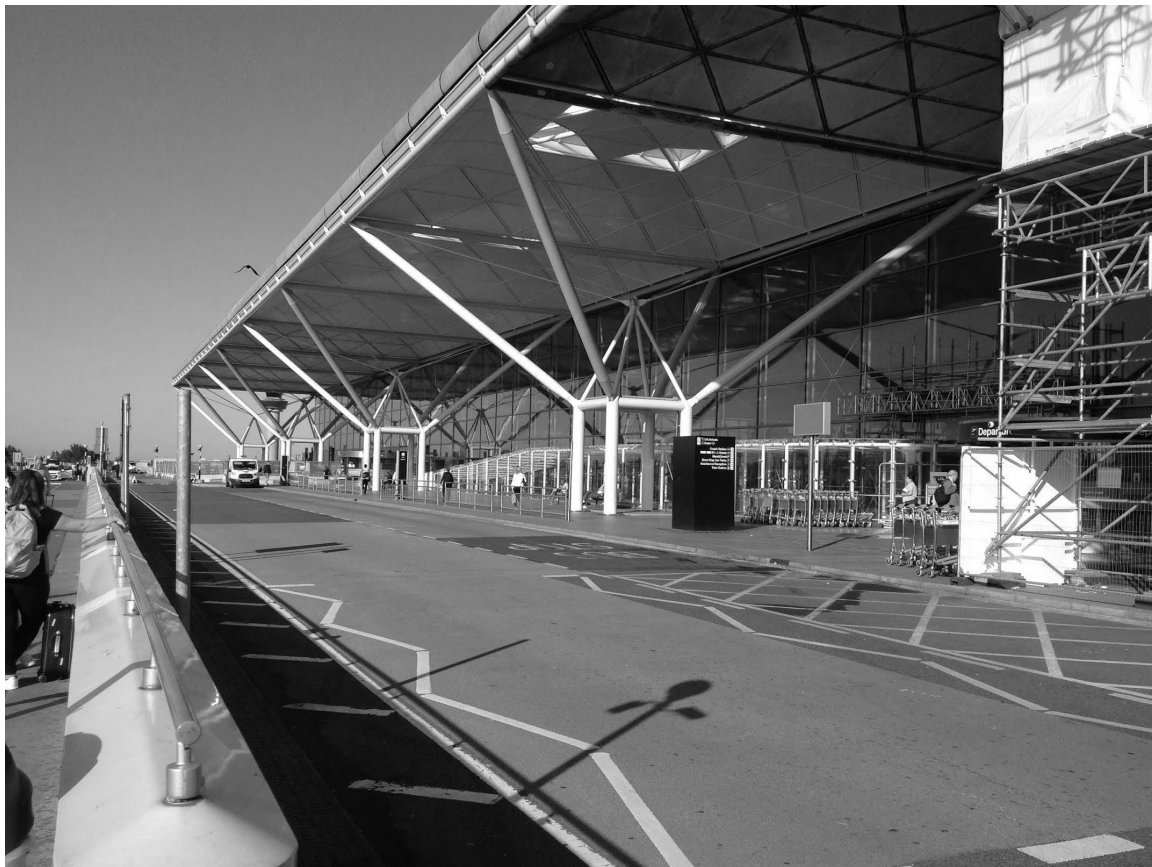
FIGURE 5-1b Struts, tie rods, and columns at an airport entrance canopy (Photo by Abi Aghayere)
