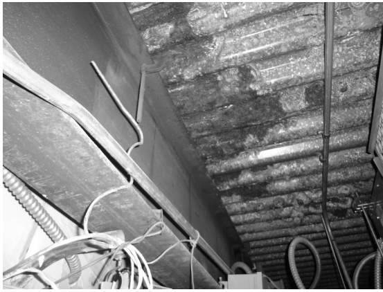
FIGURE 14-26g Corroded steel beams and floor deck (Courtesy of Jason Vigil, P.E., S.E.)
