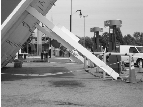
FIGURE 14-26a Canopy collapse due to exterior HSS column corrosion (Courtesy of Darren A. Brooks, P.E.)
