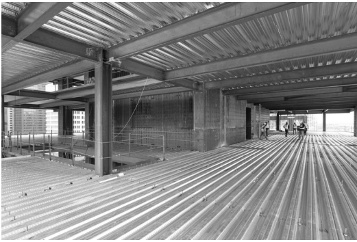
FIGURE 7-2a Steel beams and girders with composite metal deck and steel studs (Courtesy of Magnusson Klemencic Associates)
