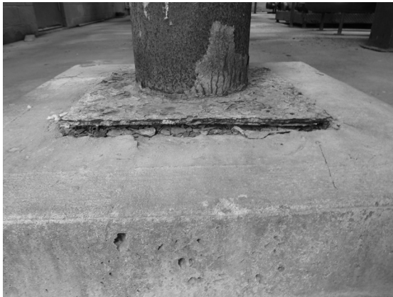
FIGURE 14-26i Corroded exterior steel column (Courtesy of Jason Vigil, P.E., S.E.)
