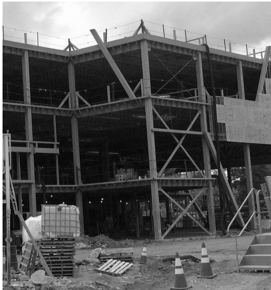
FIGURE 1-21b Braced frames: Plate and steel rod X-braces in a steel building under construction (Photo by Abi Aghayere).
