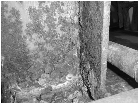
FIGURE 14-26c Corroded steel column base (Courtesy of Jason Vigil, P.E., S.E.)
