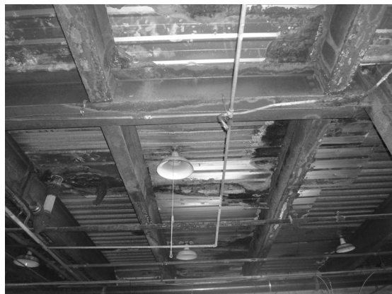
FIGURE 14-26f Corroded steel beams and floor deck (Courtesy of Jason Vigil, P.E., S.E.)
