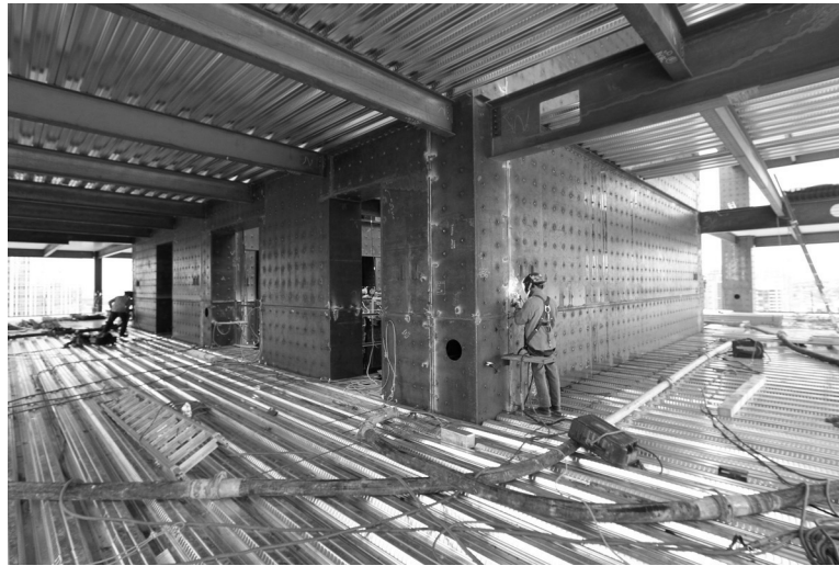
FIGURE 3-8c Steel plate composite shear walls (Speedcore) under construction (Photo courtesy of Magnusson Klemencic Associates)
