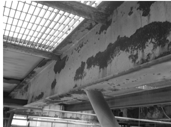
FIGURE 14-26j Corroded exterior steel framing (Courtesy of Jason Vigil, P.E., S.E.)
