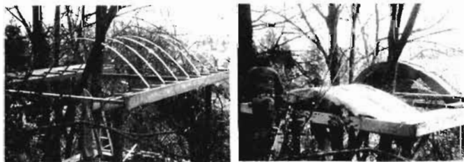
Another version of a roof vault, built by Bob Harris in Oregon.
