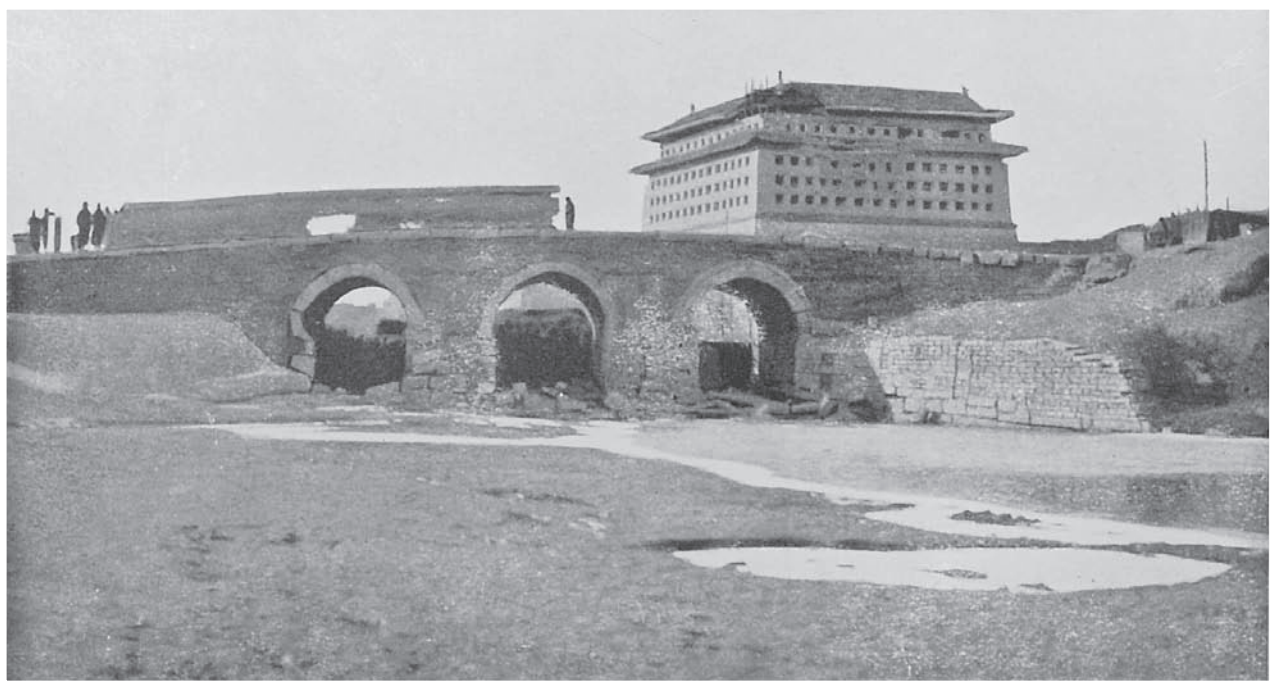
The stone arch bridge in this photograph is quite run down and so is the watchtower nearby, where one corner of its roofs has disintegrated.
