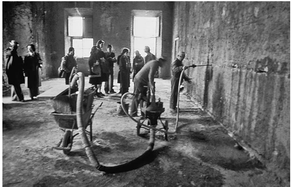
Figure 1-8 Cement grout injection during a 1977 restoration as a structural stabilization measure at the Ospedale di San Michele complex in Trastevere, Rome, is illustrative of one of several conservation-engineering techniques developed in Italy.
