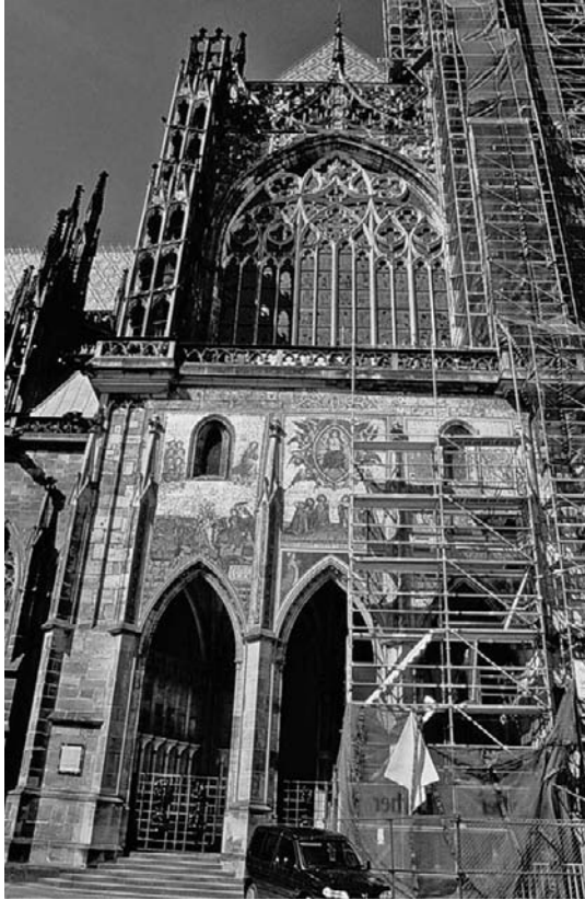
Figure 16-3 Restoration of the elaborate mosaic ornamentation (a) above exterior portals of St. Vitus Cathedral (b) at Prague Castle was made possible by technical analysis and funding provided by the Getty Conservation Institute in 1999. The project included a training component for local conservators and extensive monitoring has been ongoing since its completion.
