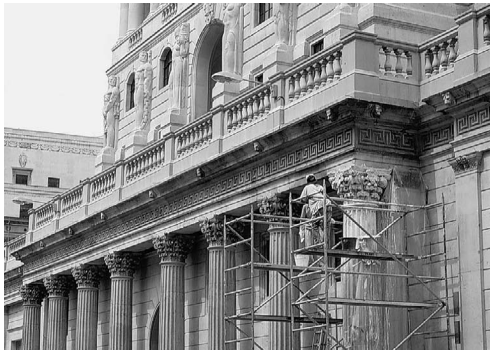
Figure 3-15 Repairs and cleaning of the fire damaged Bartholomew Street facade of the Bank of England by Donald Insall Associates Ltd.
