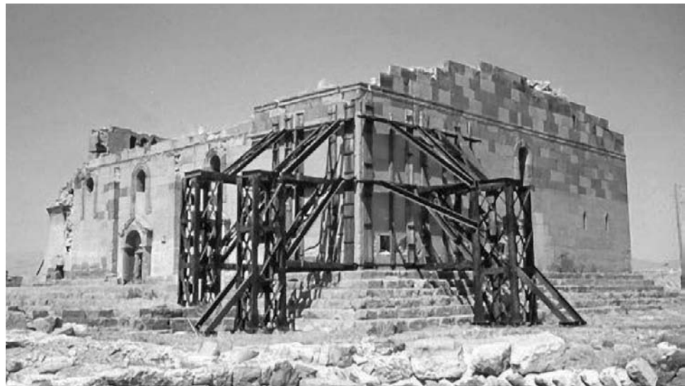
Figure 20-4 The fifth-century church of Ererouk in western Armenia is the country's earliest freestanding basilican form. A corner of the building that was in danger of collapsing in 1992 was temporarily shored in 1993, in an American-funded effort, until economic conditions in the country improved to permit more extensive measures. Preparation for this intervention included development of a site management plan.
