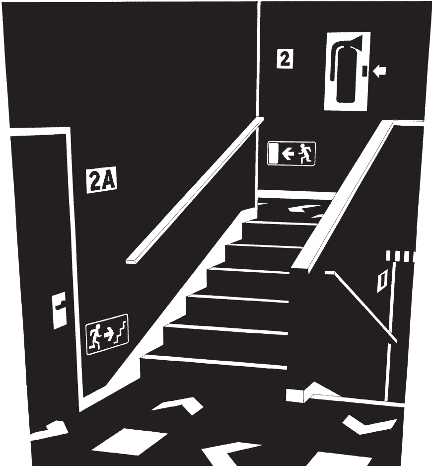
Fig. 6-32. Luminous escape route trim.
