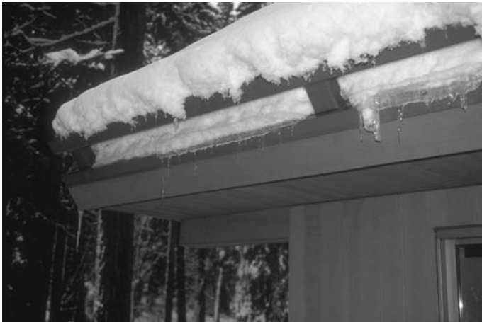
3.12 Structurally designed snow arrester. Note: heat tracing in gutter not powered at time of photo (Matrix IMA Archive photograph).
