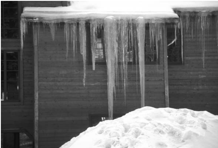
3.17 Snow up against building. Note: top of window just above ground snow. Window head is \pm 10 feet (3.048 m) above grade (Matrix IMA Archive photograph).
