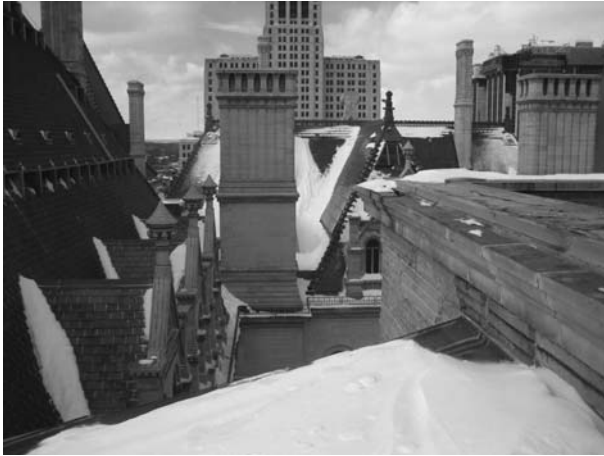
4.2 Gutters and drainage trough waterproofing height must be sized based on an anticipated height of snow accumulation.
