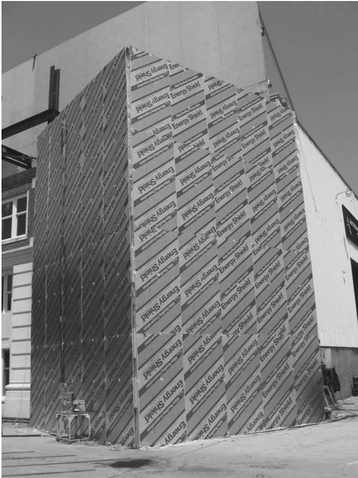
9.6 Three-story (32 feet) insulated enclosure is used for thermal cycling of a large preconstruction mock-up with outside 90° corner condition.
