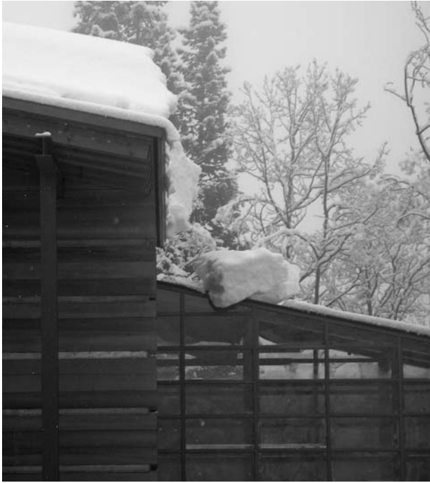
3.11 Snow cantilever calving impact damage to sloped glazing/ greenhouse 2 to 12 roof. Note: snow inside enclosure (Matrix IMA Archive photograph).
