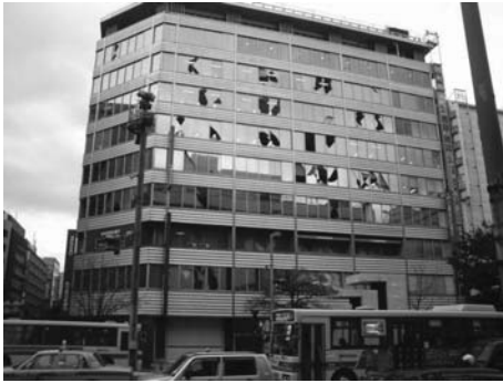
2.15 Glass breakage in strip window system during Fukuoka (Japan) (magnitude 7.0) Earthquake of March 20, 2005 ( answers.com/topic/2005-fukuoka-earthquake ).
