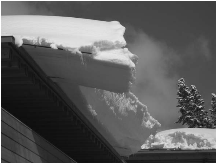
3.8 Snow creep cantilever. Metal standing seam 2 to 12 cold roof. Note: ripped away snow fence bars (Matrix IMA Archive photograph).
