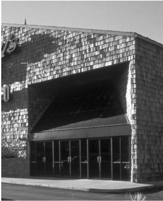
3.9 Fully sheltered sloped glazing entry below main roof rake (Matrix IMA Archive photograph).
