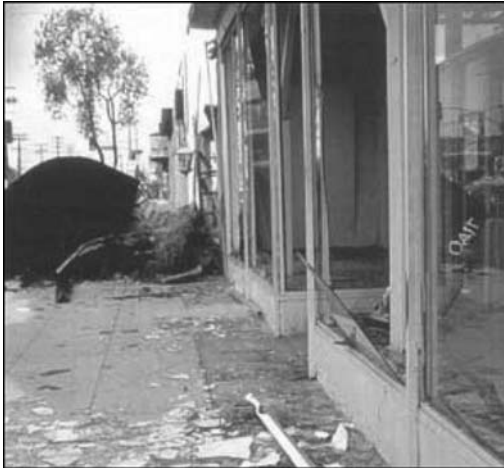
2.13 Damage to storefront during Northridge (magnitude 6.7) Earthquake of January 17, 1994 (FEMA News Photo, FEMA, Washington, DC).
