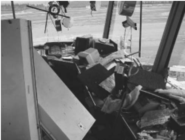
2.14 Glass damage to airport control tower during Seattle (Nisqually) Washington (magnitude 6.8) Earthquake of February 28, 2001 (propertyrisk.com/refcentr/seattleeq; photo by ABSG Consulting, 16855 Northchase, Houston, Texas 77060, www.absconsulting.com).
