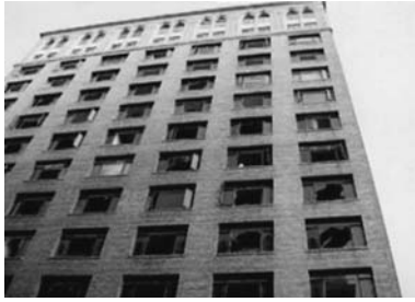
2.11 Glass breakage in punched window system during Loma Prieta (magnitude 6.9) Earthquake of October 17, 1989 ( Oaklandlibrary.org/oaklandhistory/earthquake89 ).
