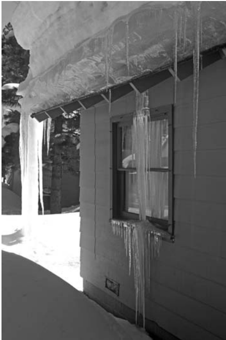
3.15 Large ice dam at cold roof overhang. Note: primary icicles have been removed (Matrix IMA Archive photograph).
