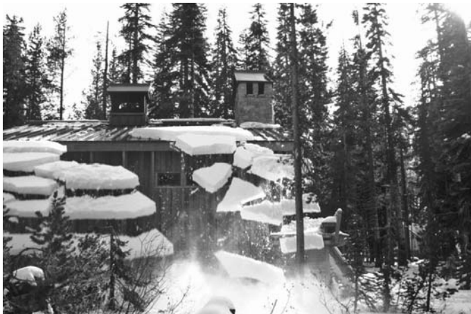
3.7 Sudden roof snow avalanche. Metal standing seam 4 to 12 cold roof (Matrix IMA Archive photograph).
