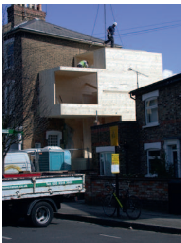
Focus House – solid timber panels being craned into position credit: Bere Architects
