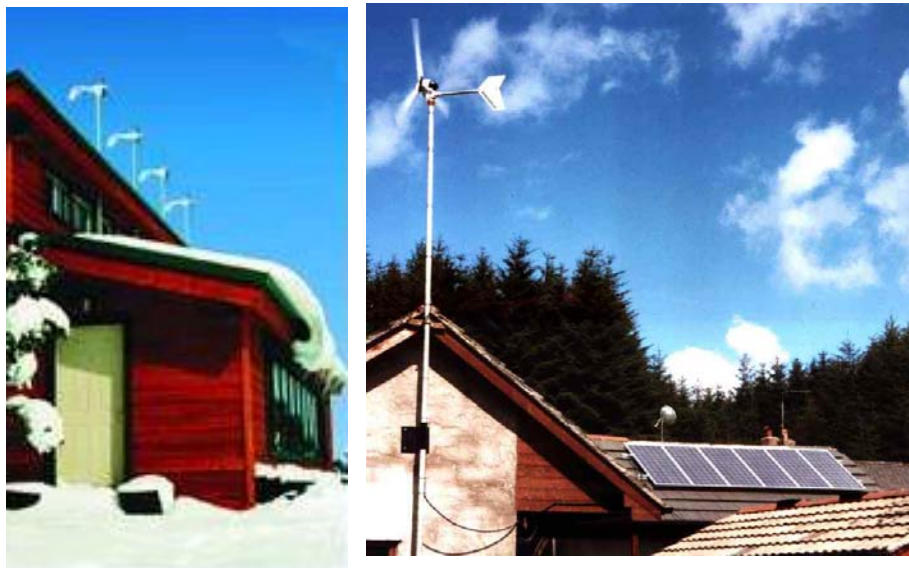
Figure 2-8: SouthWest Windpower AIR 303 turbines installed on a US building 72 (left) and Windseeker 503 turbine installation on a building in the Kielder Forest
