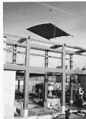
17 | Erecting the first roofing panel on an H-frame block. The projecting timber members are for the overhanging eaves at the gable.
