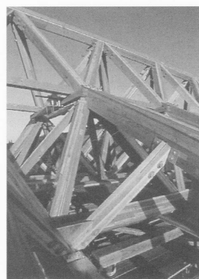
10 | The junction of the triangular cross-bracing for the clerestory sides, horizontal and inclined incoming main rafters.
