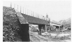
7 | Erecting the protective cladding and the posts for the balustrading from a movable platform.
