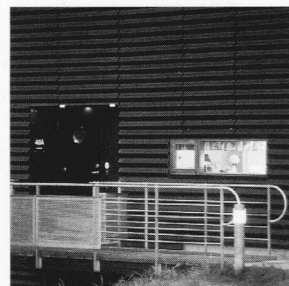
8 | Elevation showing horizontal profiled fibre-reinforced cement cladding and untreated wood windows. The supporting structure for the elevated entrance walkway is made from hot-dip galvanized steel.
