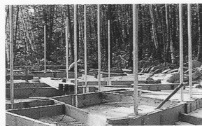
10 | The foundation during construction. Visible are the compound sole plates with their stiffening members and bolted retaining poles. The bays have not yet been filled with sand.
