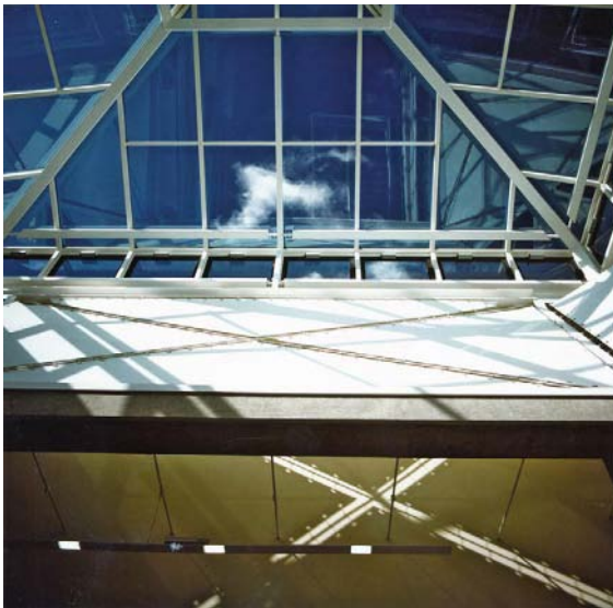
The naturally ventilated atrium at The Queens Library, Anglia Polytechnic University. Designed by ECD Architects. (Anglia Polytechnic University)
