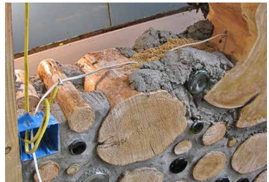
9.10. A double-wide box fastened to a door frame (left side of image) will provide switches for an overhead light, as well as the LED light inside the crystal skull's hollow log (right side), as described in Chapter 8.
