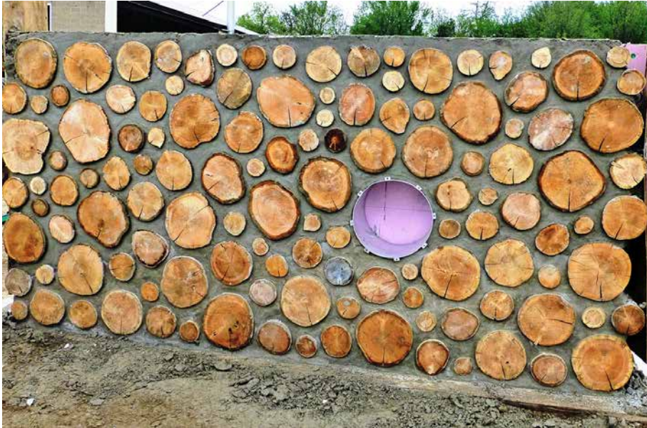
14.3. Each log-end in the 5-foot by 10-foot training panel for the Arcus Project was measured accurately. By area, the panel is 60 percent wood and 40 percent mortar. The round hollow area is rigid foam behind a special light window being tested, and counted as a large log-end.
