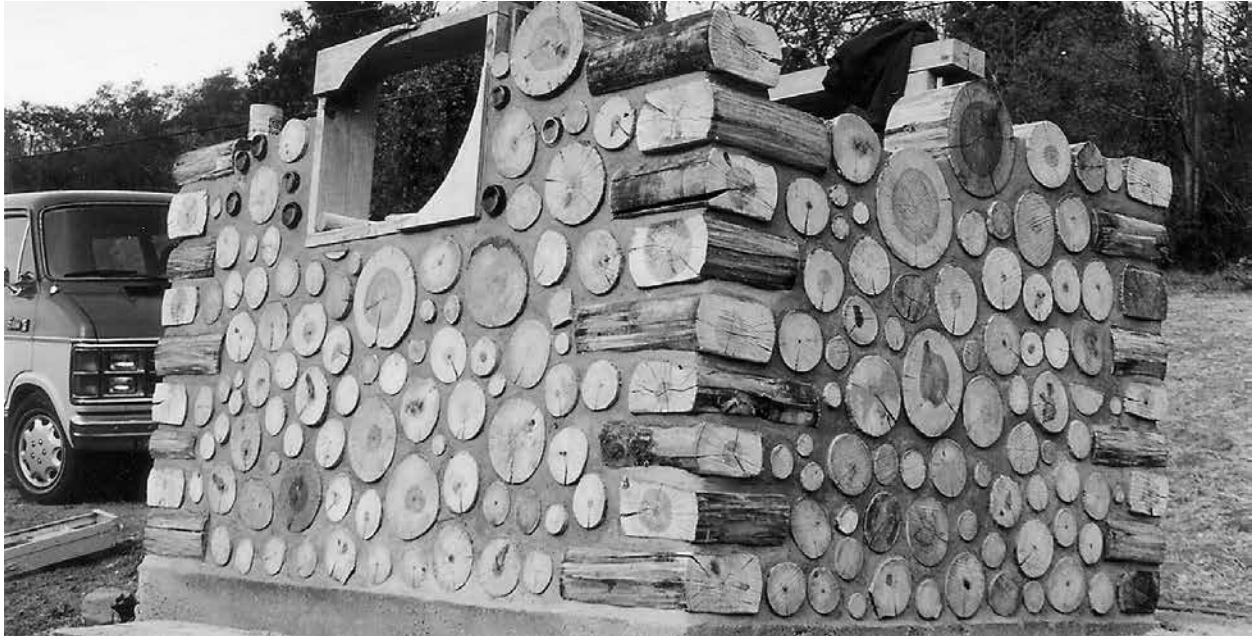
1.9. This small pump-house in North Carolina was made with single-wide quoins, cut from tulip poplar with a chainsaw, then water-sealed to minimize water absorption from mortar to wood. The staggered length of the quoin is clear in this image.
