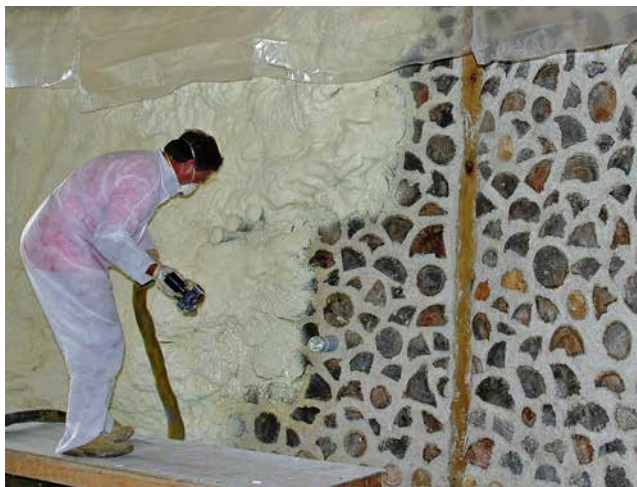
7.1. Open cell foam is sprayed onto the inner surface of Alan's exterior cordwood wall. Photo by Alan Stankevitz.
