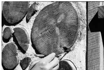
4.7. The slurry or mortar is painted on and pressed into the caulk, then blended out to the surrounding mortar. Credit: Geoff Huggins
