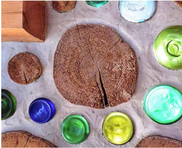
4.2. A large primary check needs to be filled.
