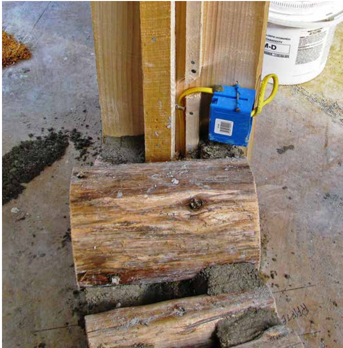
9.9. A view of the other side of the door frame shows the key pieces more clearly, as well as the first course of cordwood masonry.
