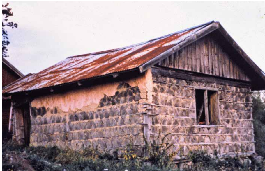
P.3. This old house in Botkyrka, Sweden, dates back to about 1860. Despite a foundation of stones on the ground, unbarked spruce log-ends, a clay and sawdust mortar, and more than 60 years of neglect, the walls are mostly intact. Olle Hagman visited the same house in 2015 and reported that one side of the roof was ruined and so one wall was starting to rot. Credit: Olle Lind.
