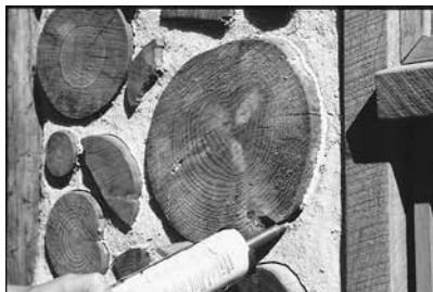
4.6. A small wedge beneath the log pushes it up so that the biggest gap is on the bottom, where it is less visible. Next, the gap is cleaned of loose mortar with any sharp tool, such as a nail (not shown). Particles and dust can be blown away with a small rubber hose. A bead of latex or acrylic caulking is applied and then smoothed with a popsicle stick, pointing knife, or finger. Credit: Geoff Huggins
