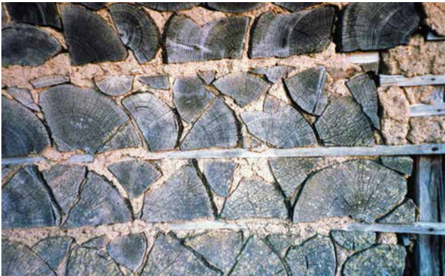
P.4. Wall detail of the Botkyrka house. Note the use of horizontal boards as stabilizers between courses. The mortar is a mixture of clay and sawdust. Credit: Olle Lind.
