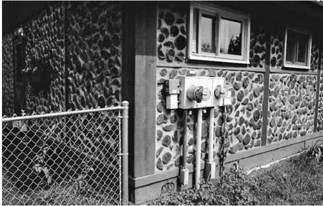
9.1. Power is brought underground to the service entrance at this suburban cordwood home in Eau Claire, Wisconsin.
