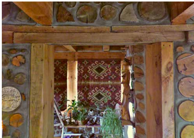
1.12. Top of door frame at Earthwood, made from doubled 4-inch by 8-inch jambs and header.
