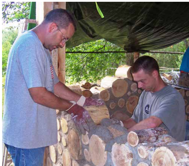
3.6. These students have created two adjacent cradles. After installing insulation, they will find log-ends to fit.
