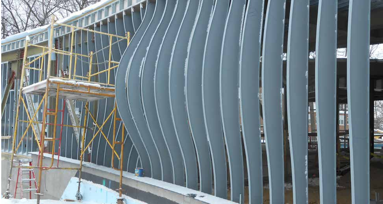
16.12. Specially fabricated metal studs shaped the “warped” wall. Credit: Studio Gang Architects.
