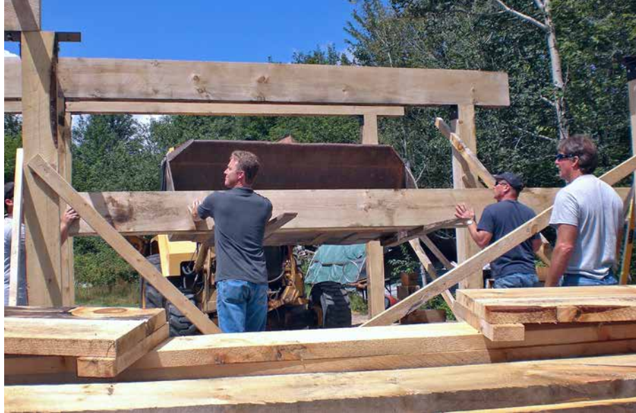
19.3. A very heavy timber frame was designed to support the living roof. Credit: Bruce Kilgore.
