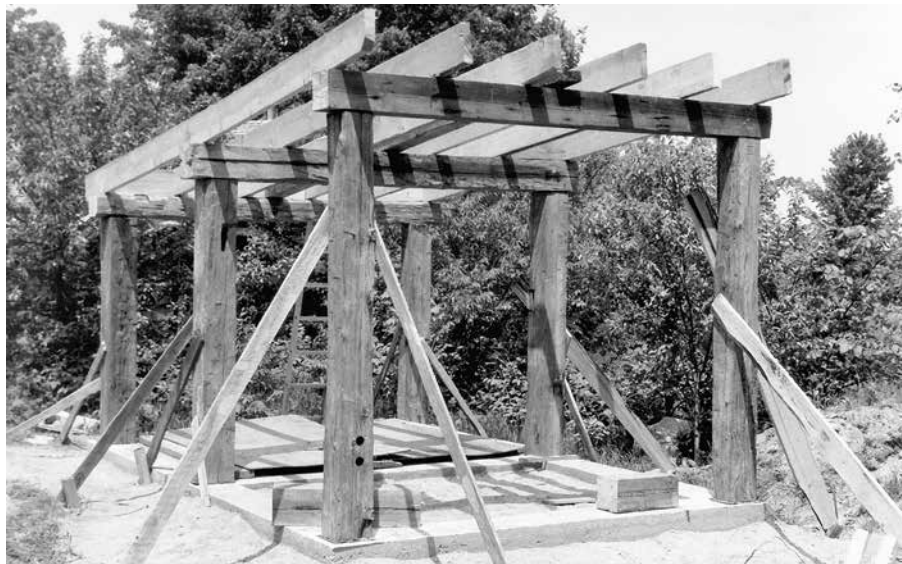
23.2. The six posts are plumbed, then braced to stakes with scrap lumber.
