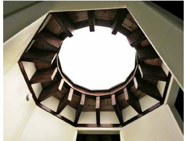
20.8. Sixteen of the 32 heavy Douglas fir rafters are exposed in the center of the building, and support a large round skylight. Credit: Ben Oliveros.
