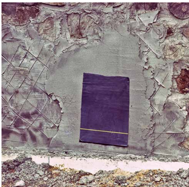
4.1. We tested our intended waterproofing technique on the hardwood wall before tearing it down.
