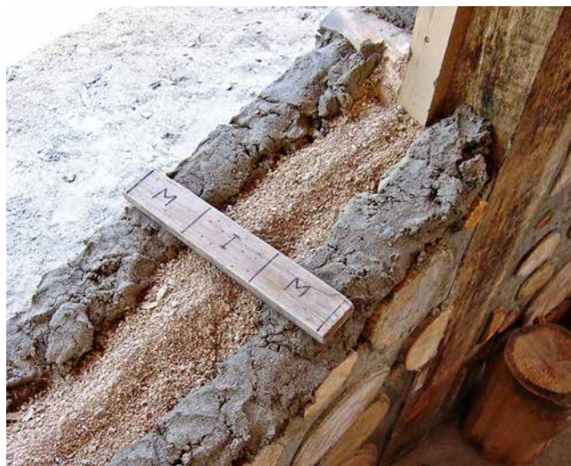
3.5. The MIM stick is used as a guide for new builders to gauge their mortar width.
