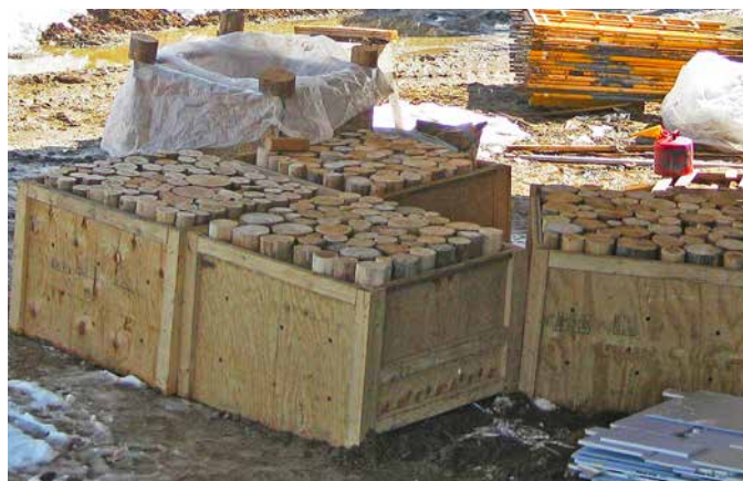
16.7. Logs pre-sorted with random size mix into bins at the job site, ready to be used. Credit: Studio Gang Architects.
