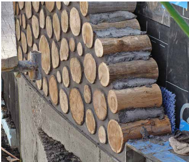
16.8. Typical exterior wood masonry walls are 11 inches thick, with a solid mortar joint. The other layers that make up the wall assembly are described in the text. Credit: Studio Gang Architects.
