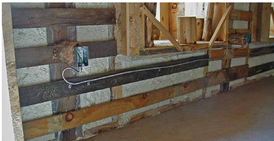
19.5. View from inside showing the outer wall built up to the horizontal wooden lath. Credit: Bruce Kilgore.
