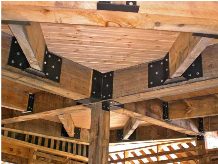
19.4. I spent a winter fabricating the metal hangers we would use to connect our timber frame. Credit: Bruce Kilgore.
