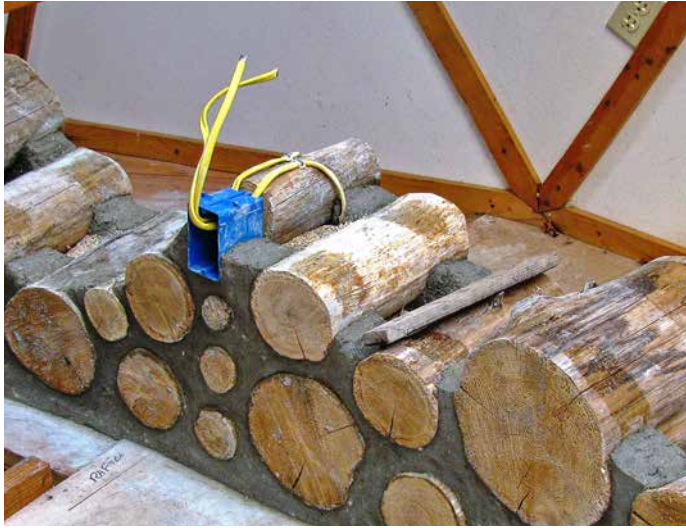
9.7. The wall is built up to and around the electrical box. Notice that plenty of cable is left sticking out of the box to make the connections to the electrical equipment easy for the installer.
