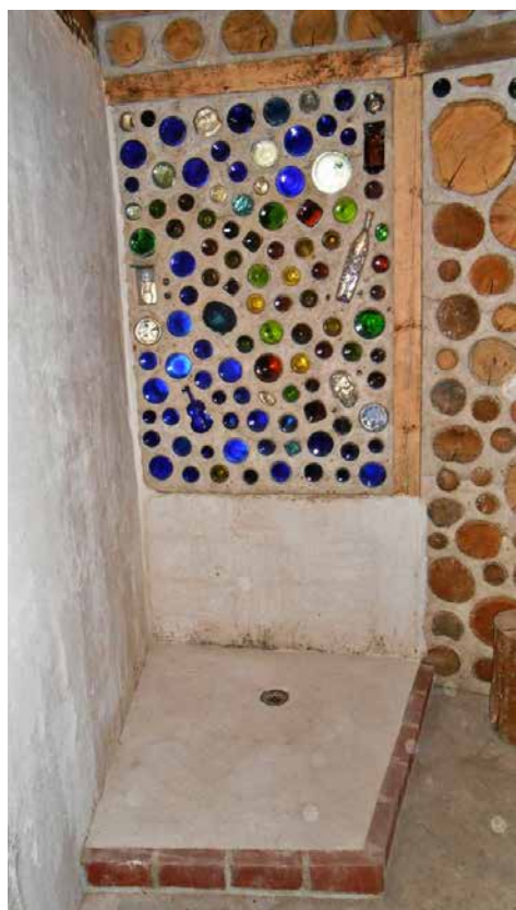
8.9. Shower Island, one of the last walls to be completed, was pointed to a nearly glossy finish.
