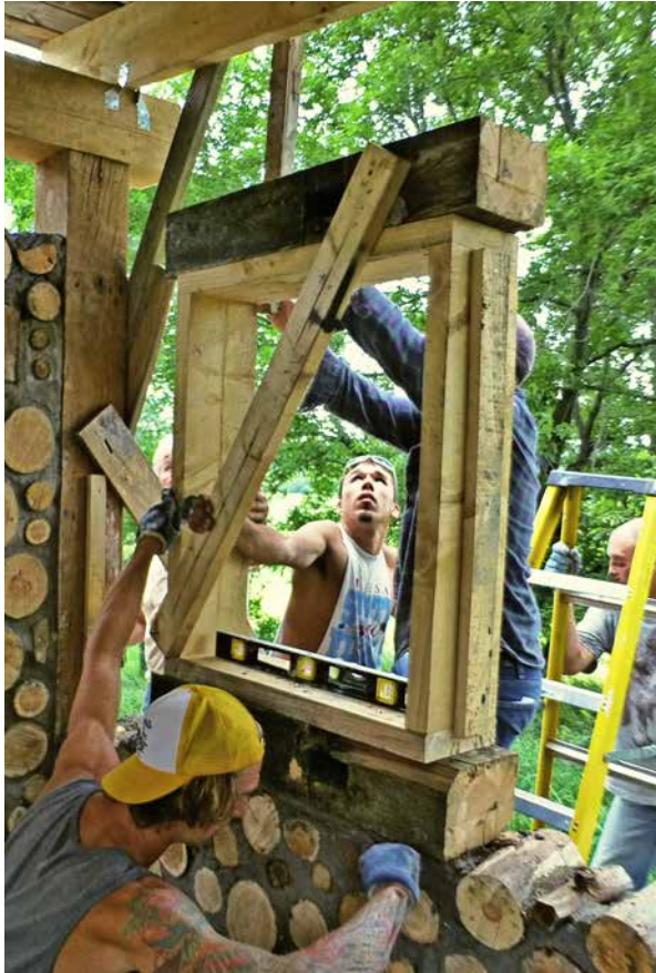
3.8. This window buck is made of full-size 2-by-8 inch lumber. The heavy 6-by-8 inch sill and lintel were an optional design feature which the owner requested. The entire unit was leveled and plumbed, then vertical braces held it plumb against one of the rafters. Note the diagonal brace to hold the buck square, and the key piece on the side.
