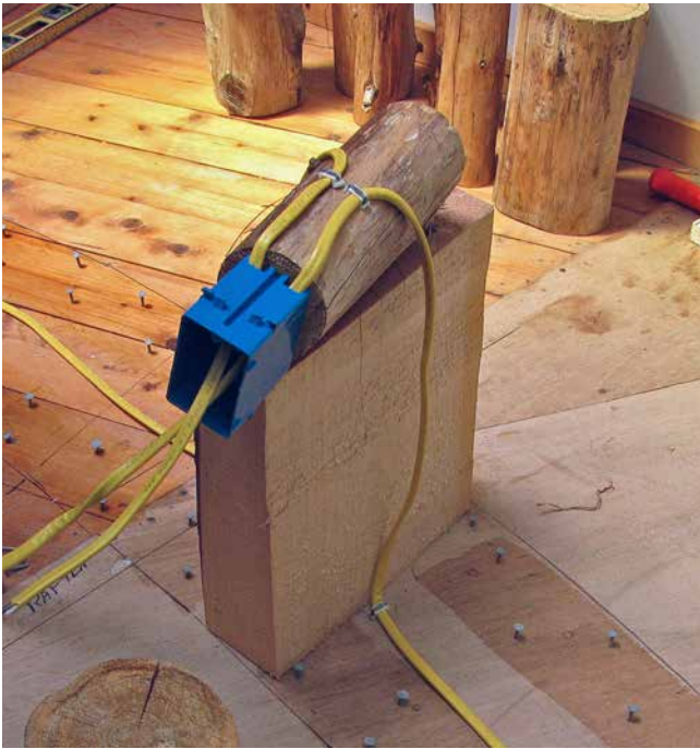
9.5. Before laying the first course, we installed electrical boxes to the ends of 4-inch diameter by 8-inch long log-ends, and held them off the floor with 16-inch tall pieces of wood, so that the duplex receptacles (DRs) would be at the conventional height off the floor. These log-ends were later built into the cordwood wall. The Romex follows the insulated space between the inner and outer mortar joints. The little roofing nails sticking out of the plywood help lock the mortar to the floor. The wood is also treated with sealer and bonding agent prior to laying down the 4-inch-wide mortar joint.
