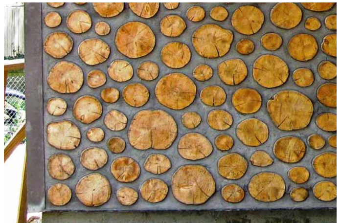
16.14. The masons maintained a good balance of log sizes throughout, while keeping a constant minimum width of mortar joint. Credit: Studio Gang Architects.
