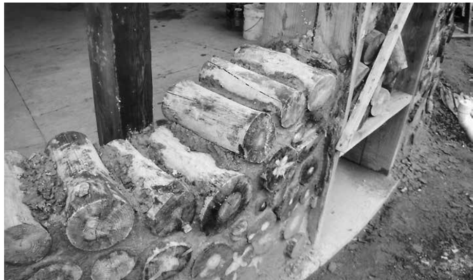
12.1. Our 16-inch-thick walls have a solid papercrete mortar joint. The log-ends are pine. Credit: Jim Juczak.
