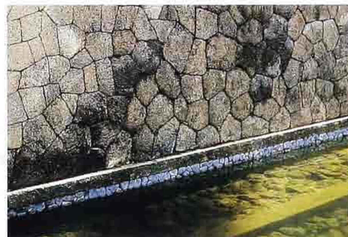
WA-63 Pool wall in hammered-finish sandstone with mosaic bond and water-line courses of roughly squared stone and beach pebbles
