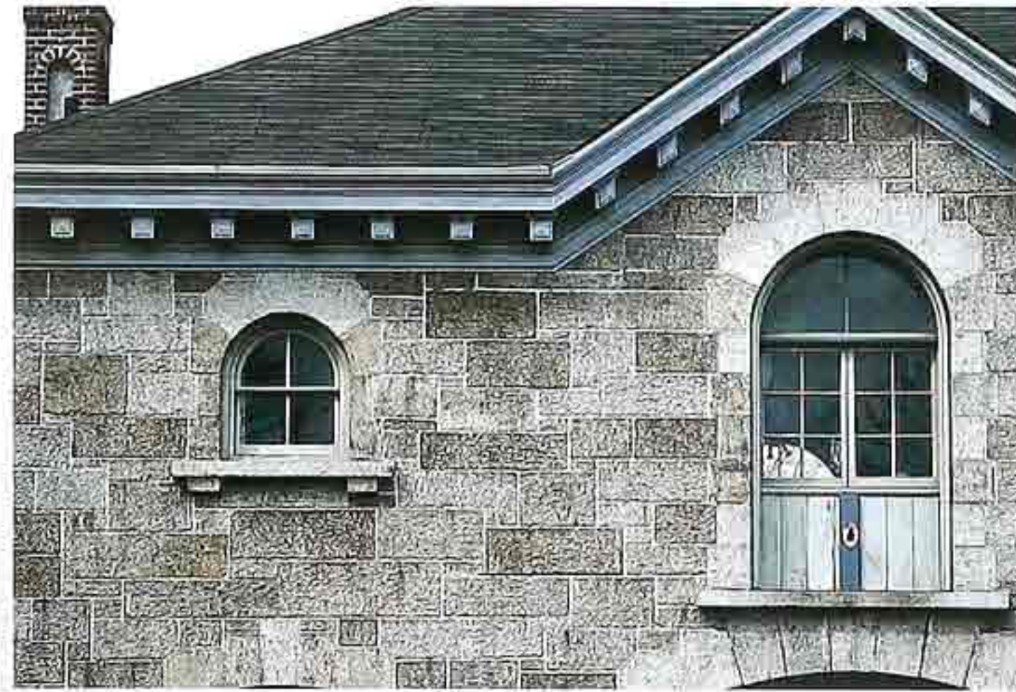
WA-123 Gable-end wall in random ashlar; block modillion cornice; quoins around arched windows; corbelled window sill (left)
