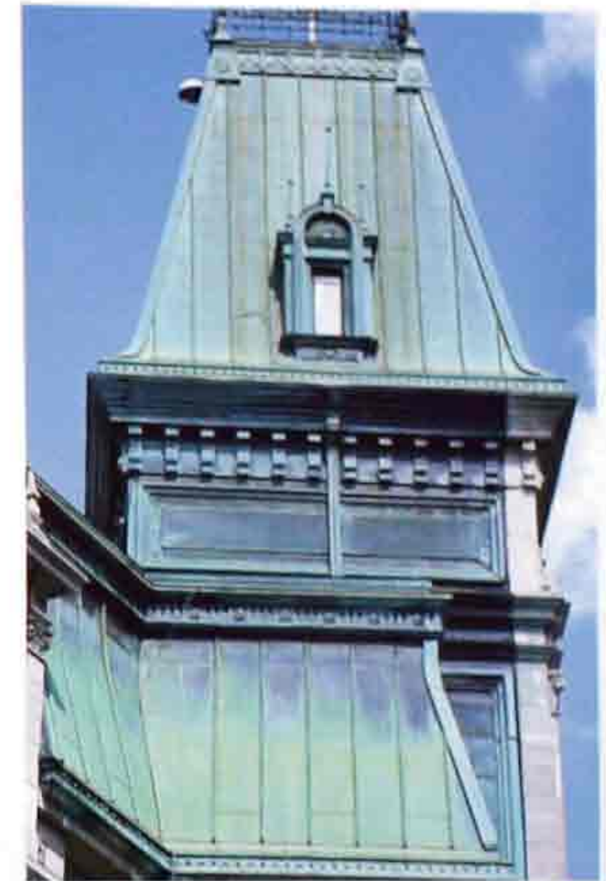
CR-35 Copper with standing seams, hipped roof with cresting and arched roof dormer; copper cladding and molding on walls
