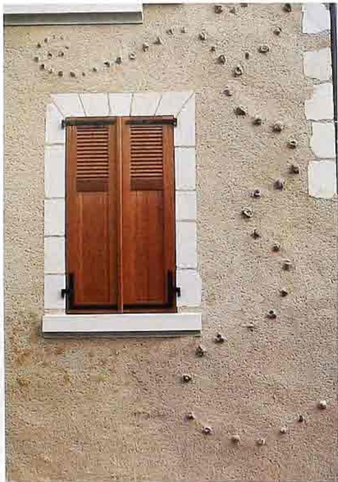
WA-230 Stucco with dimension-stone window and corner quoins and natural stone insets in serpentine design; louvered shutters, house
