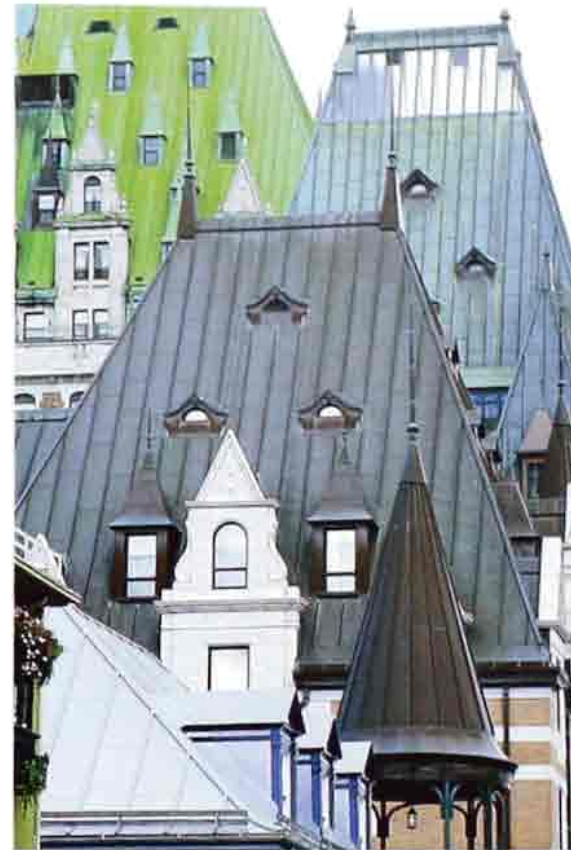
CR-34 Copper (top) and other varieties of sheet metal with batten and standing seams on hipped and conical roofs, 19th-c. chateau-style mixed-use buildings
