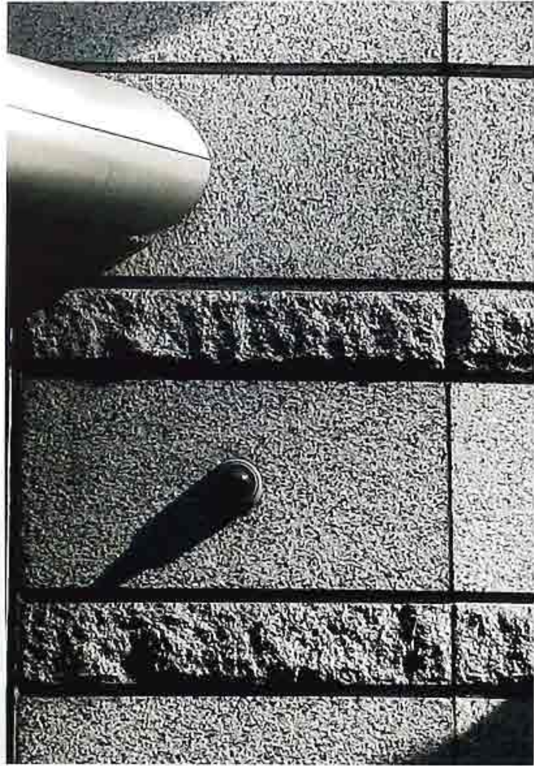
WA-82 Detail of doorway reveal in stack bond with alternating courses of rock-face and sawn granite; mitered corner joints
