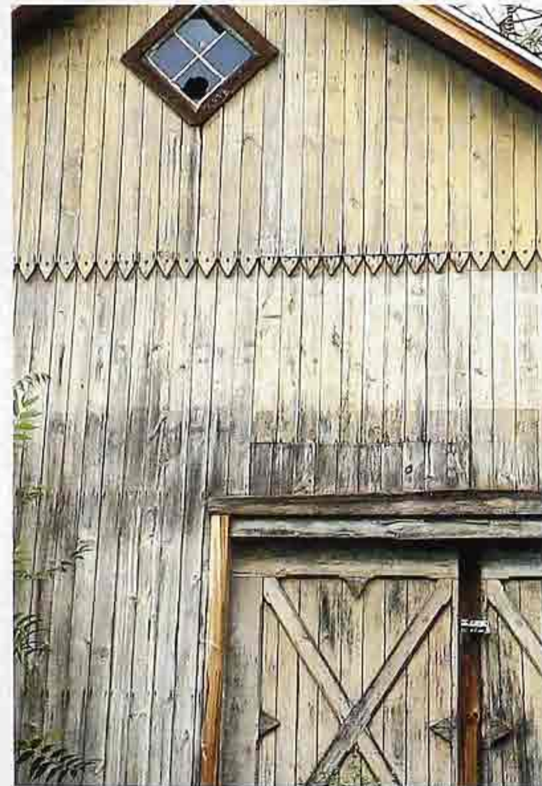
WA-30 Weathered painted flush vertical board cladding on barn gable end with diamond-shaped window and vertical scallop-edged siding
