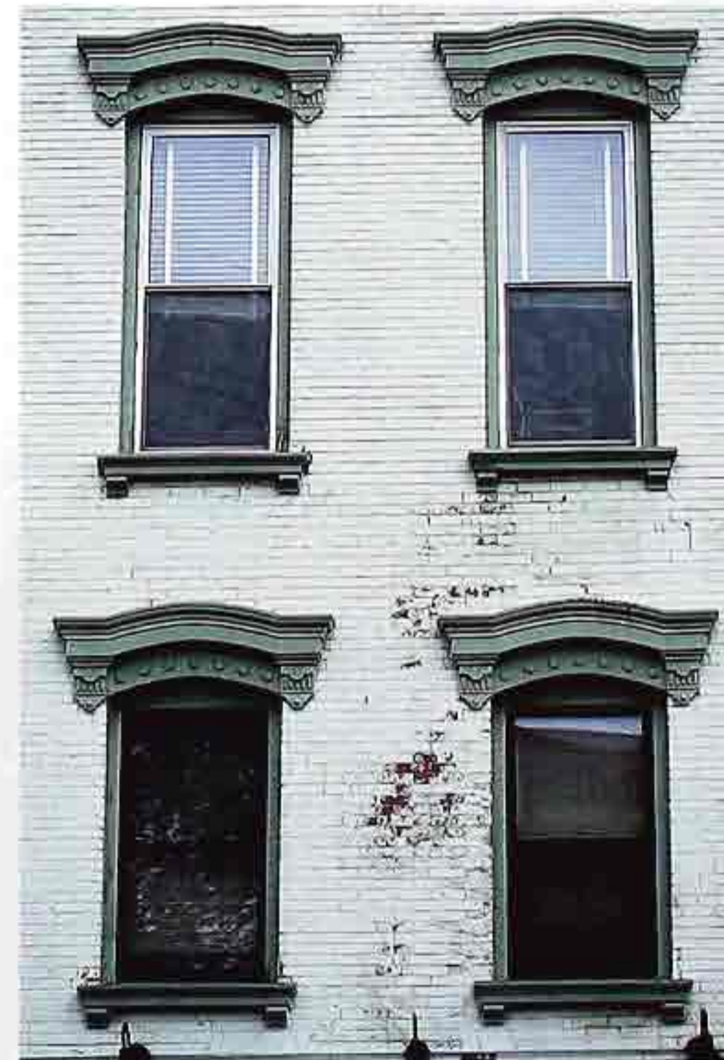
WI-109 Flat trim echoing arch profiles of window openings, 19th-c. American mixed-use building
