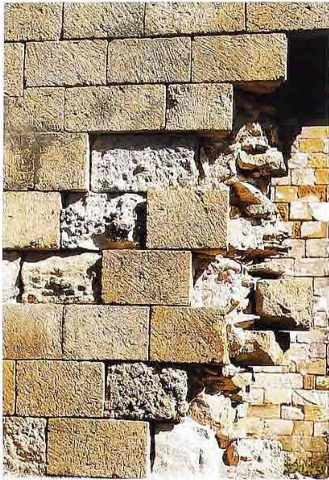
WA-72 Coursed ashlar sandstone wall in ruins revealing structural rubble wall
