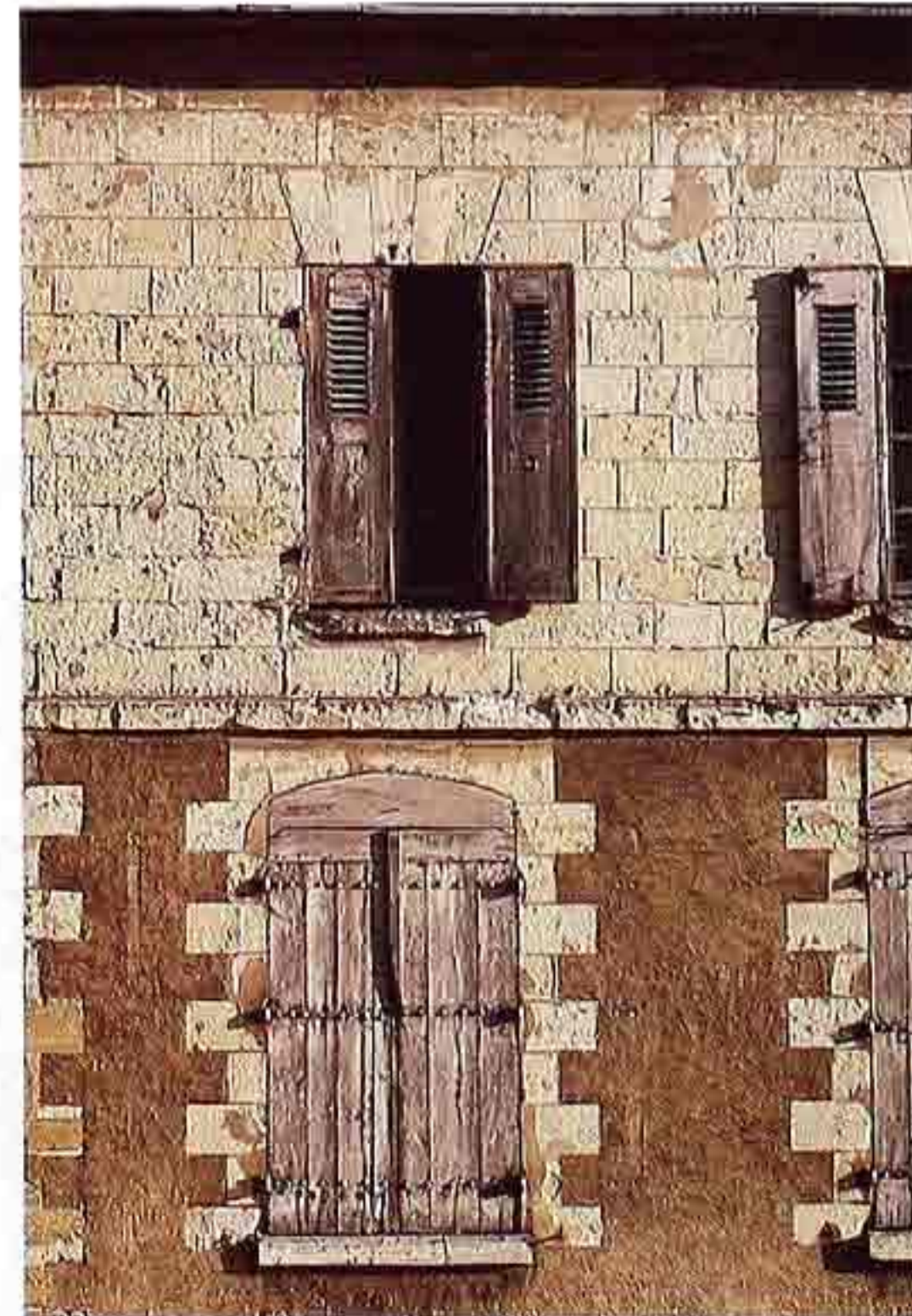
WI-197 Weathered painted wood paneled shutters
