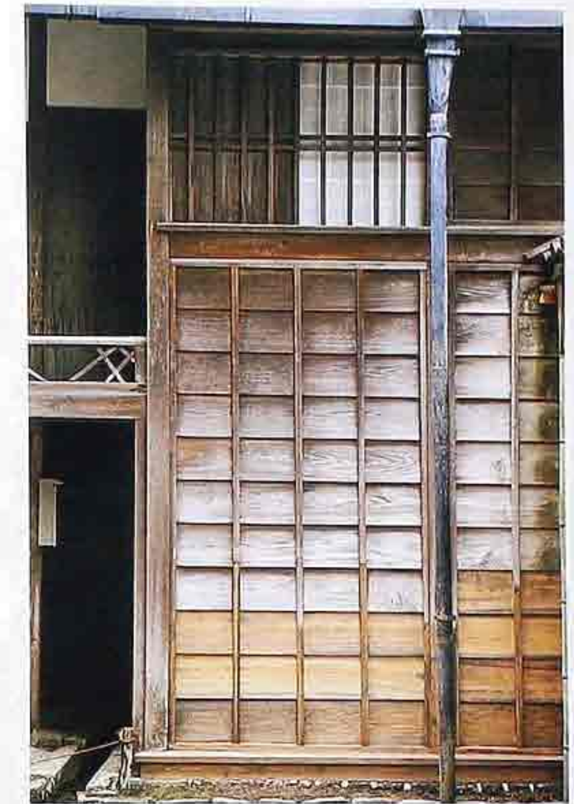
WA-41 Timber frame with infill of plain-sawn cedar planks; gutter with rainwater head
