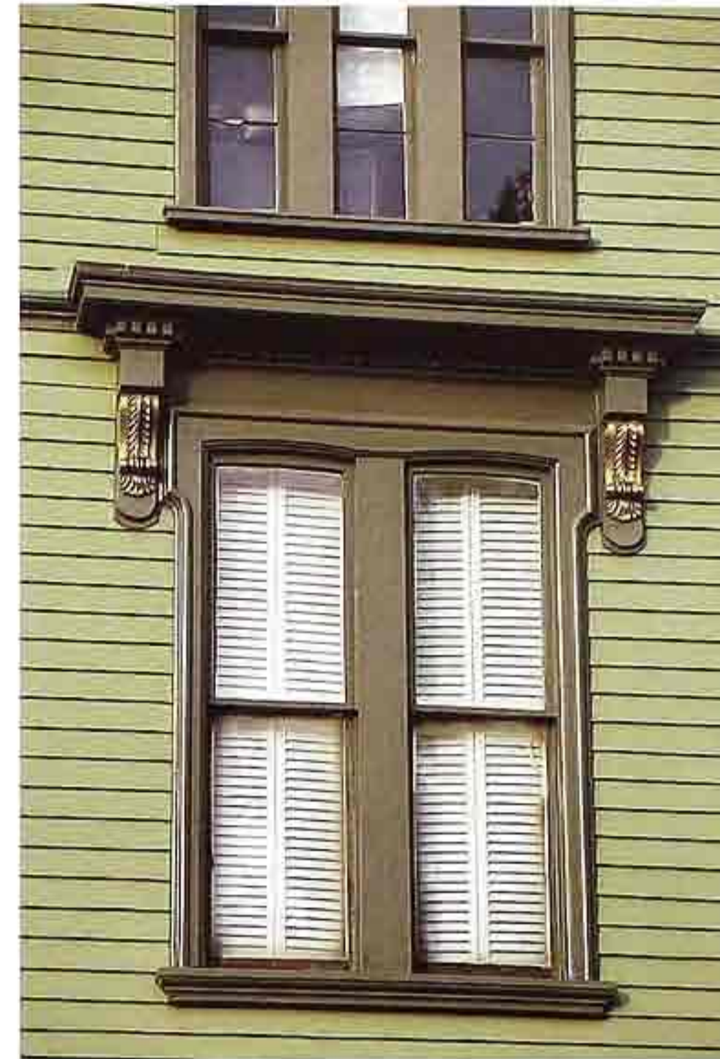
WI-107 Flat wood casing with crossettes around one-over-one double-hung windows; hood supported by brackets, American clapboard house
