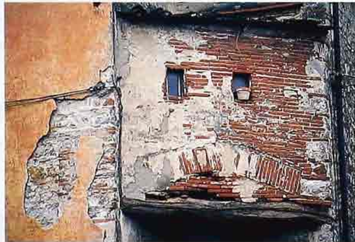
WA-256 Weathered colored stucco revealing timber lintel, scratch coat and structural stone, and Roman brick
