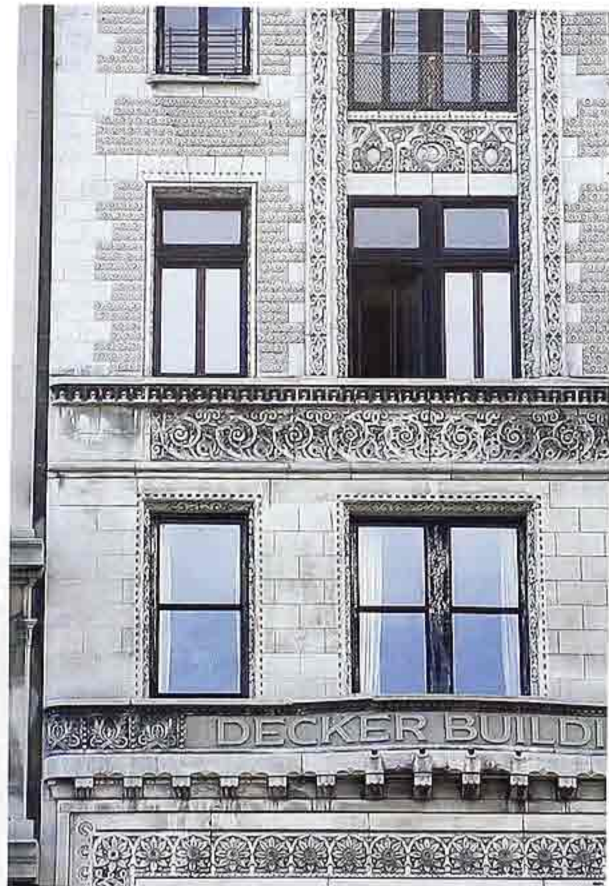
FA-112 Molded cornices and window surrounds with running ornament on multistory masonry facade
