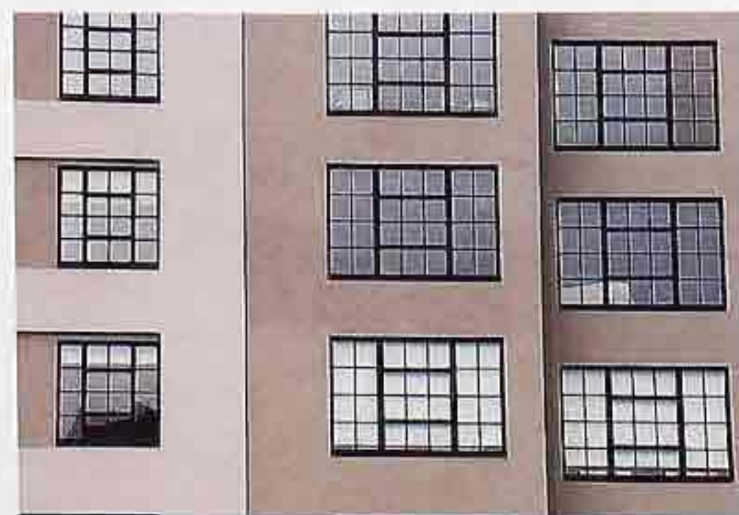
WI-42 Single-hung or awning windows with various muntin patterns, modern apartment house
