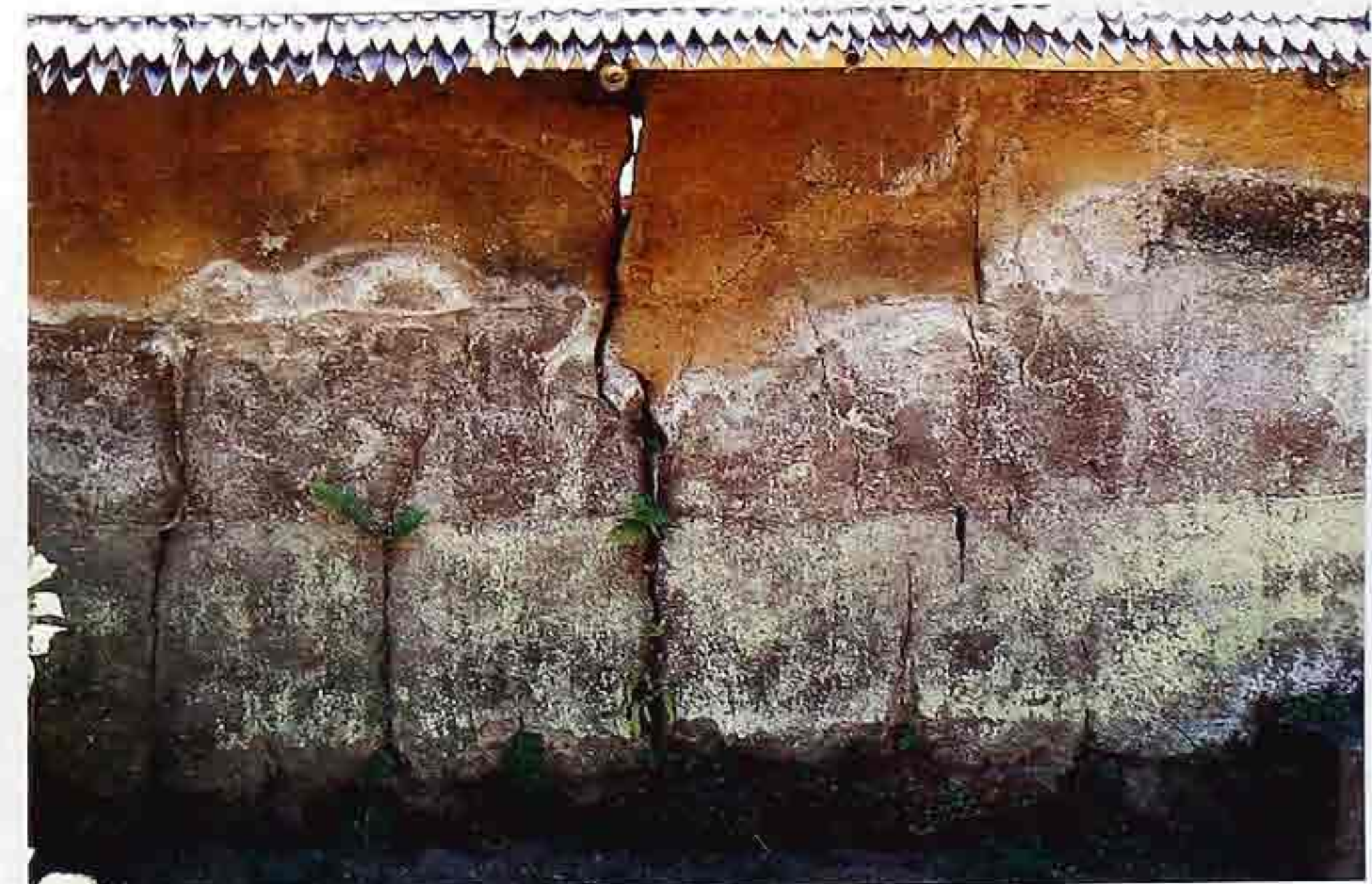
WA-253 Weathered tinted mud stucco revealing rammed mud wall
