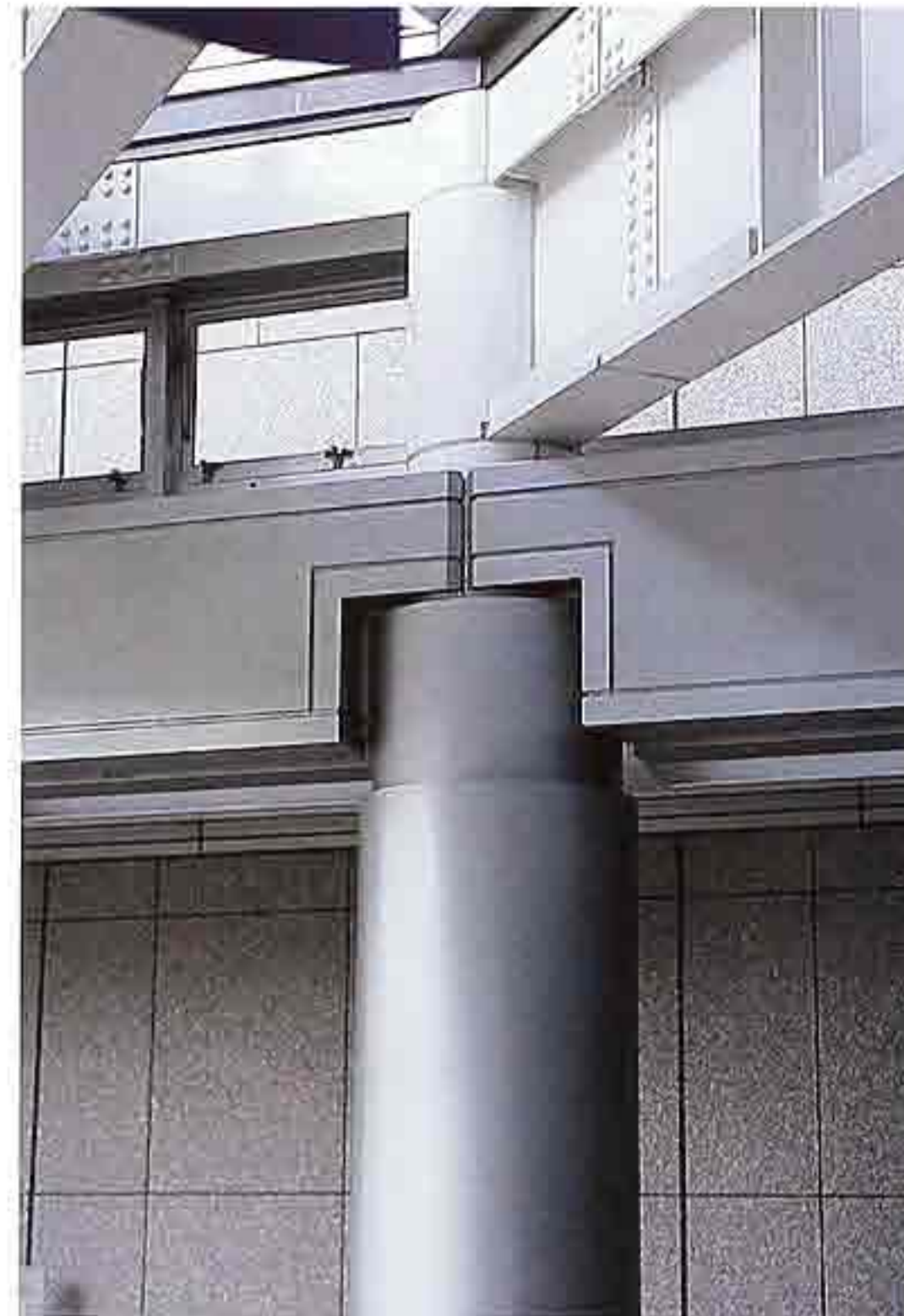
CP-123 Detail of steel frame with metal-clad column and beam beneath exposed riveted plate girders, modern commercial building
