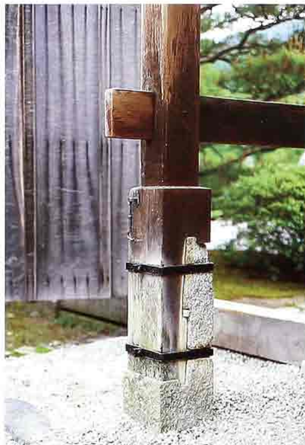
CP-106 Timber post connected to stone plinth with rabeted scarf joint and metal hoops. Horizontal brace joined by mortise-and-through-tenon joint.
