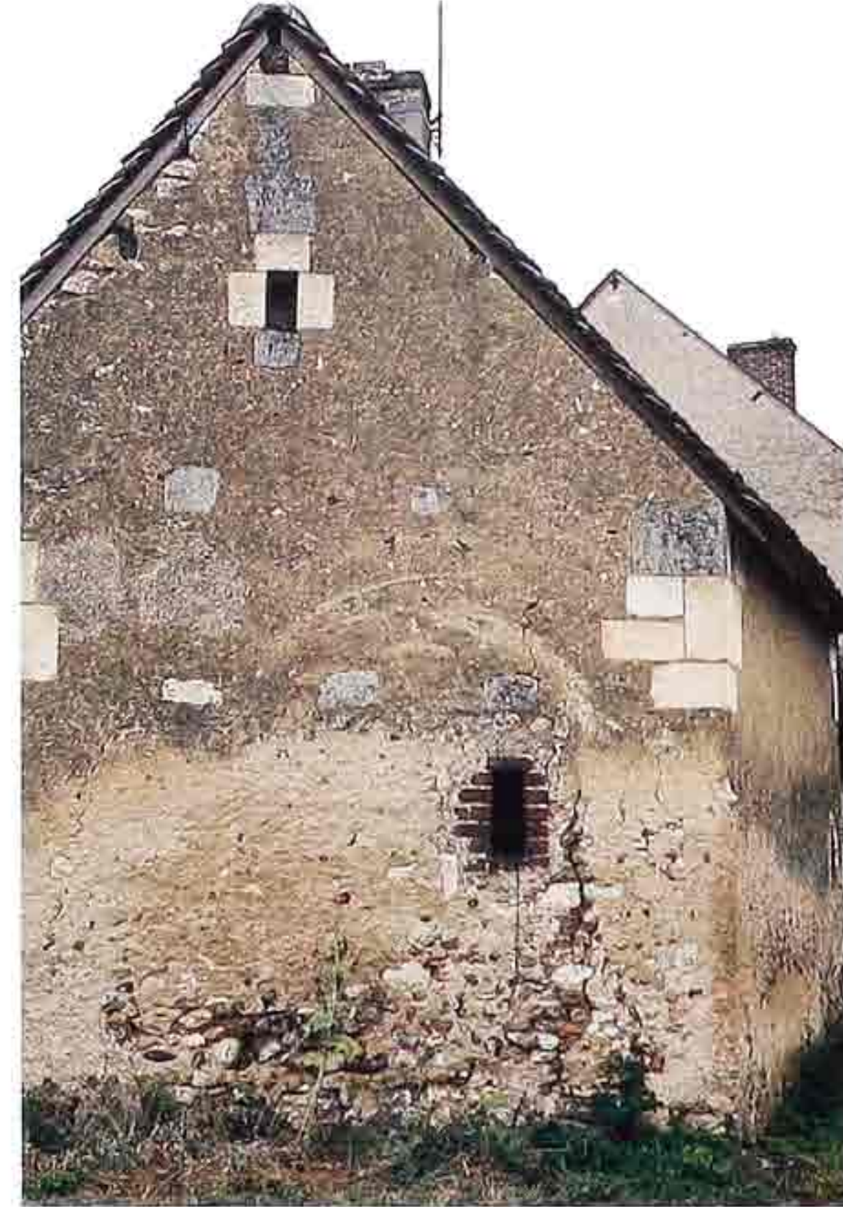
WA-249 Large-aggregate stucco with cobbles and quins on weathered gable-end wall, farm building
