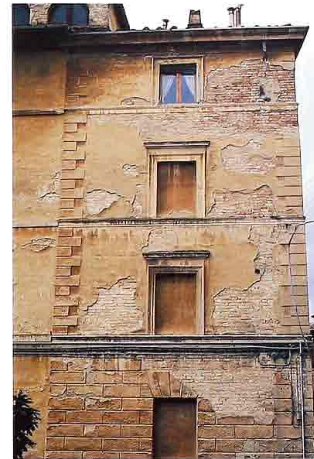
WA-260 Weathered stucco exposing structural brick and stone. Original plasterwork included faux-stone quoins and blocks in running bond
