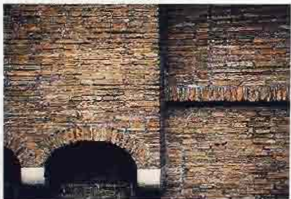
WA-155 Roman brick with projecting soldier course and elliptical arch with stone corbels, ancient Roman wall
