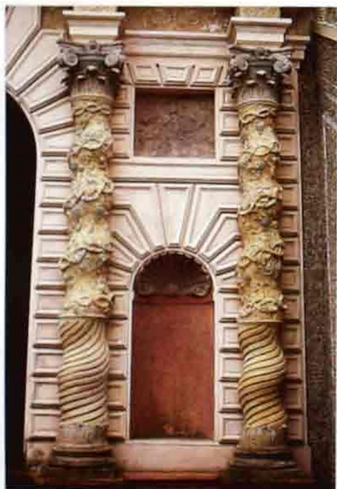
CP-67 Stone entryway with partially fluted Salomonic columns, garland ornament, and Composite capitals
