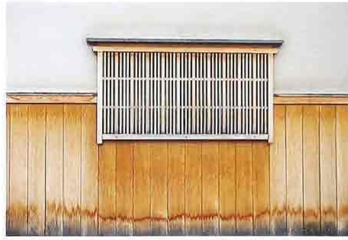
WA-274 Stucco and wood-planked infill; timber-frame construction; traditional Japanese wood lattice window
