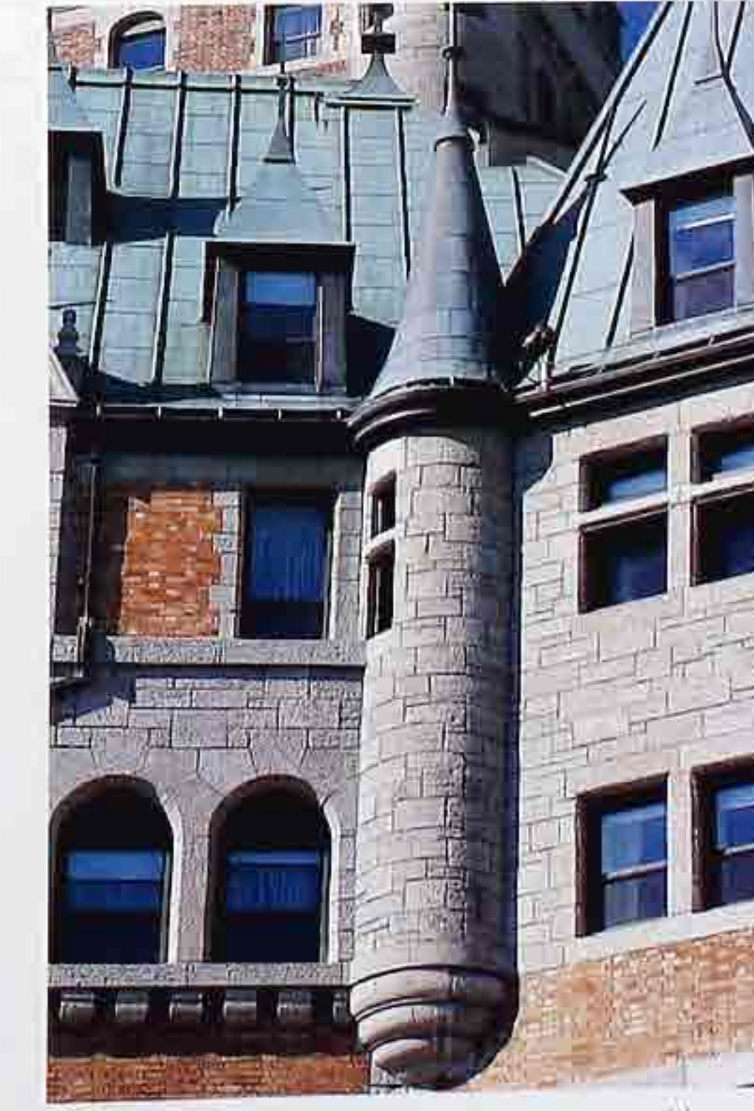
WA-289 Coursed ashlar on inside-corner turret with corbelled jetty and adjacent upper story; remaining walls of brick
