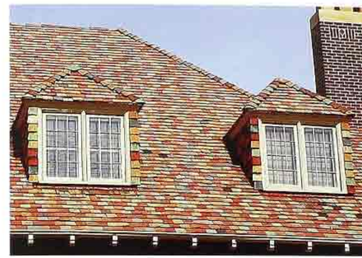
CR-49 Flat multicolored shingle tiles with hipped roof dormers, 20th-c. American house
