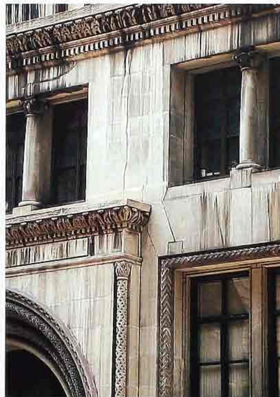
WA-115 Weathered limestone in coursed ashlar with dentil and modillion cornice; carved ornament on columns and window frames
