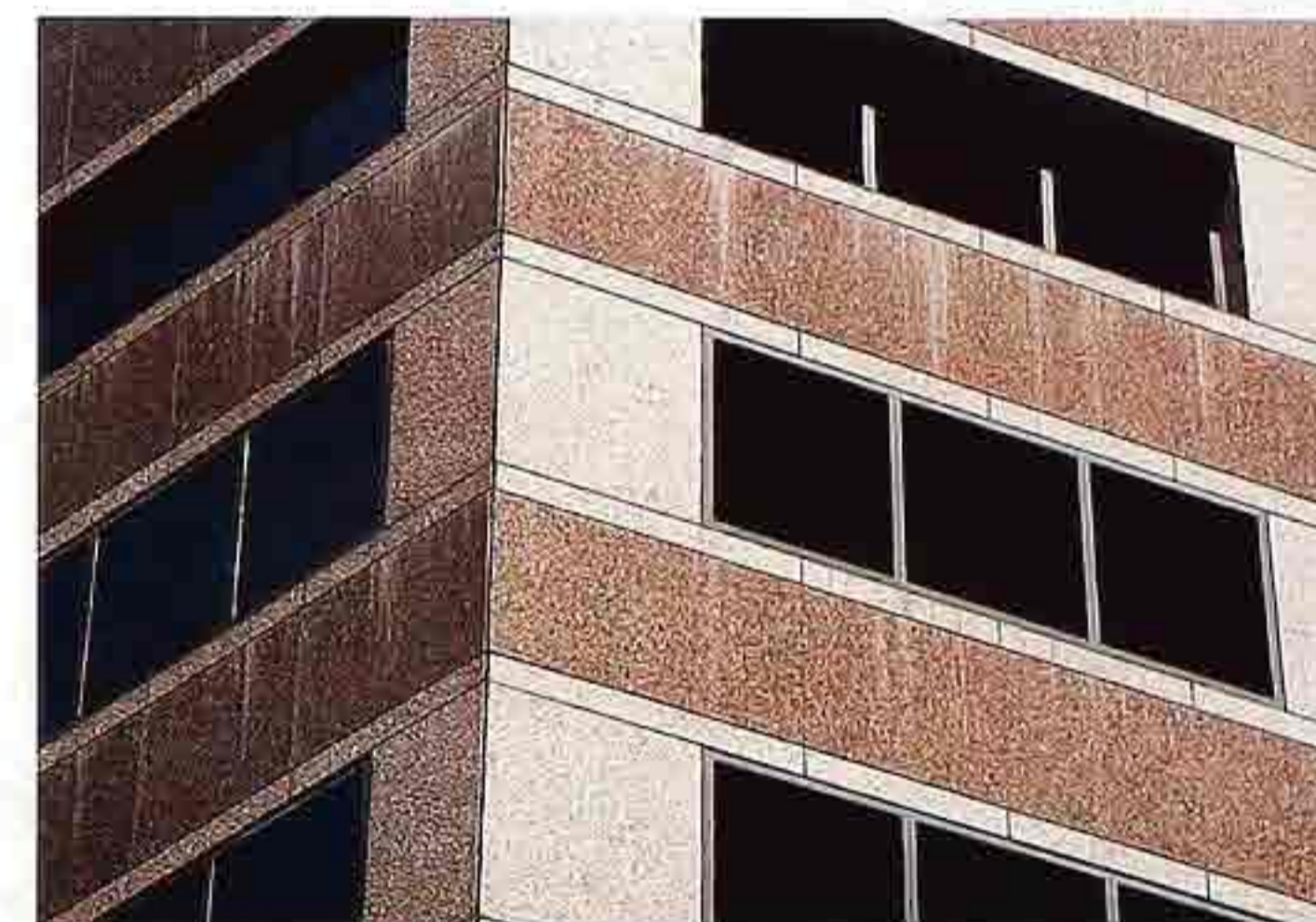
WA-136 Banded polished-granite-veer spandrels alternating with honed granite and ribbon windows, modern commercial building
