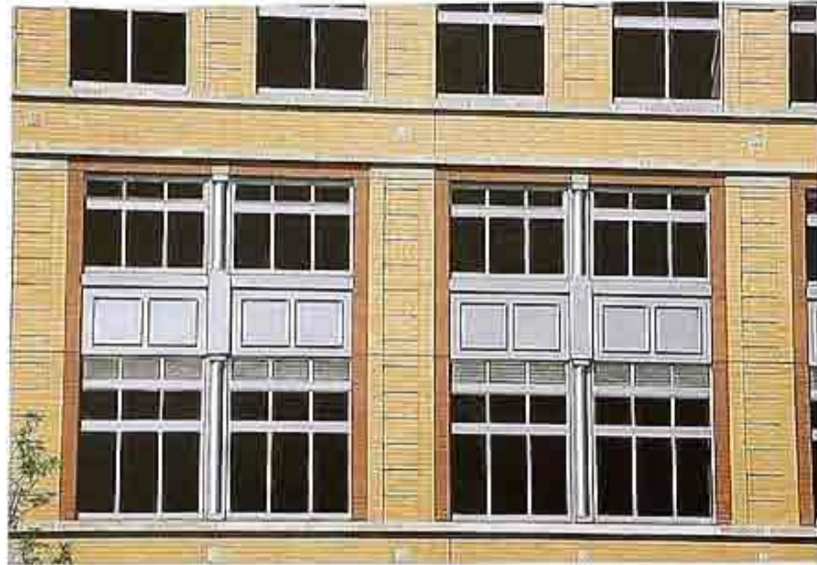
WI-158 Repetitive fenestration of three-mullion windows with raised panel spandrels, modern commercial building
