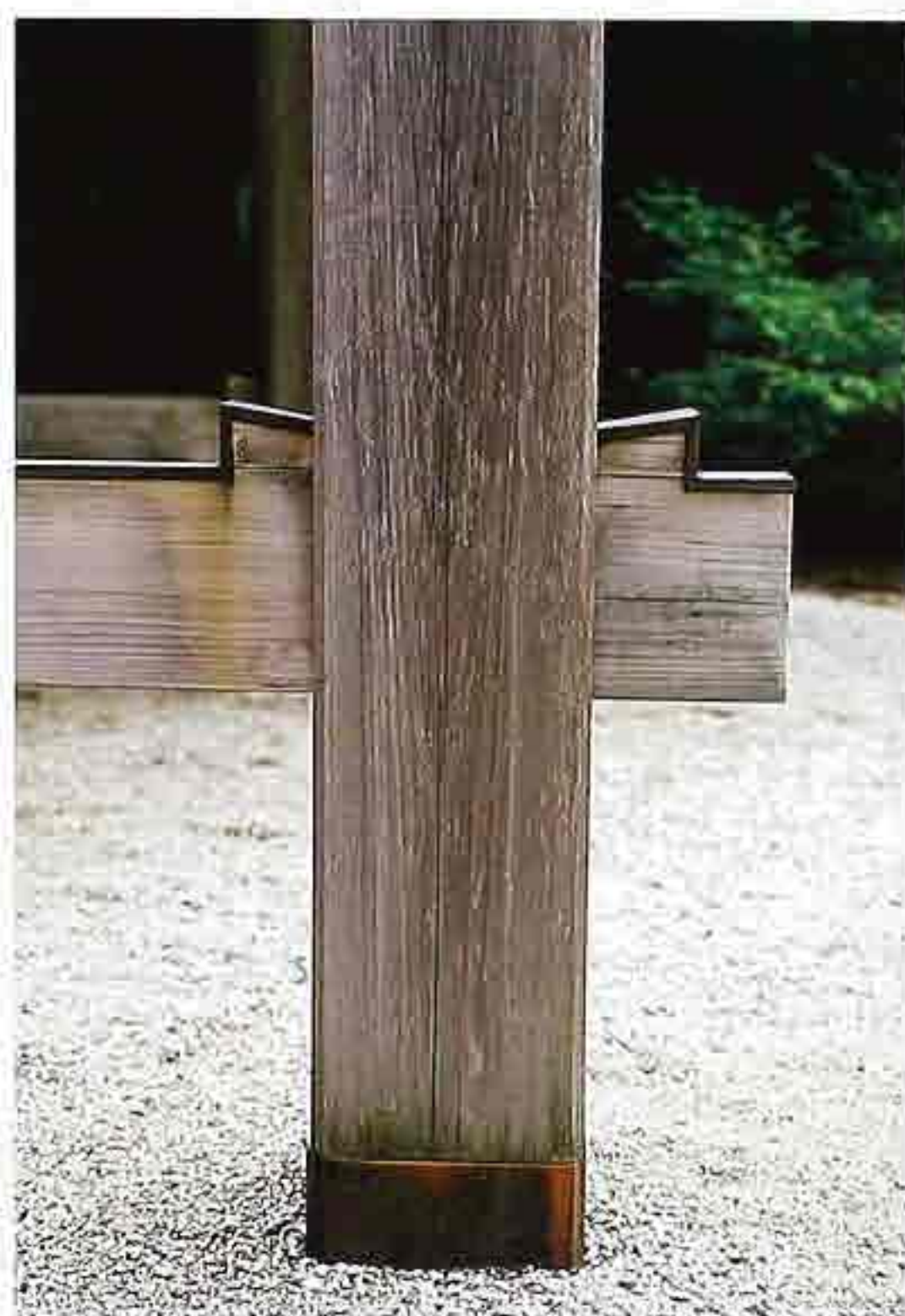
CP-108 Timber post with a horizontal brace attached by a double-wedged through-tenon joint with metal striping on the top.
