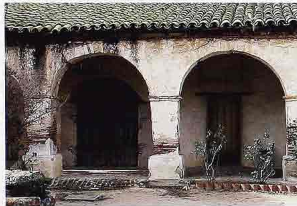
CP-164 Arcade with semicircular arches with molding at springing, stucco over adobe brick, late-18th-c. American Southwestern mission
