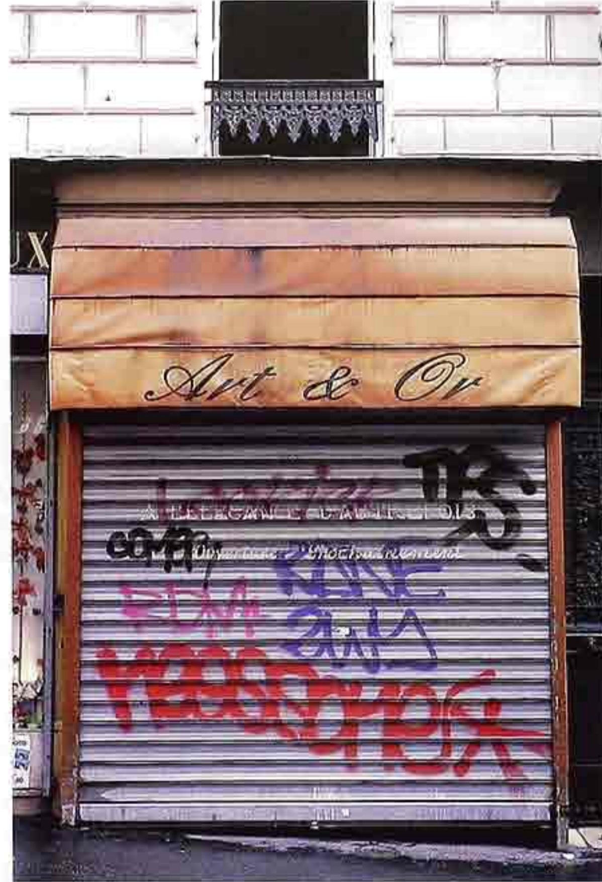
DW-53 Rolling galvanized-metal security door with graffiti
