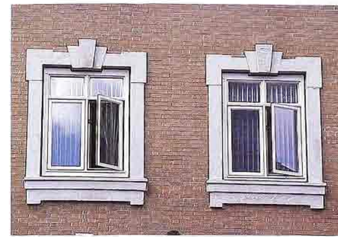
WI-25 Two double-casement windows with divided transom lights, stone window surrounds, 19th-c. apartment house
