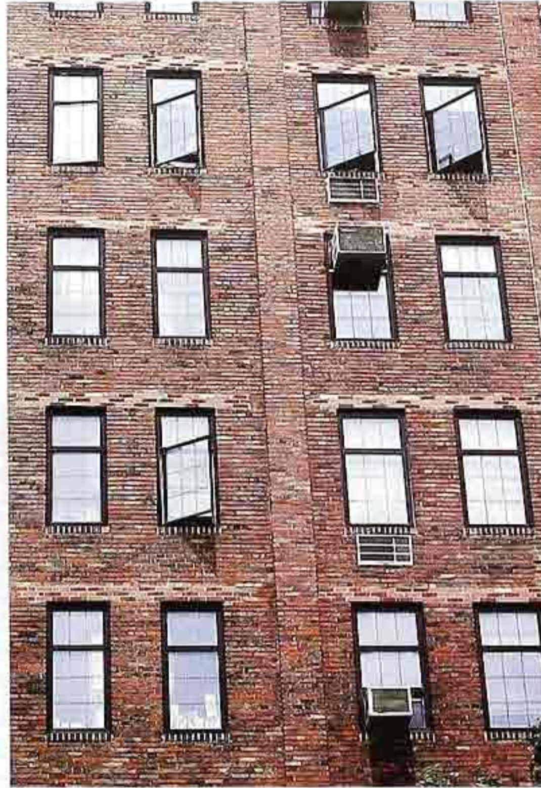
WI-31 Casement windows with internal muntins and fixed light above, modern metal replacement windows in older apartment house
