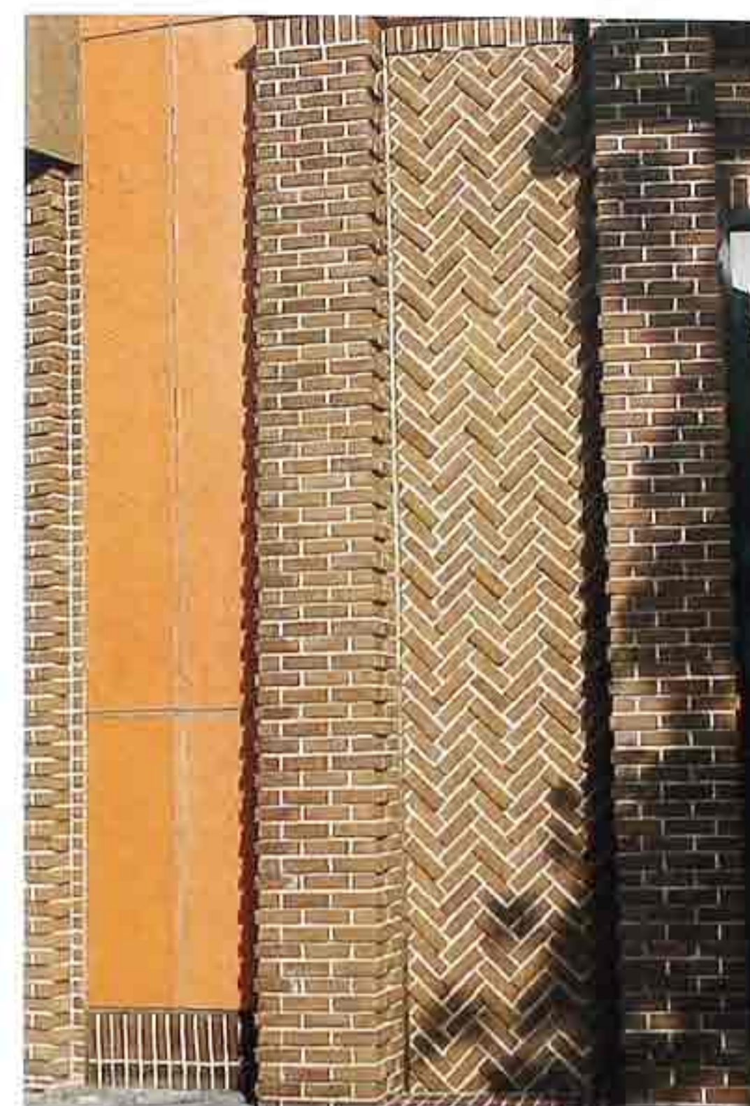
WA-201 Pilasters in running bond with variation of dog's-tooth edge; inset panel of decorative brickwork in herringbone pattern with projecting bricks
