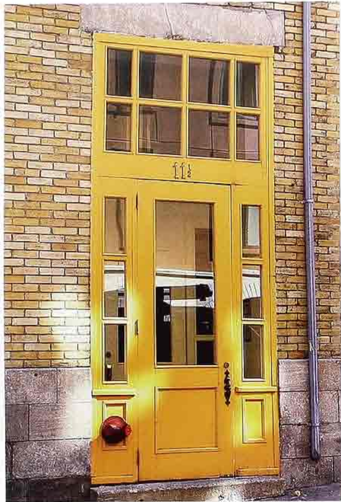
DW-66 Painted wood doorway with eight-light transom panel over three-light side lights and single-light paneled door, commercial building
