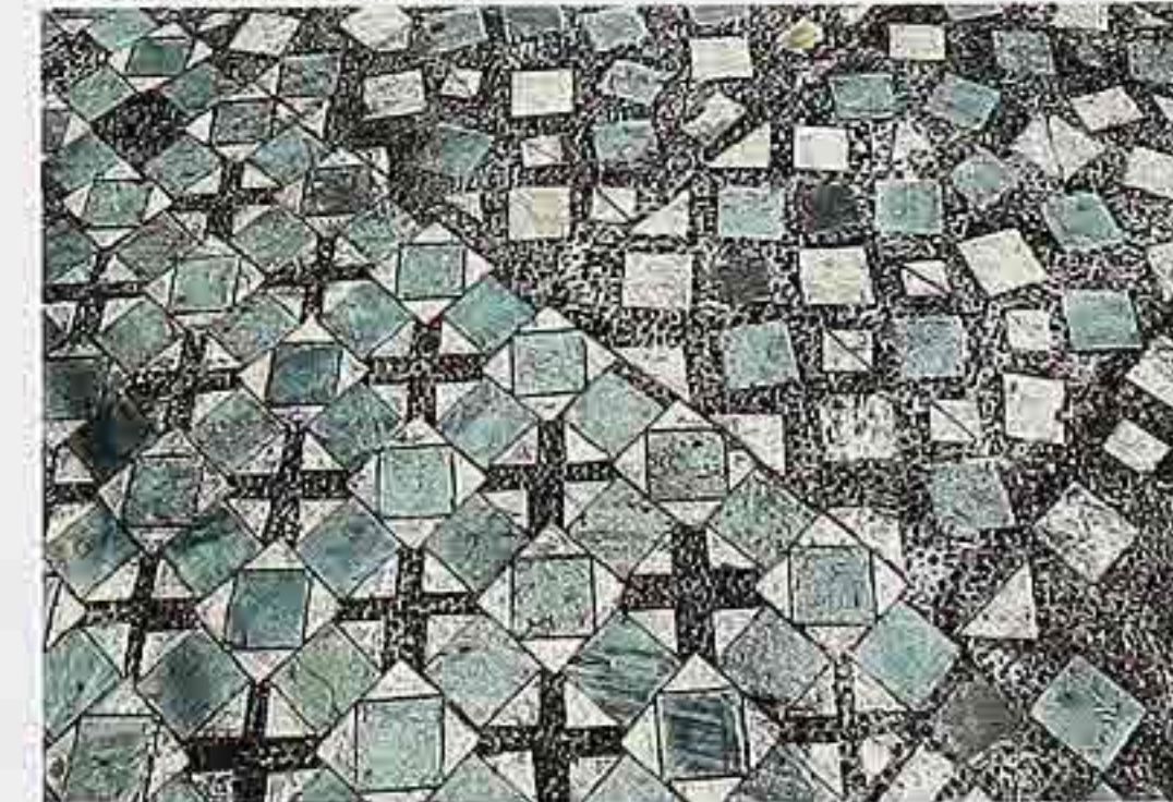
FP-101 Square and triangular ceramic tiles set in exposed-aggregate field in geometric and random patterns, entryway
