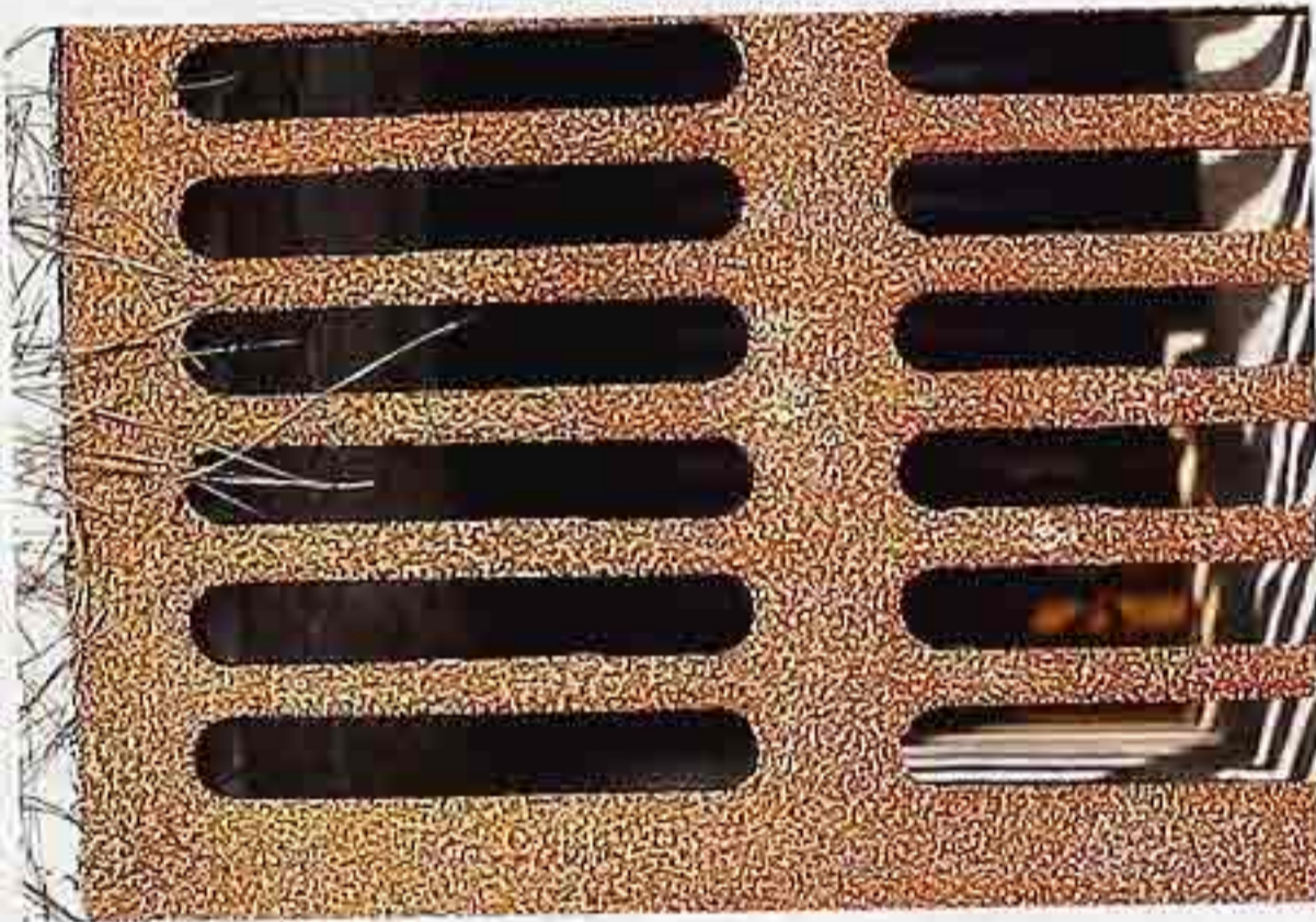
FP-115 Rusting cast-iron drain grate
