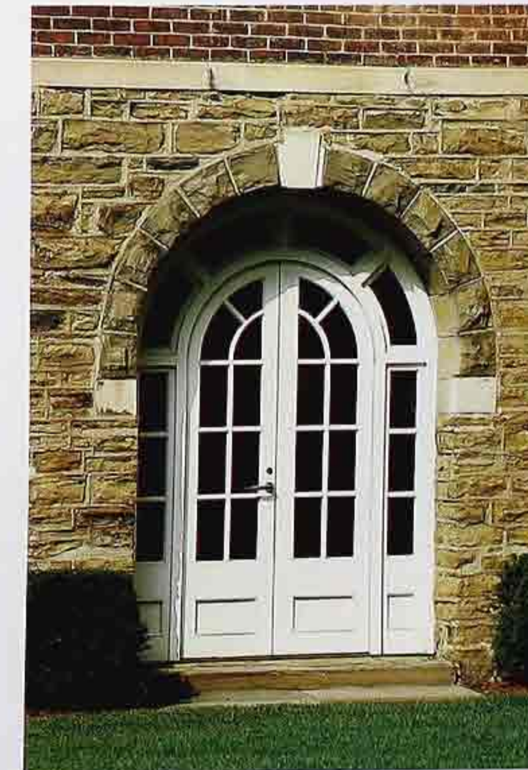
DW-65 Wood double doors and side lights in semicircular doorway; stone arch with keystone and imposts
