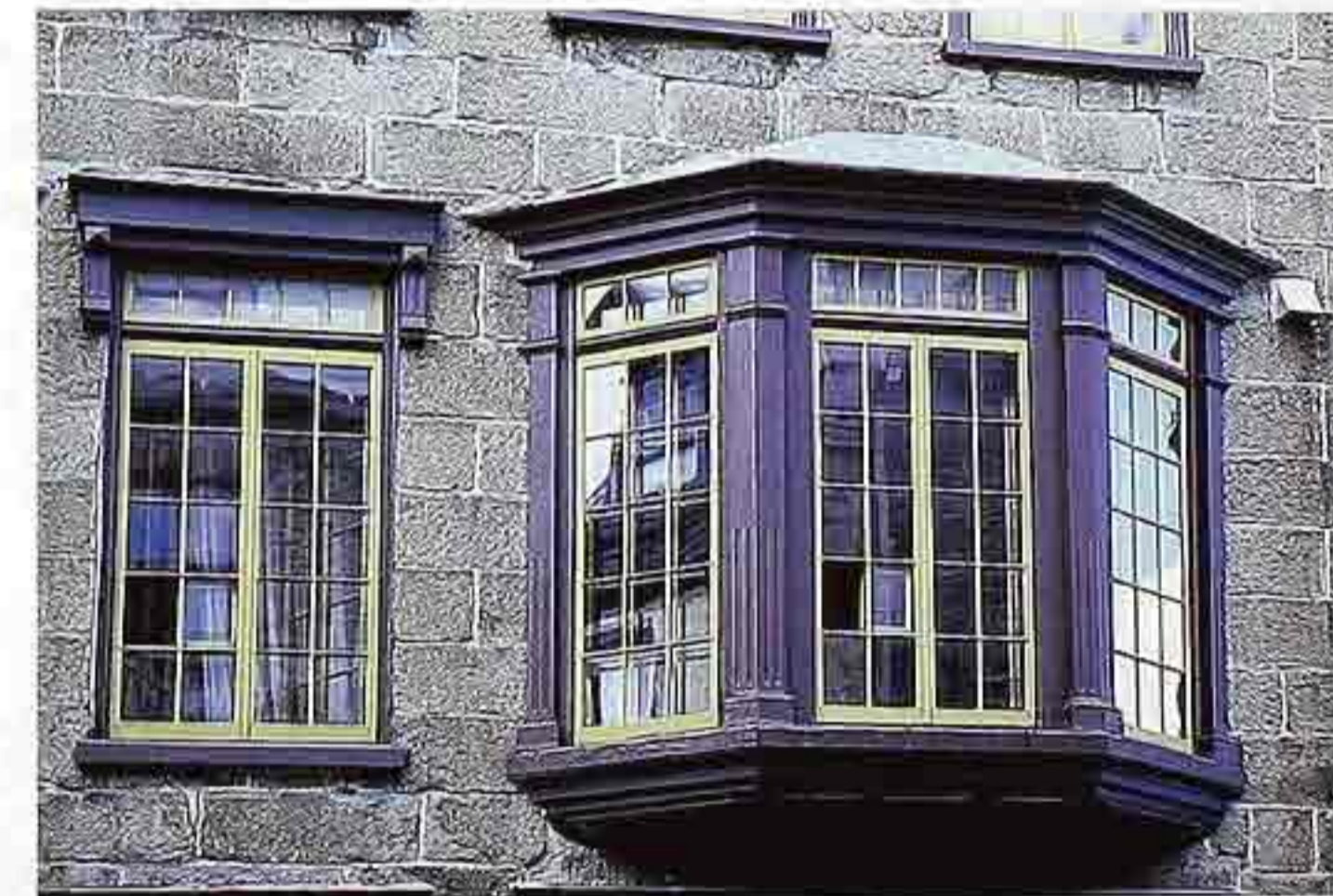
WI-84 Left: double-casement window; right: cant-oriel with fixed side and transom lights and center casement window, 19th-c. mixed-use building
