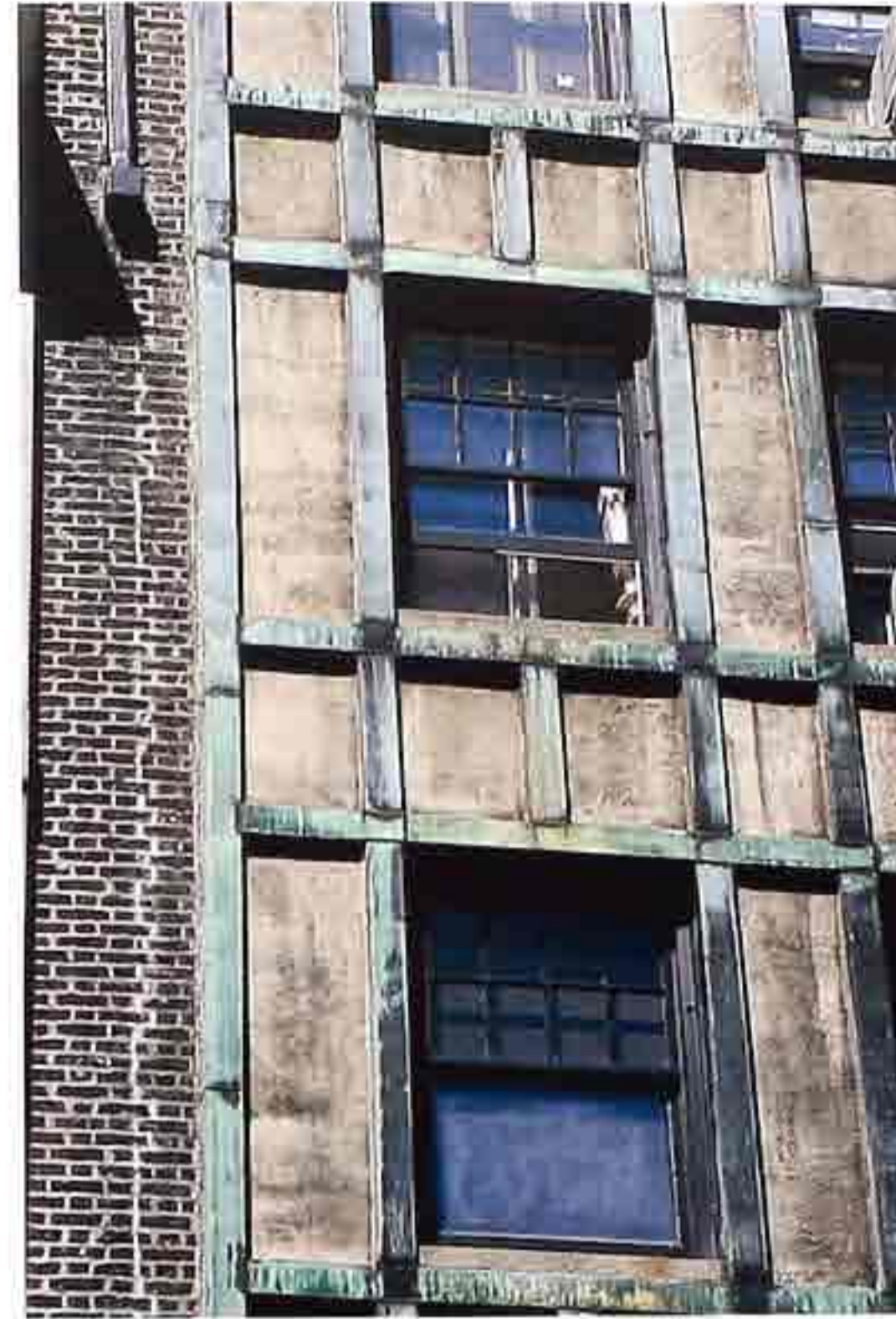
WA-278 Decorative half-timbered facade with concrete infill and copper "timbers," 20th-c. residential building
