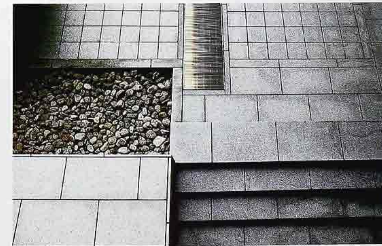
FP-27 Textured dimension paving stone with straight joints (top), and running bond (bottom), metal grates, and river rocks in courtyard of modern commercial building
