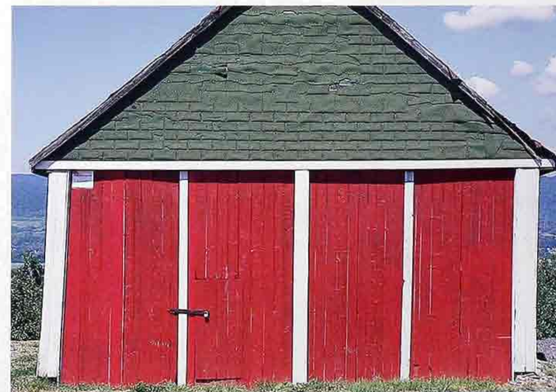
FA-81 Painted garage with shingles on gable end, vertical tongue-and-groove siding and door
