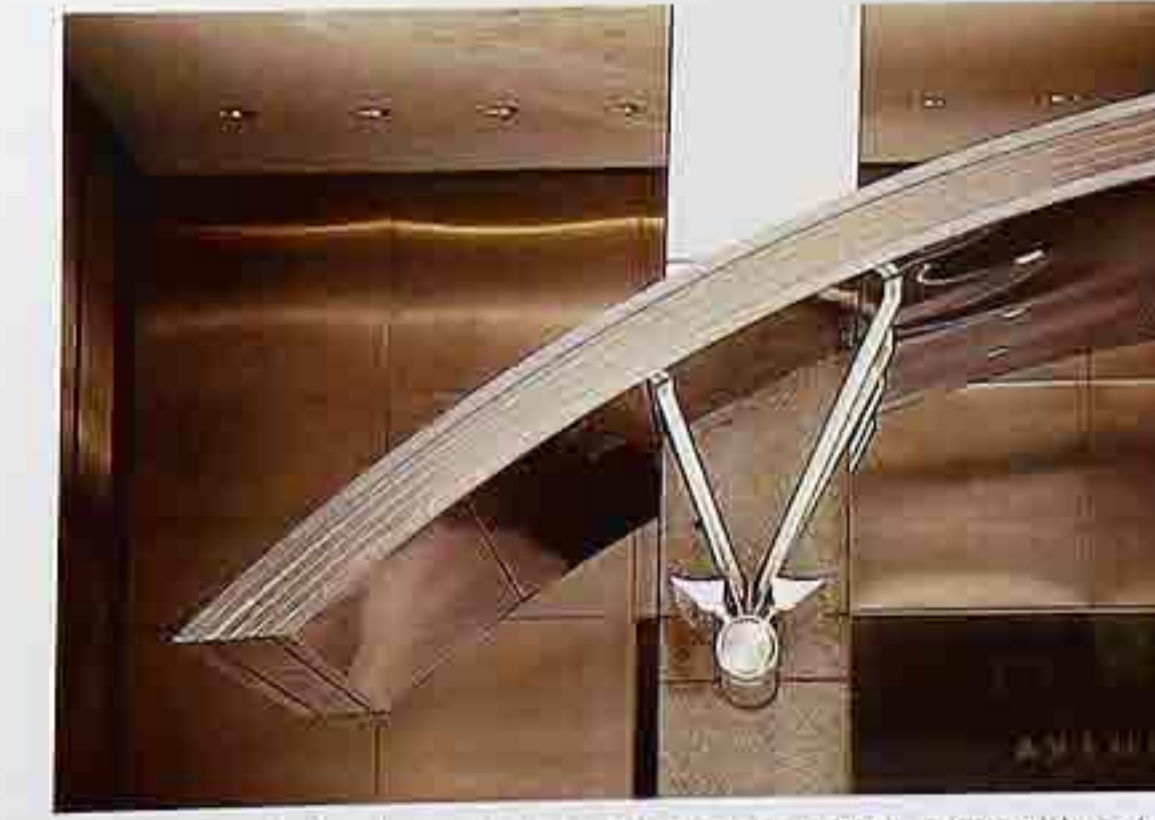
CP-121 Semicircular metal canopy supported by a metal bracket set into a masonry column, modern commercial building
