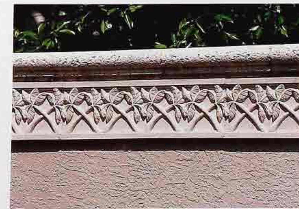
OM-38 Ornamental band with interlocking palm motif below the coping of a garden wall
