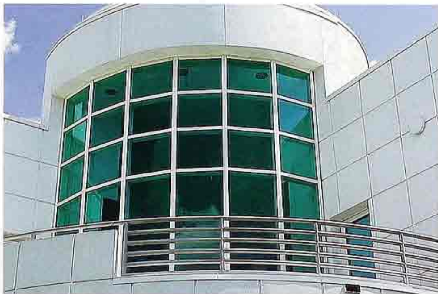
WI-74 Fixed tinted windows in stainless steel frames on curved wall, modern commercial building
