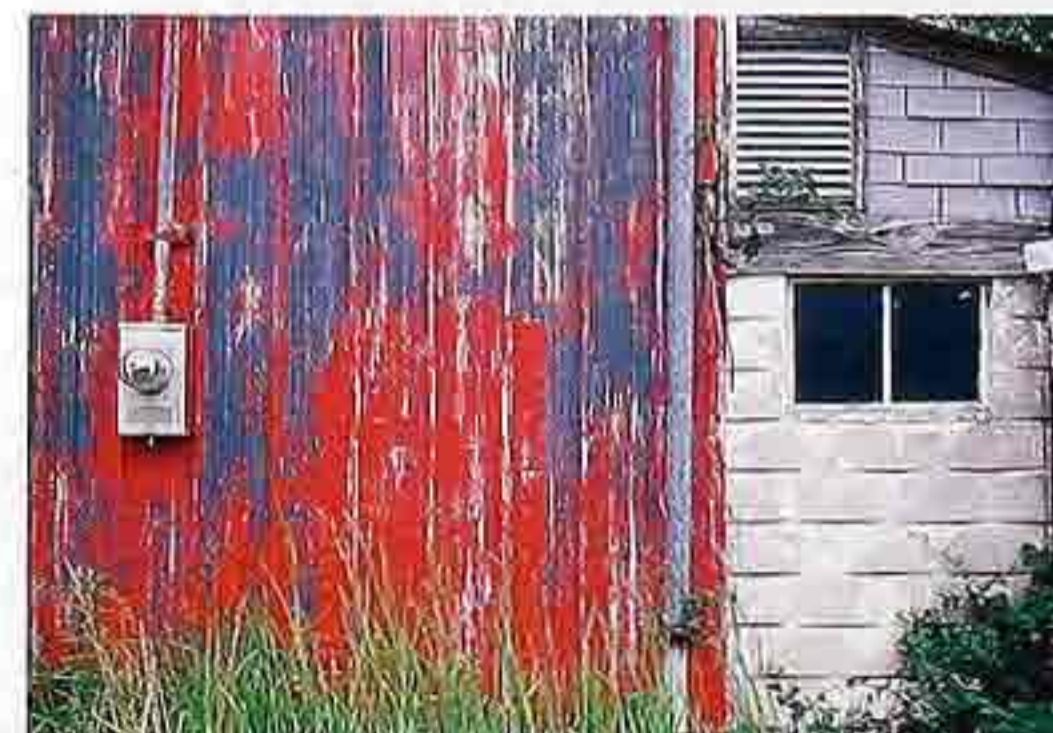
FA-100 Weathered painted vertical board-and-batten wall and adjacent masonry structure
