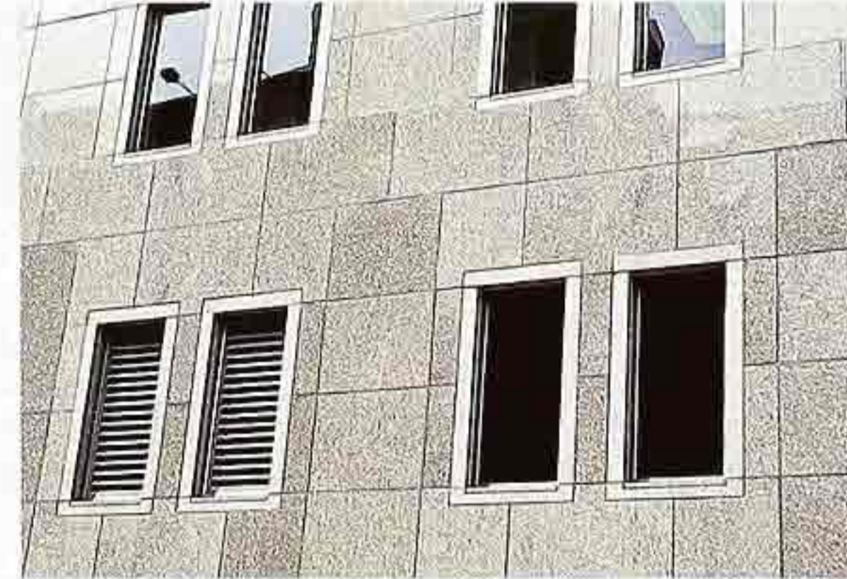
WI-161 Group of fixed windows with two louvered ventilation panels in stone surround, modern commercial building
