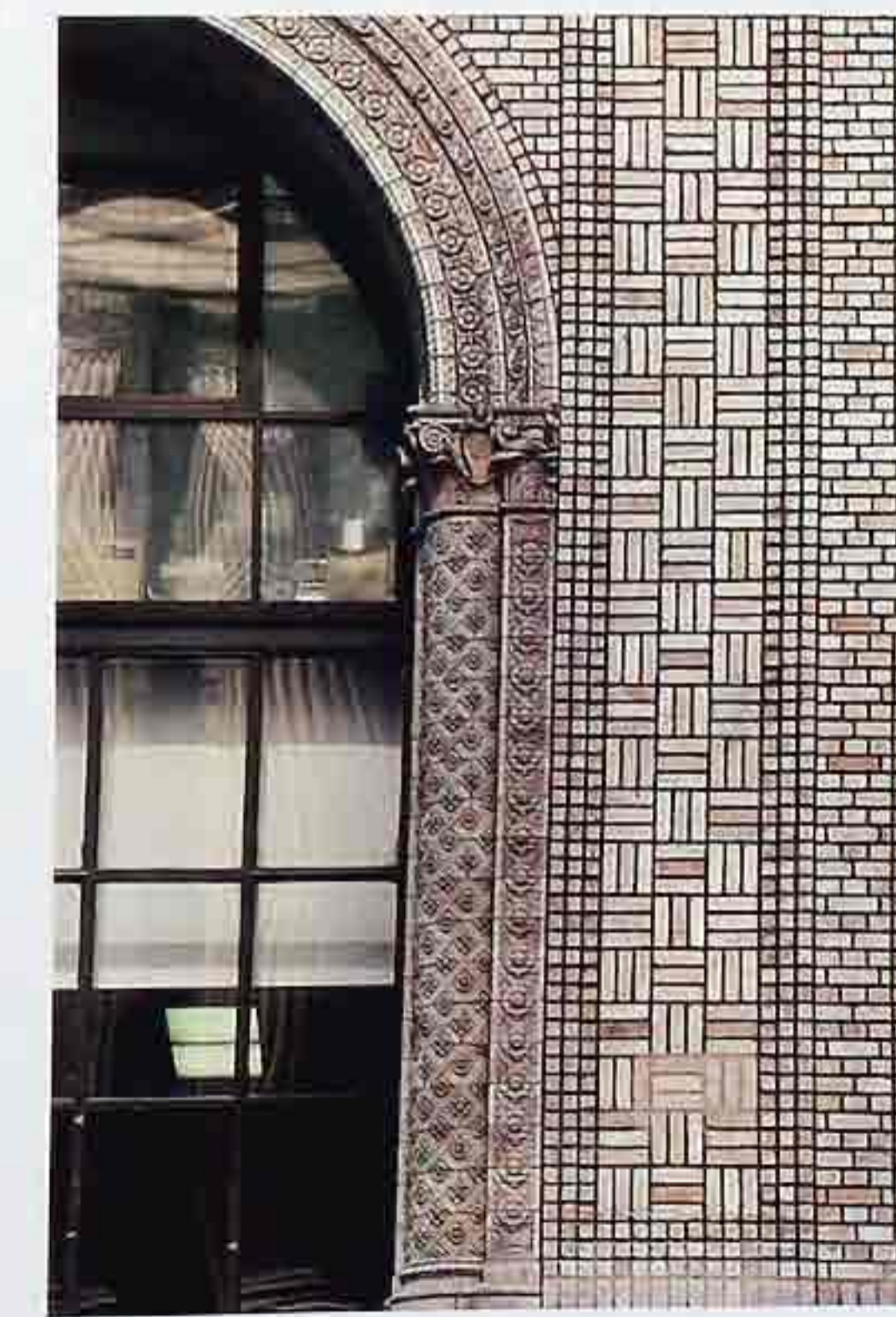
WA-204 Bands of decorative brickwork. Left to right: terracotta arch, stacked header rows, basket-weave, stacked header rows, English bond
