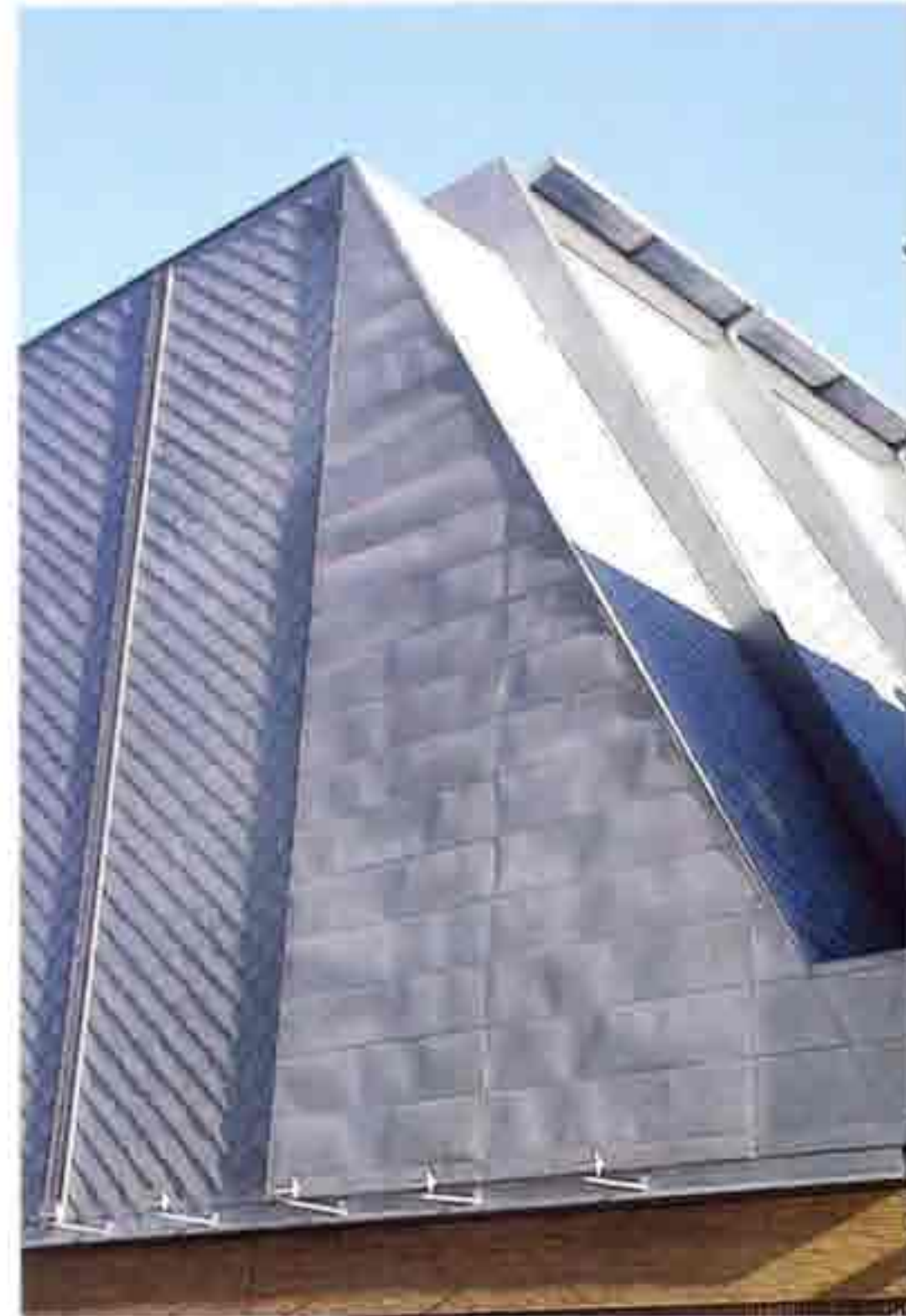
CR-31 Anodized aluminum or coated sheet steel with a variety of flat and batten seams on roof and gable wall, modern commercial building
