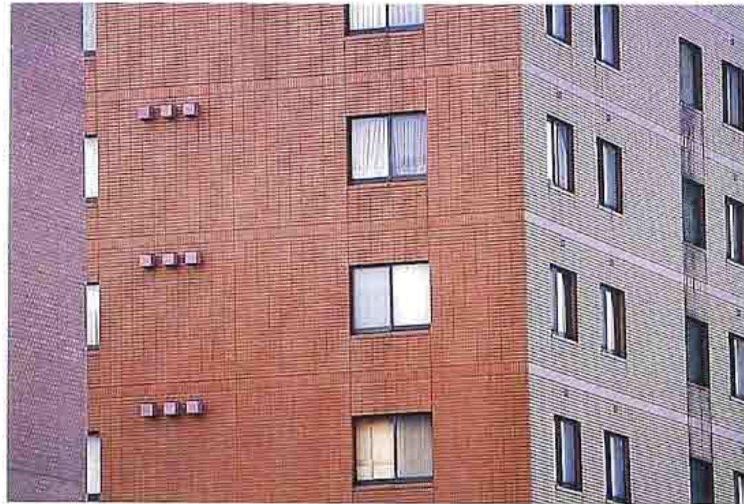
WA-205 Brick in stack bond with subtle soldier-course banding, modern apartment house
