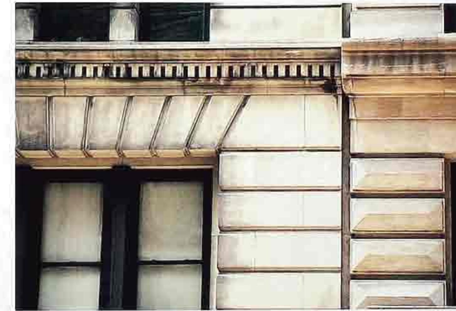
WA-87 Limestone walls. Left: bevel-cut stack bond with jack arch and dentil cornice; right: gem-cut stack bond
