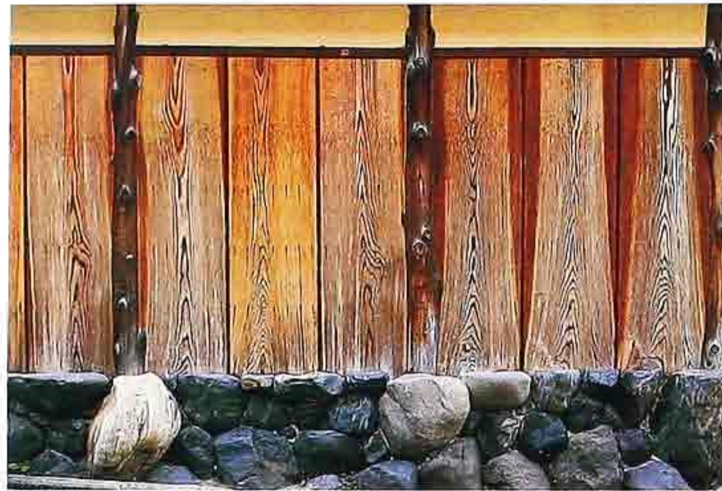
WA-44 Weathered unfinished plain-sawn planks with vertical undressed timbers on rubble foundation
