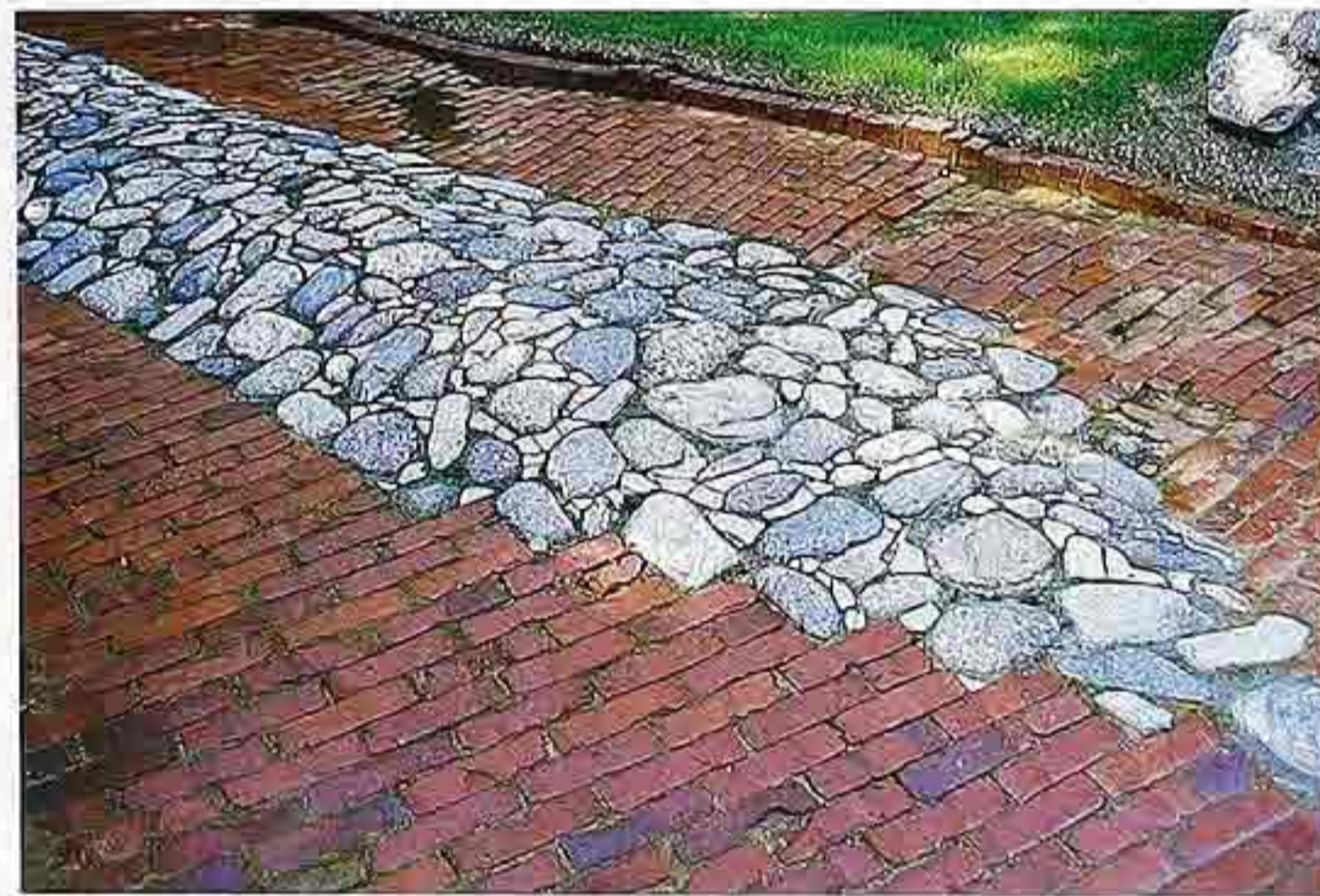
FP-38 Uncoursed fieldstone used as divider in running-bond brick driveway, Arts and Crafts residence
