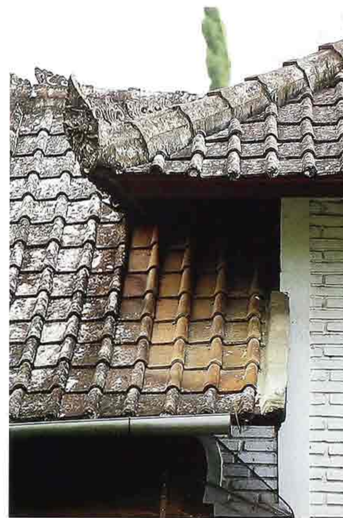
CR-40 Weathered terracotta pantile with antefix at end of ridge tiles on hip, Balinese house
