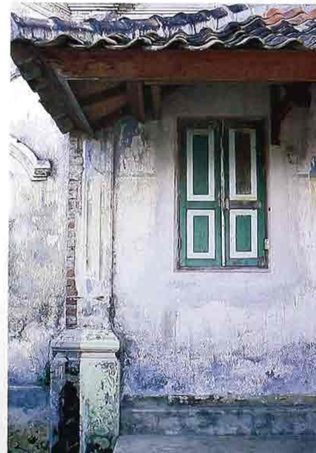
FA-95 Weathered painted stucco over brick
