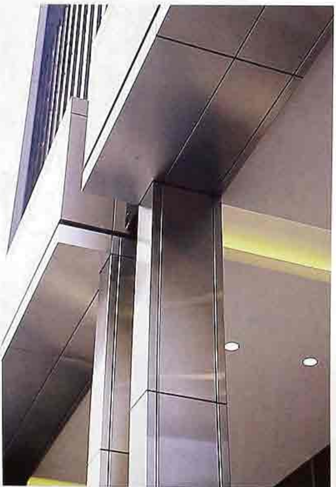
CP-124 Steel frame clad with possibly stainless steel panels, modern commercial building
