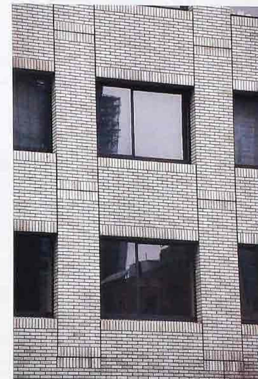
WA-180 Brick panels in running bond articulated by joints and soldier courses; soldier courses top and bottom of windows, modern commercial building
