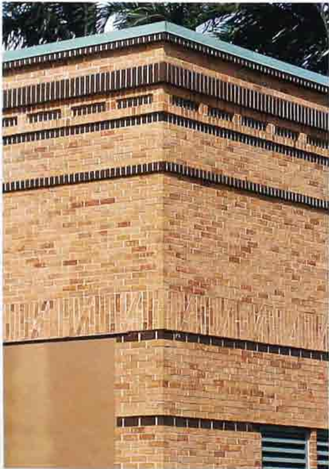
WA-191 Corner detail of bands of running bond, rowlock and soldier courses in contrasting colors, modern commercial building
