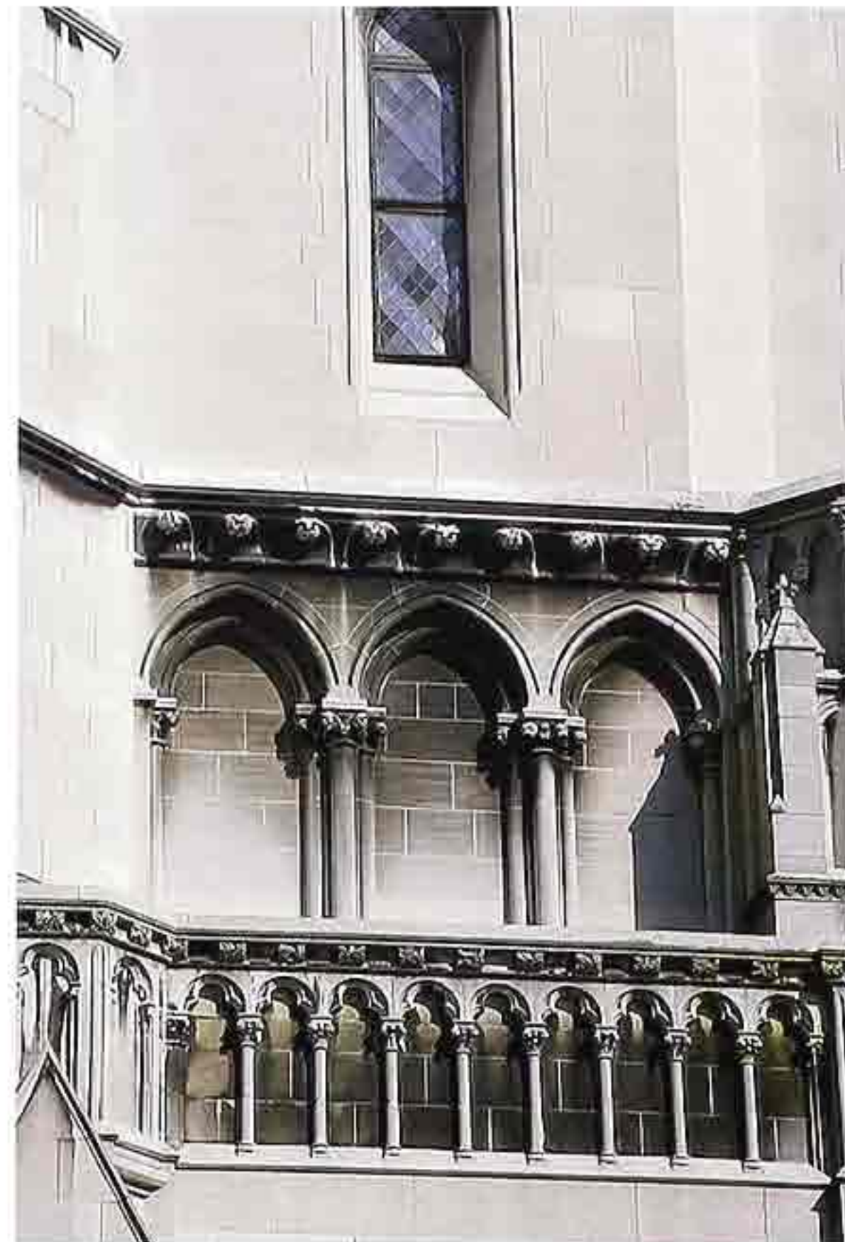
CP-171 Blind arcade: drop arches and trefoil blind arcade on Gothic-style facade
