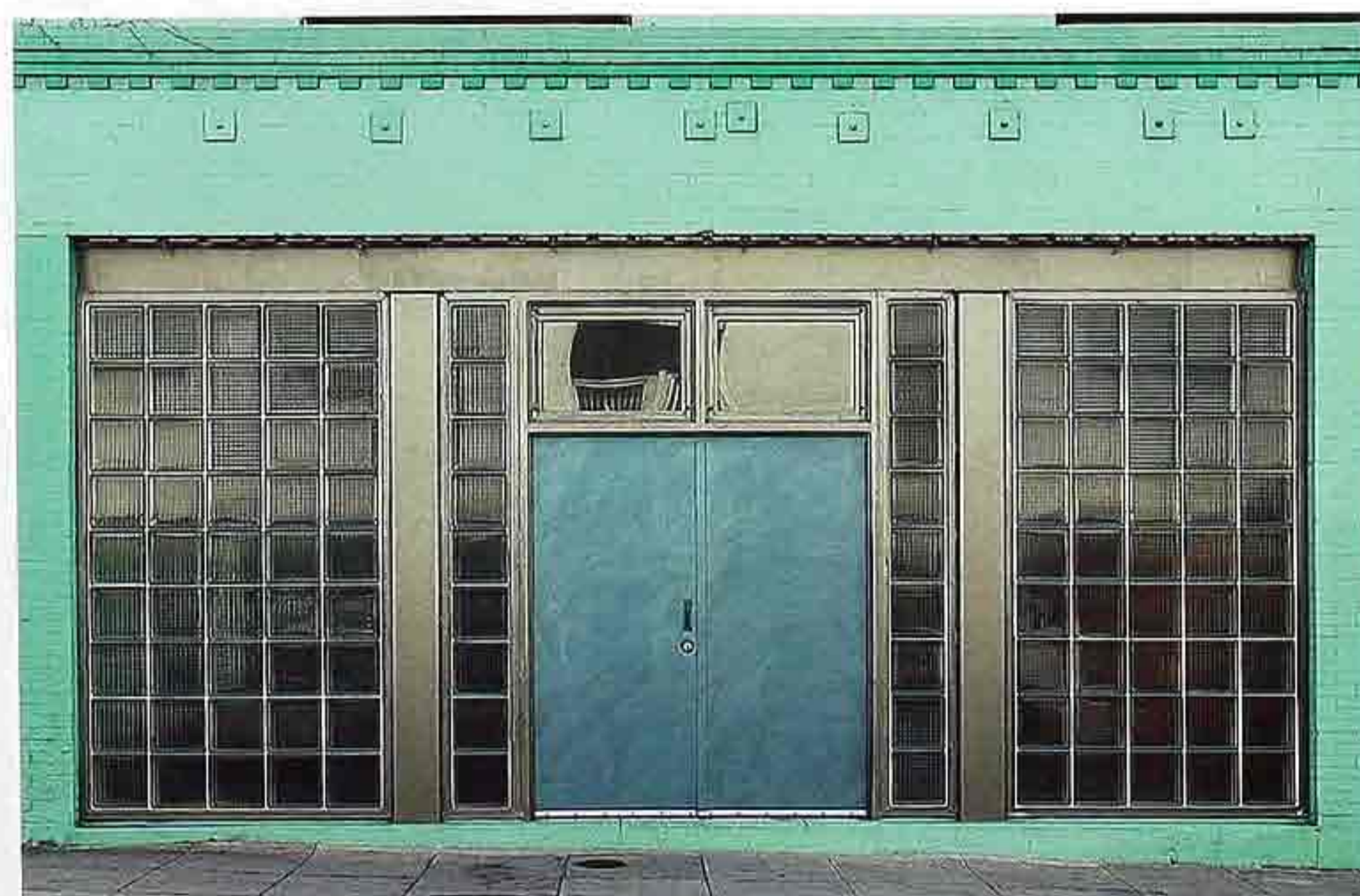
DW-103 Painted metal double doors flanked by side lights, stainless steel panels, and window wall
