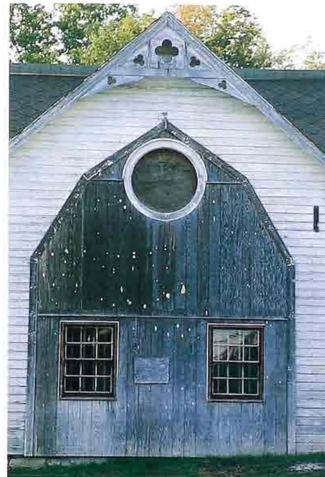
WA-22 Painted clapboard gable-end wall with gable ornament and exposed vertical board cladding
