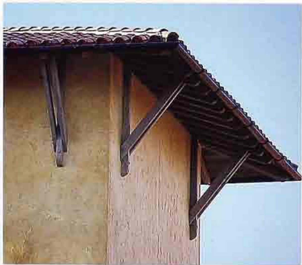
CR-107 Wood eave brackets supporting mission-tile hipped roof, American Southwestern mission-style house
