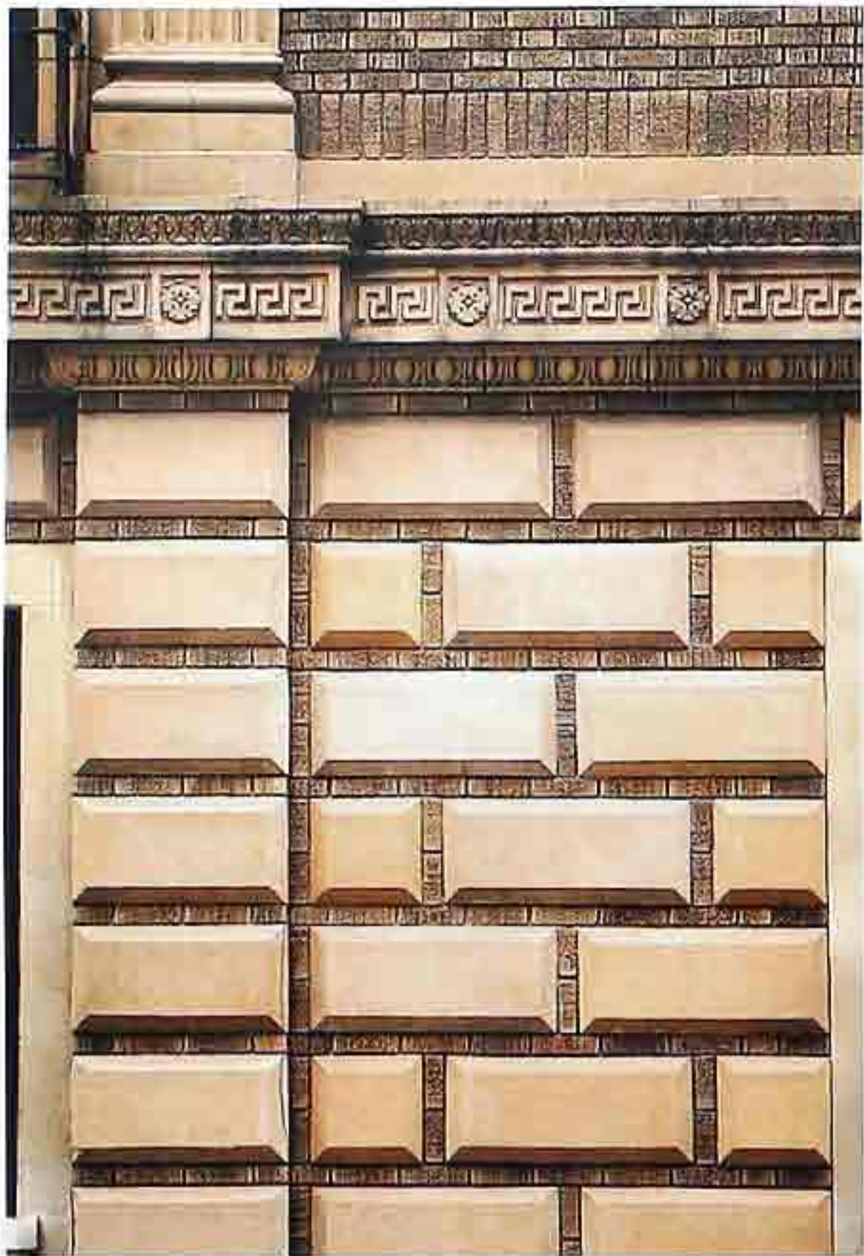
WA-290 Rusticated stone blocks in running bond, surrounded by brick; egg-and-dart pilaster cap and molding, with relief ornament band between stories
