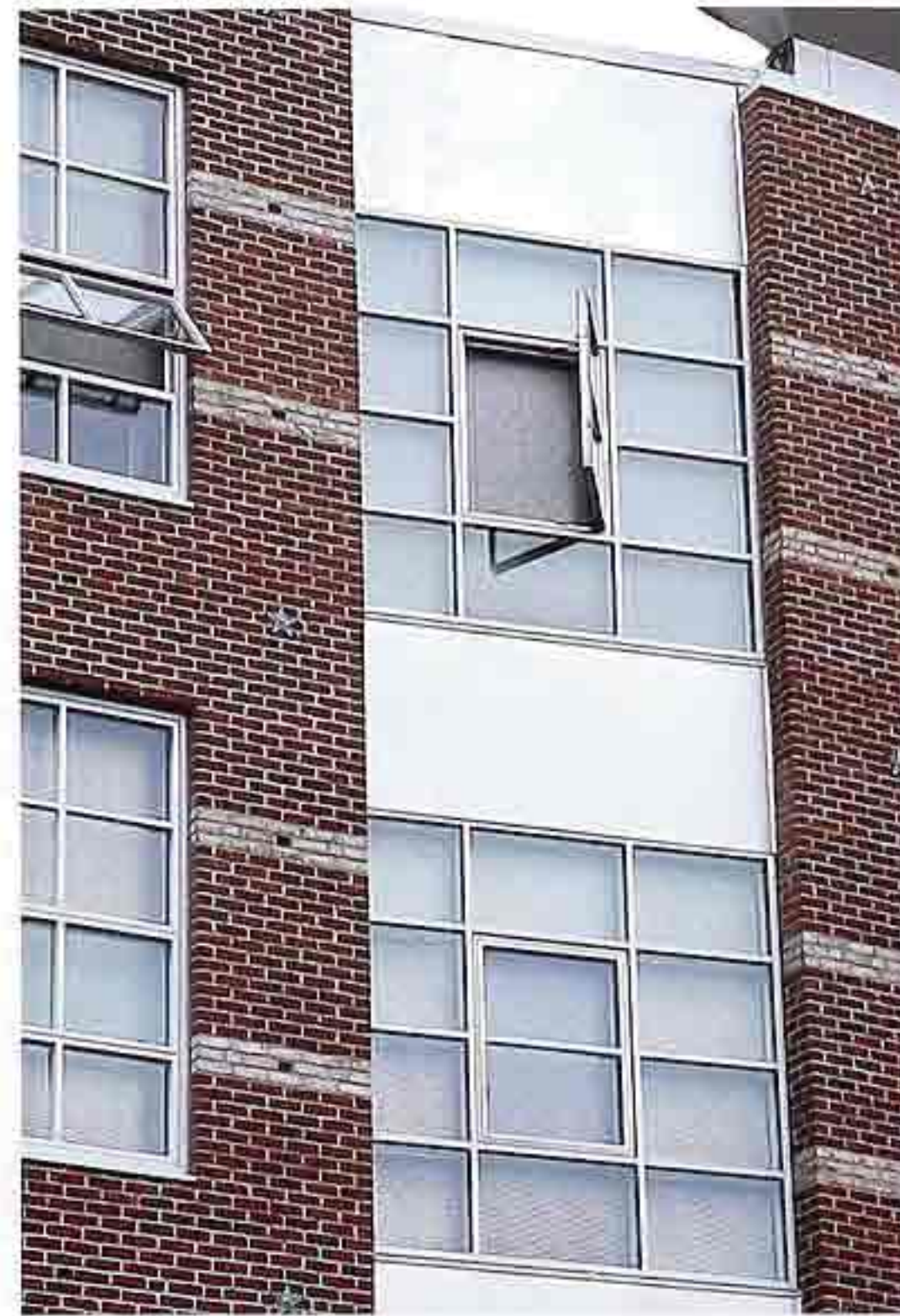
WI-39 Casement windows (center) and awning window (left) set in fixed lights; extruded aluminum mullions, modern apartment house
