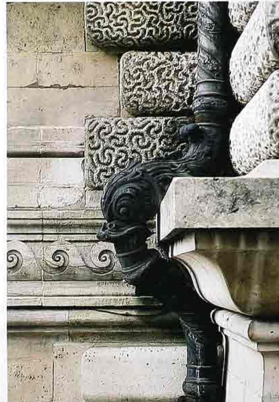
CR-158 Copper drainpipe and rainwater head
