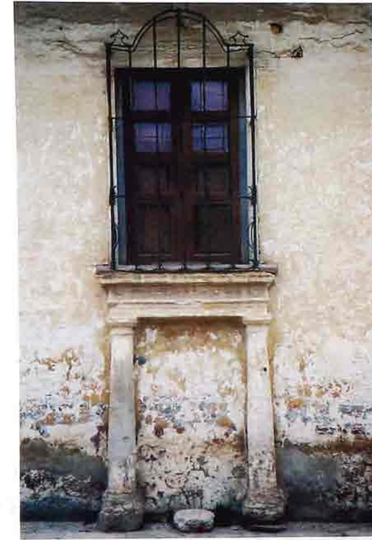
WA-252 Weathered stucco wall surrounding balcony with stucco-covered pillars
