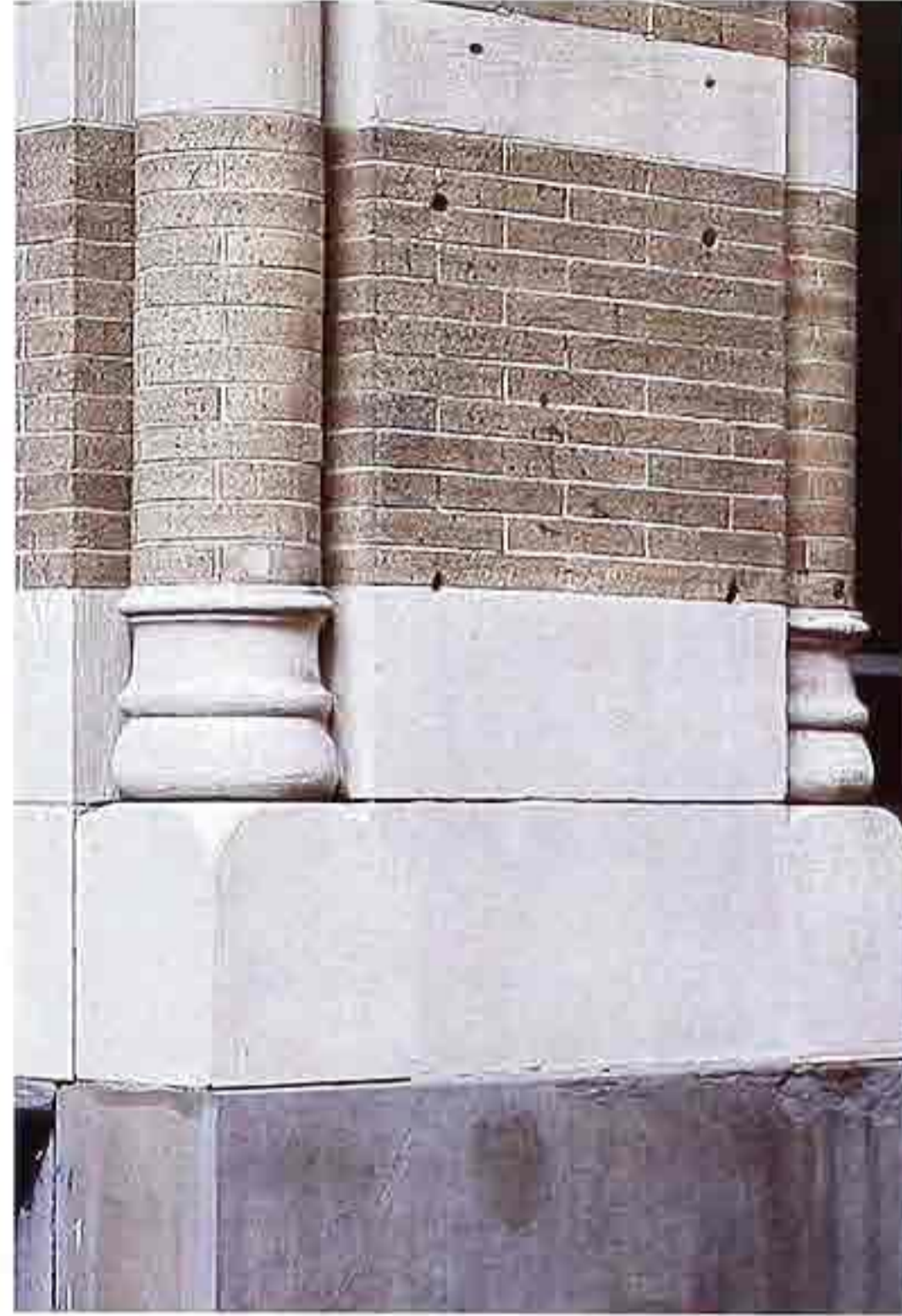
CP-42 Banded brick and stone jamb-shafts; base with shallow, elongated scotia over torus on plinth with scalloped corner
