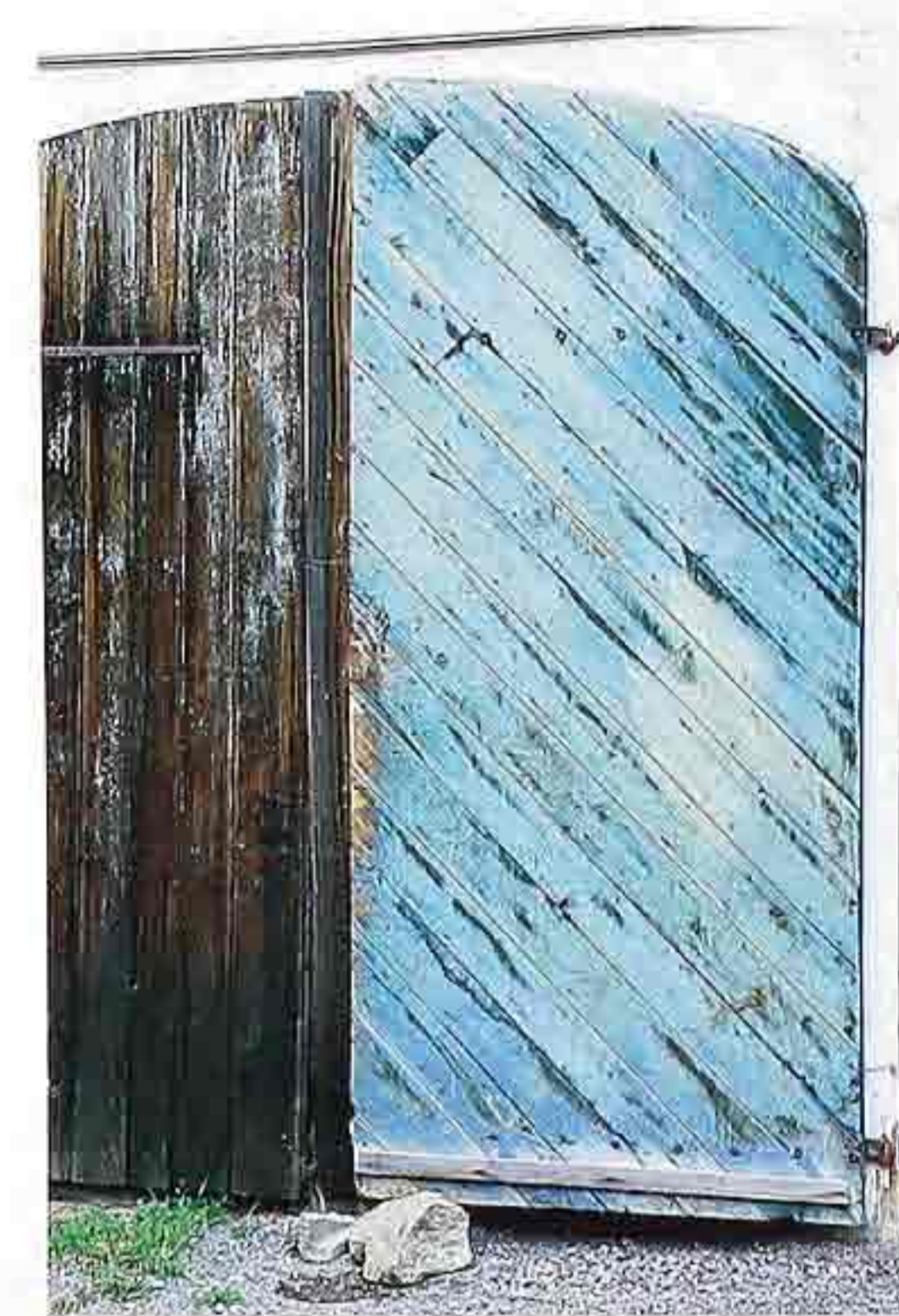
DW-34 Weathered wood double doors with rough-sawn vertical planks and painted diagonal planks
