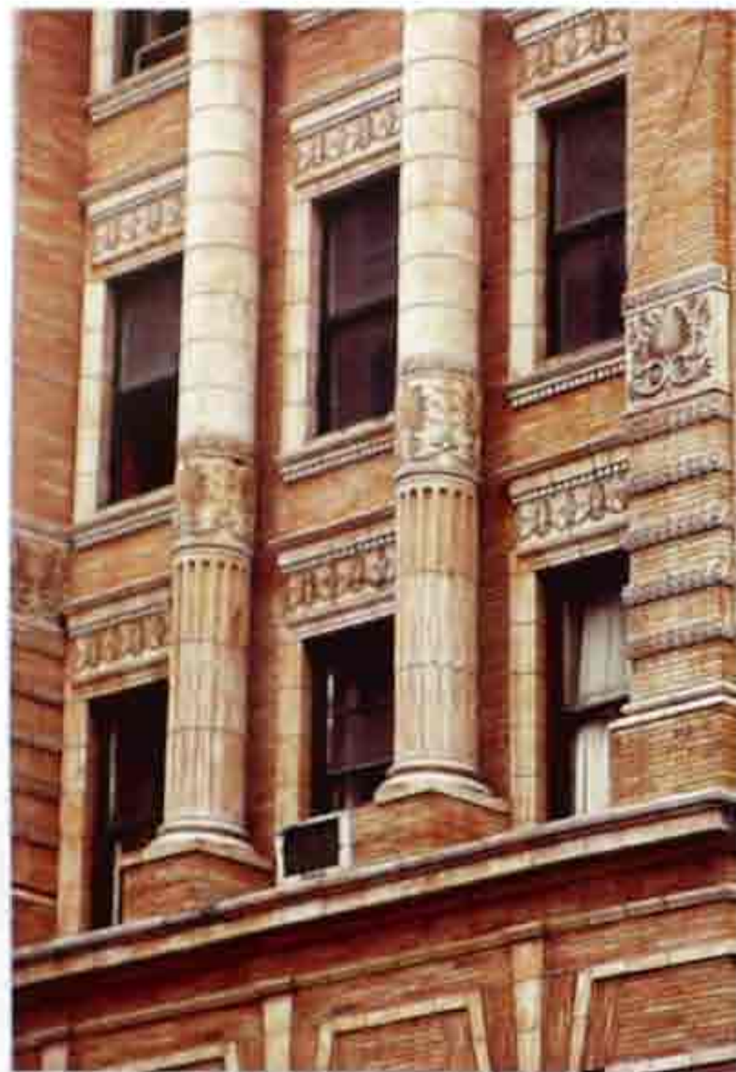
CP-65 Center: partially fluted shafts with band of anthemion ornament and visible joints between drums; right: flat pilaster with brick and ornamented bands
