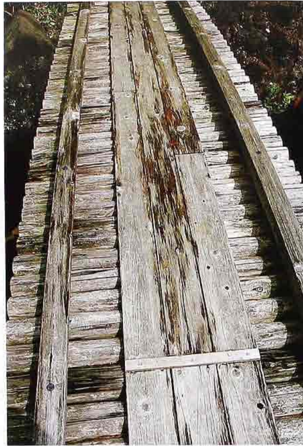
FP-2 Dressed logs with center-sawn planks and wood-peg construction, rustic garden bridge
