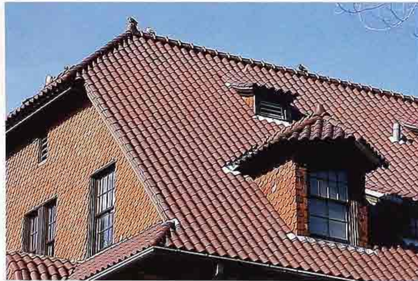
CR-87 Dormer with hipped roof on jerkinhead tile roof with scalloped terracotta tiles, gable-end wall
