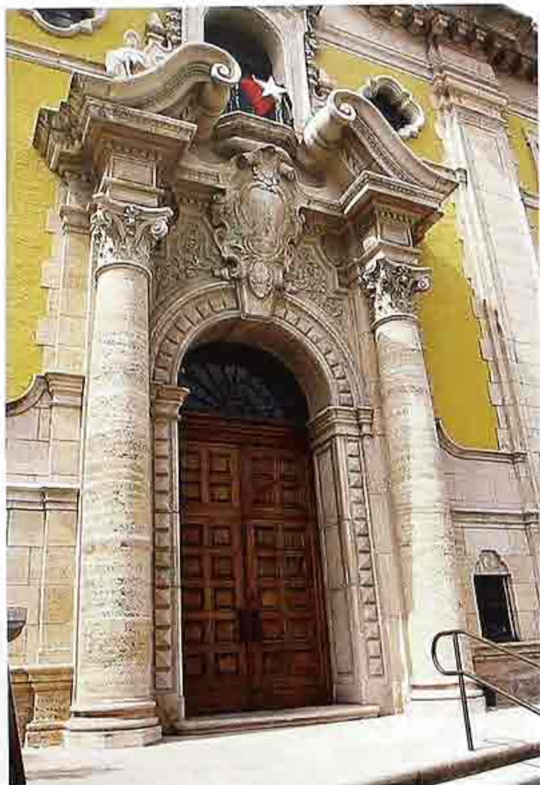
DW-72 Ornate arched entry with Corinthian capitals on engaged columns, fanlight, archivolt, cartouche keystone, and scrolled pediment
