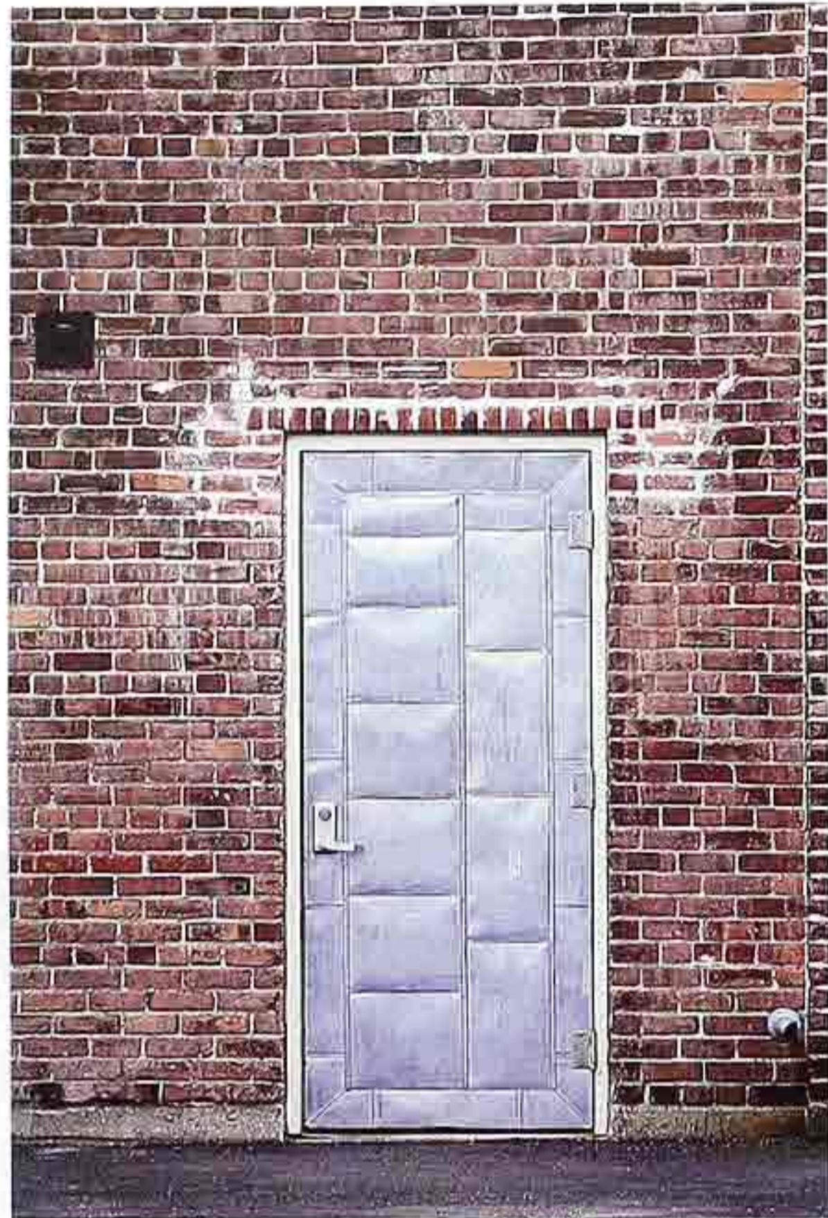
DW-52 Metal-clad door with "quilted" panels; brick surround with rowlock course above door opening
