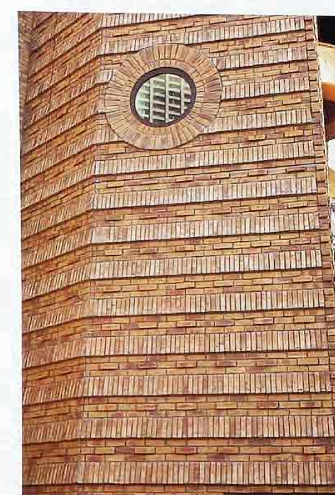
WA-202 Bands of decorative brickwork: running bond alternating with projecting soldier rows; rowlock and soldiers around roundel, modern commercial building
