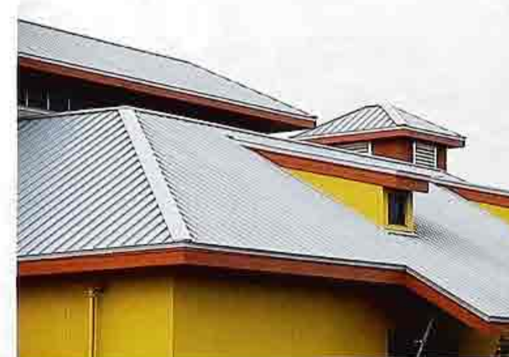
CR-101 Shed-roof dormer on metal hipped roof with standing seams, modern house
