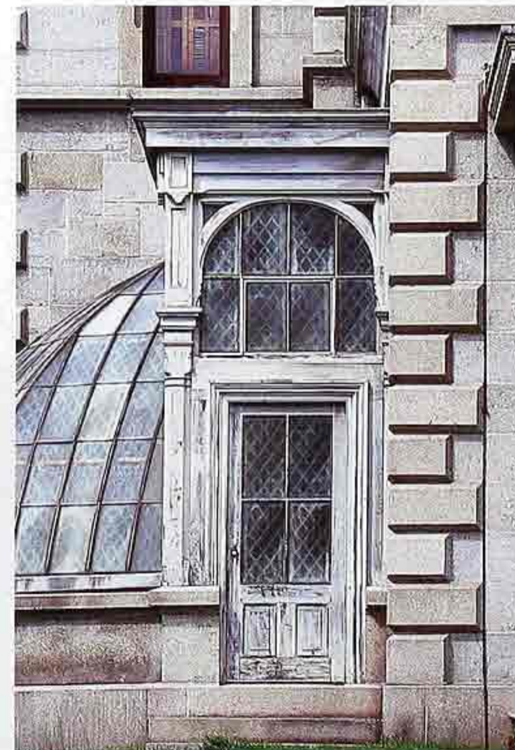
DW-78 Victorian conservatory entry: painted wood four-light door and transom light with etched glass; wood pilasters and crown molding; stone base
