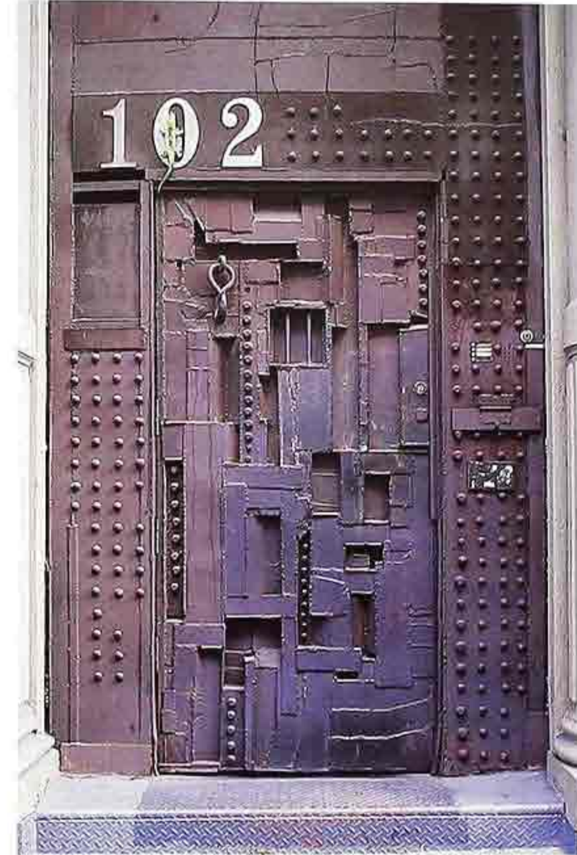
DW-55 Welded and painted metal collage applied to door and frame, with textured metal threshold
