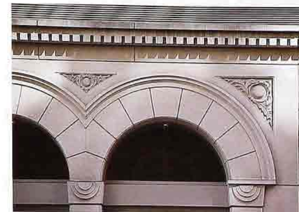
CP-142 Semicircular arches with voussoirs and archivolt, carved spandrel, and dentilated molding
