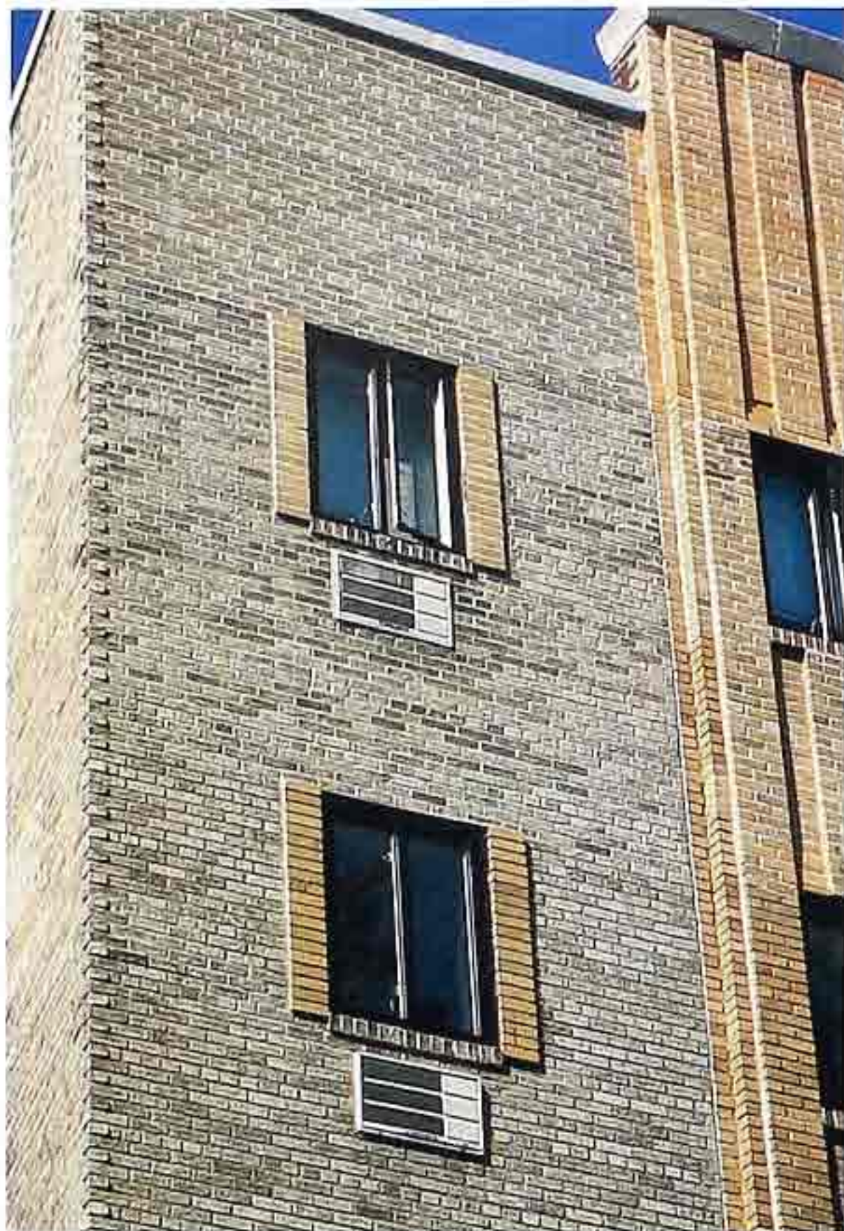
WA-183 Rusticated-brick corner; window with rowlock sill, and raised stacked bond imitating shutters, modern apartment house
