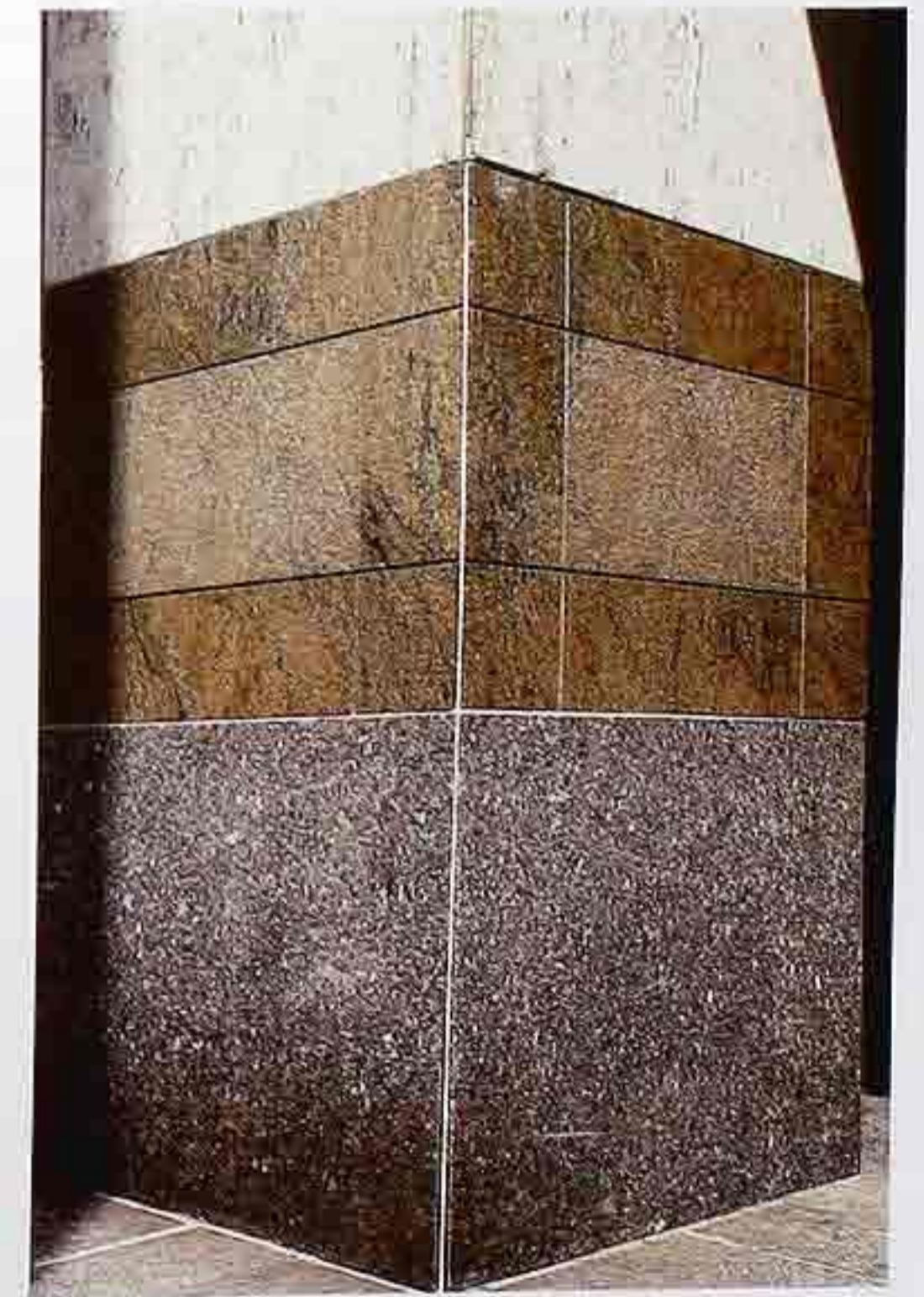
CP-48 Banded stone-veneer pier on base, grouted corner and joints, modern commercial building
