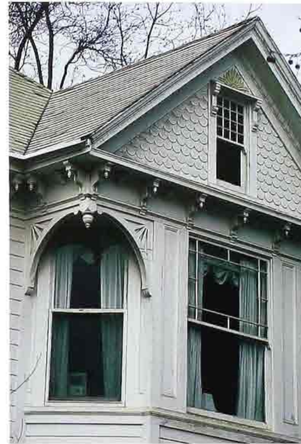
WI-51 Double-hung windows: one-over-one (left); sixteen-over-one (gable); one-over-one decorative-lights (right), 19th-c. clapboard house
