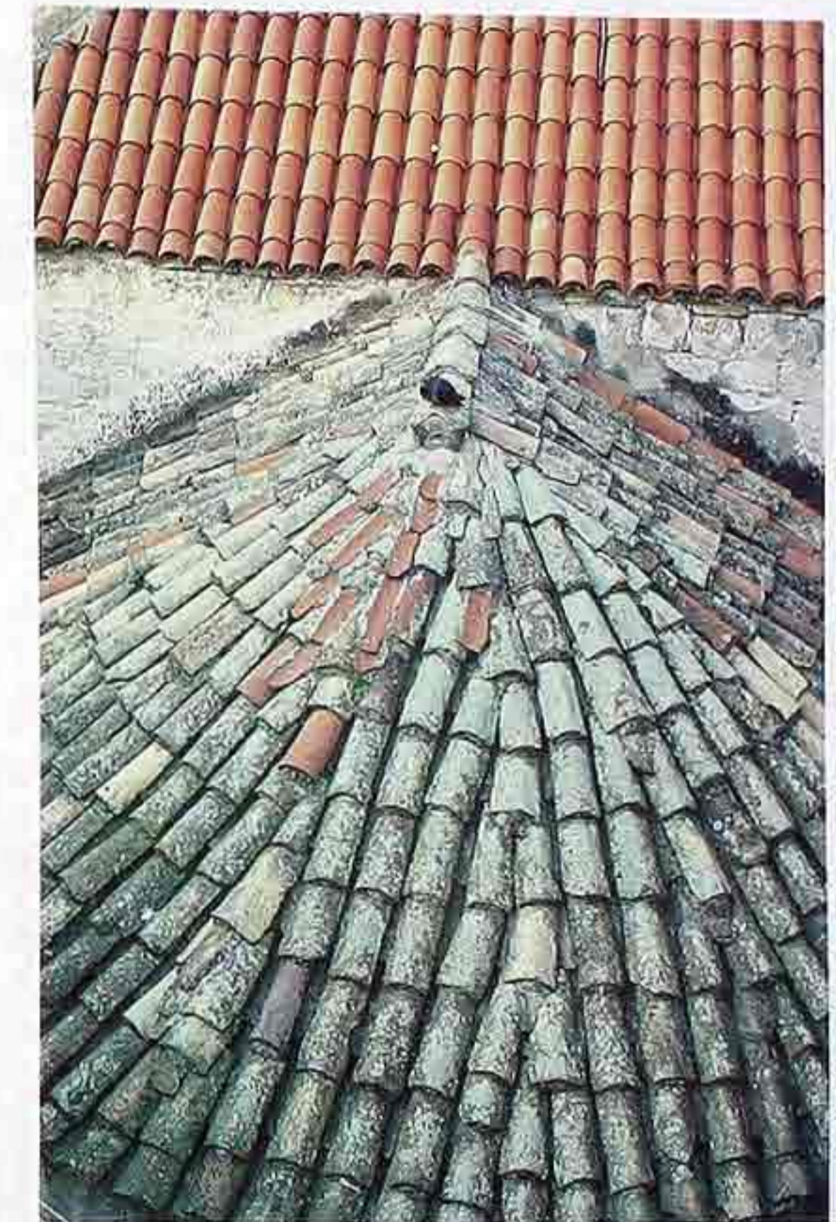
CR-41 New and weathered terracotta mission tiles. Top to bottom: shed roof; gable roof, half-cone roof
