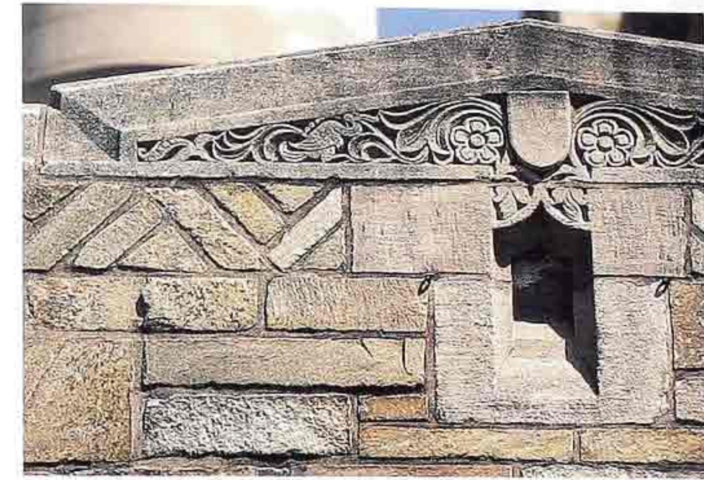
WA-86 Sandstone and quartzite in coursed ashlar below herringbone pattern; Indiana limestone ornamented cap
