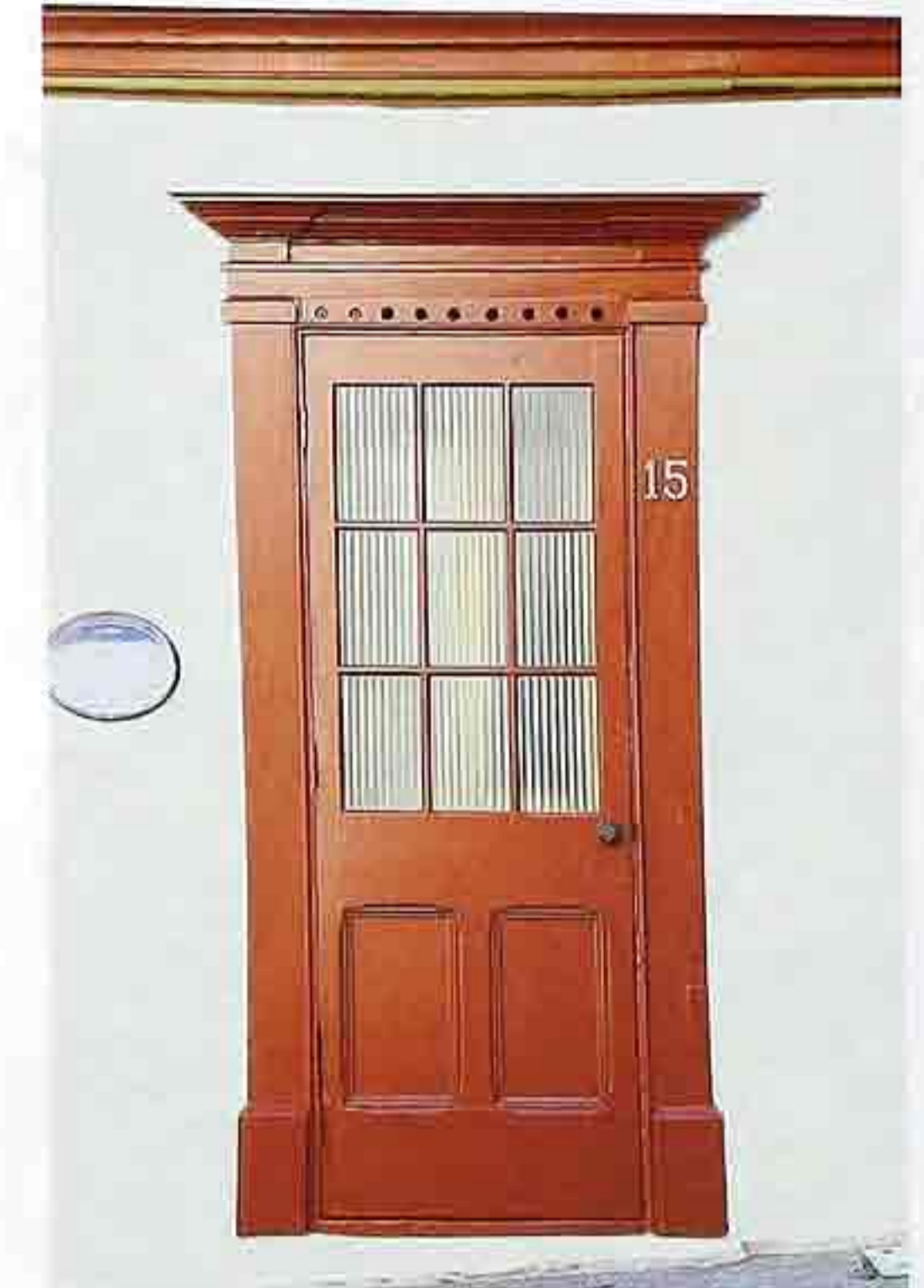
DW-20 Painted wood door; ribbed-glass panel with nine lights; wood panels flush-molded; pilaster frame
