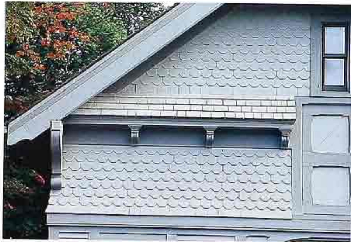
FA-47 Painted sawn shingles in fish-scale pattern, gable detail
