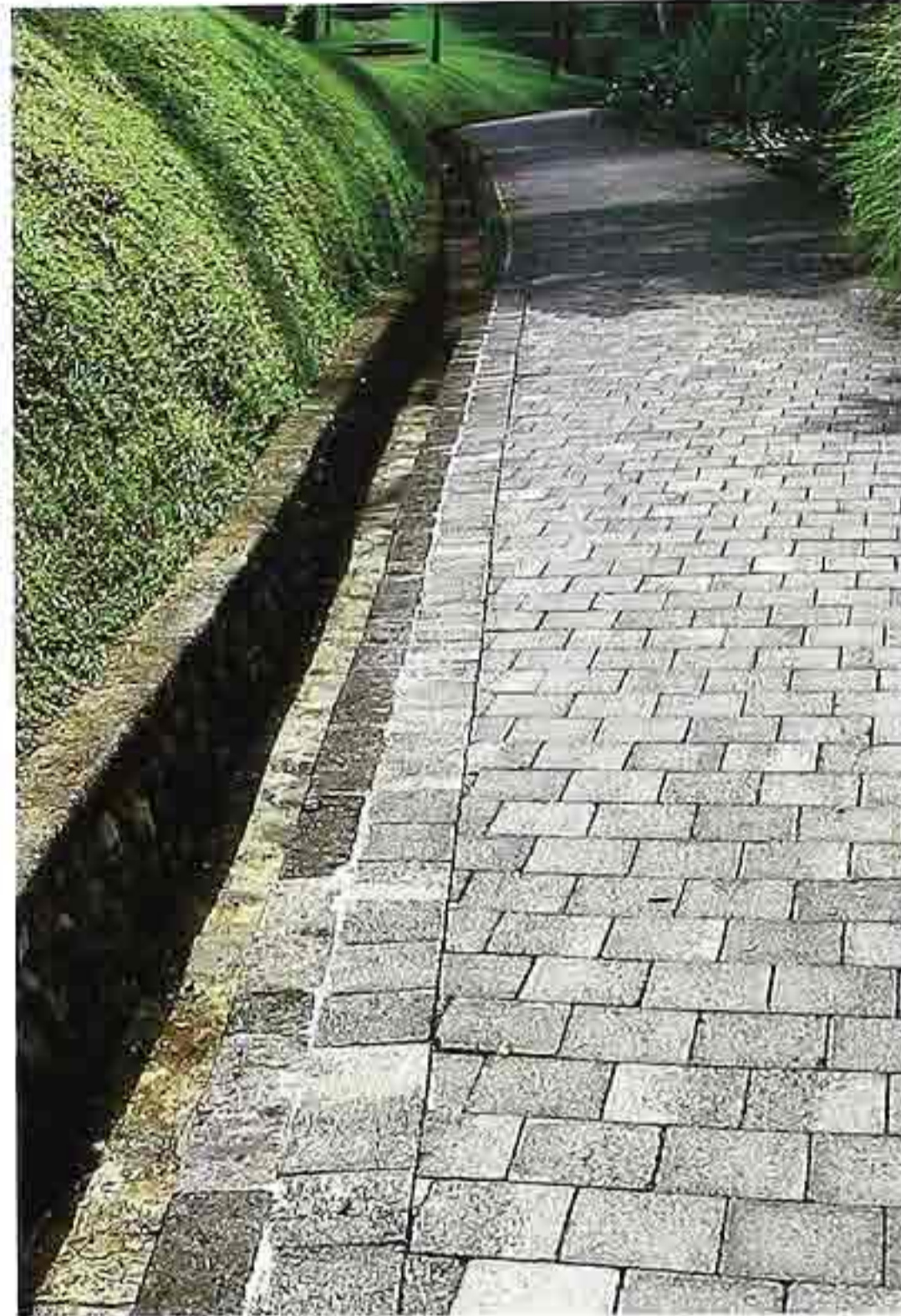
FP-20 Dimension fieldstone in running bond with soldier-course border and stone gutter, garden walkway
