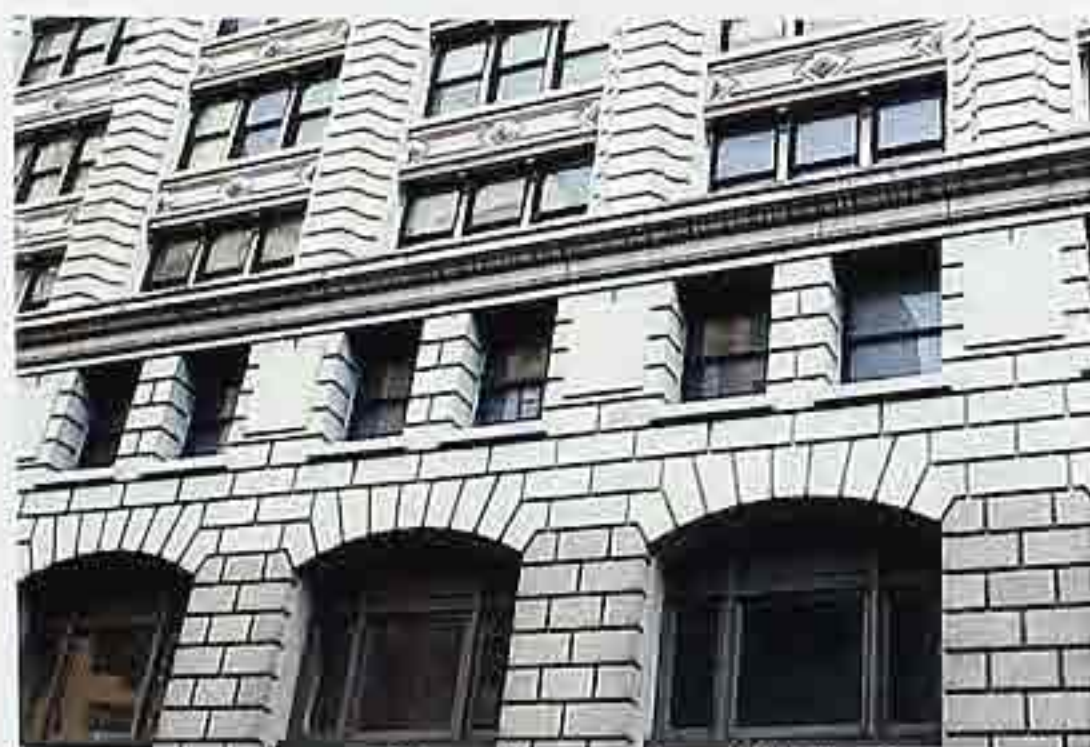
WA-118 Limestone in running bond with cornice; upper story with carved spandrels; varied window openings
