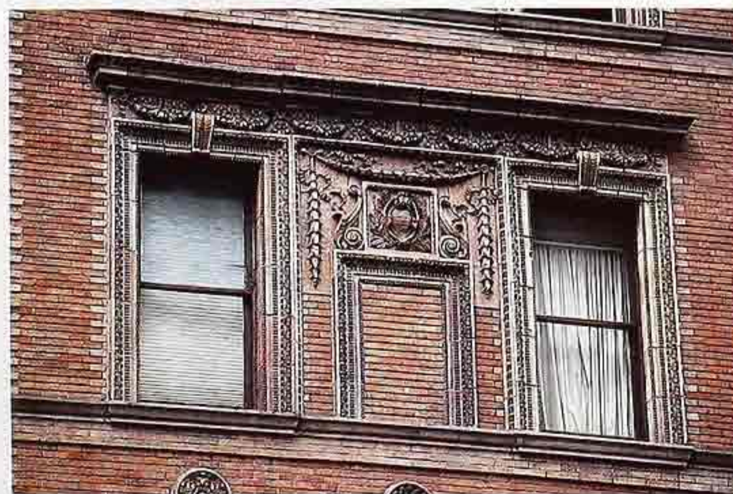
WI-128 Terracotta cornice with garlands around windows with terracotta casings; blind window under cartouche
