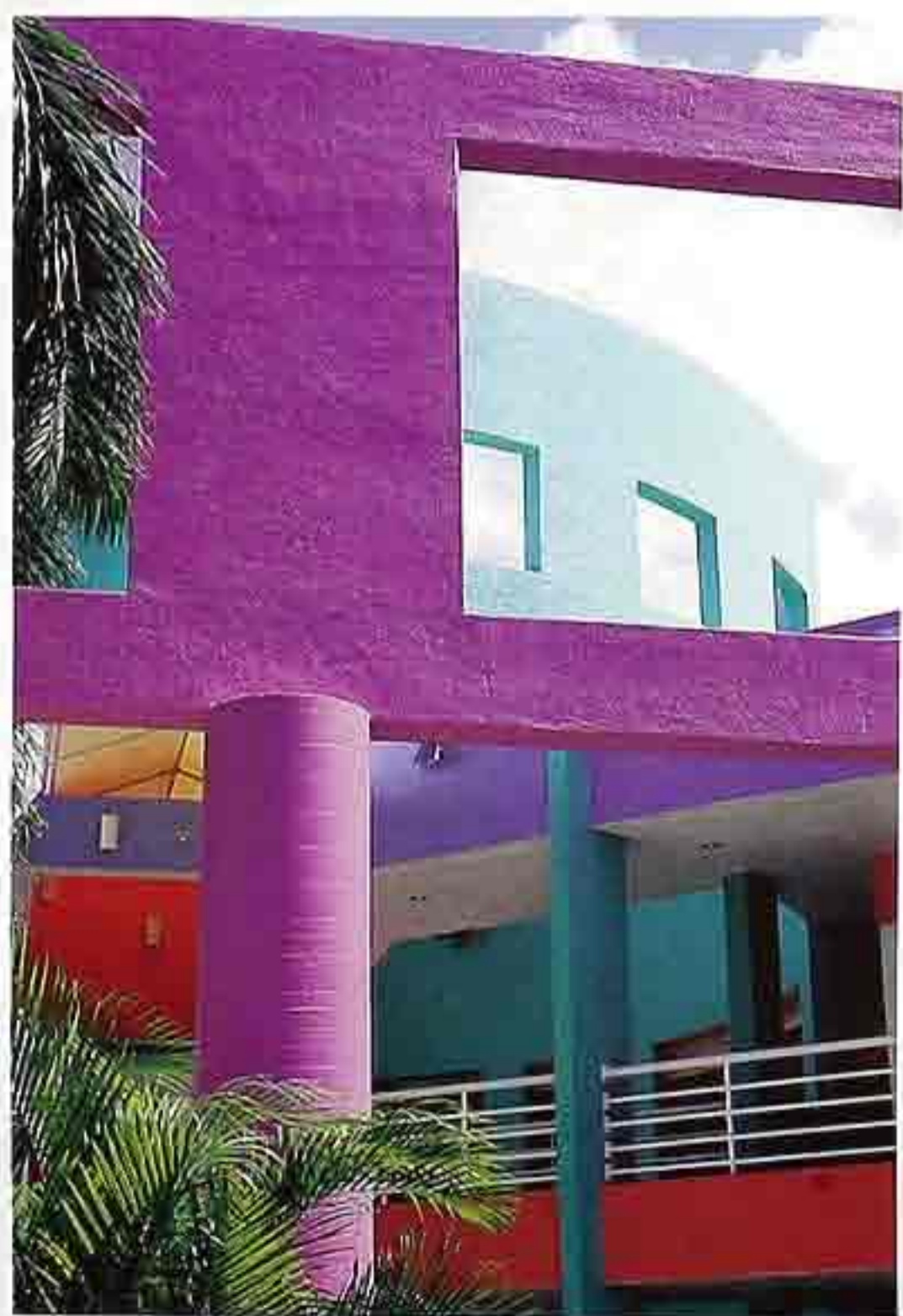
CP-114 Painted poured-in-place concrete pier supporting a steel frame with cladding finished with spray-on stucco
