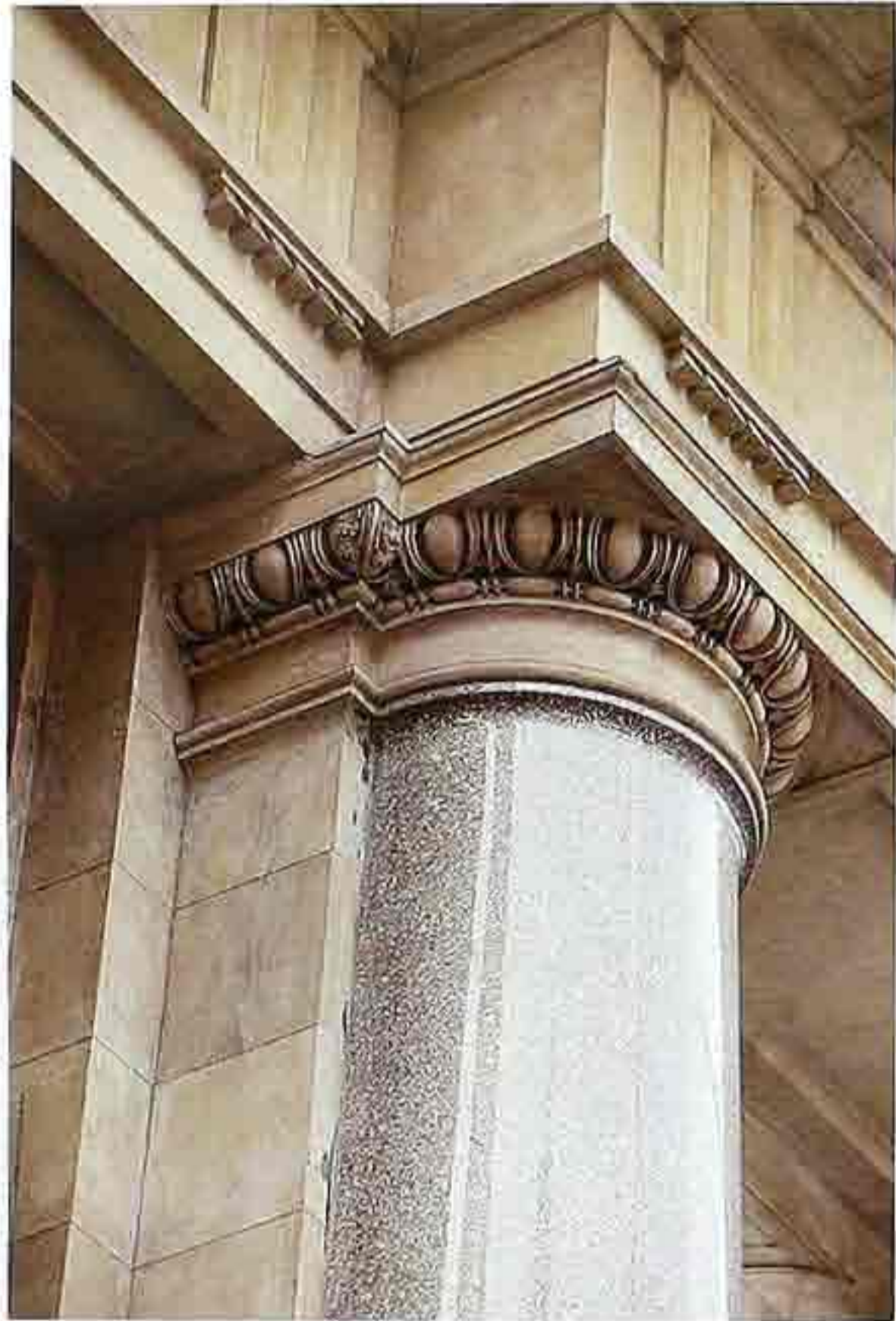
CP-18 Roman-style Doric capitals on adjacent engaged column and pilaster, egg-and-dart echinus, and typical Doric entablature
