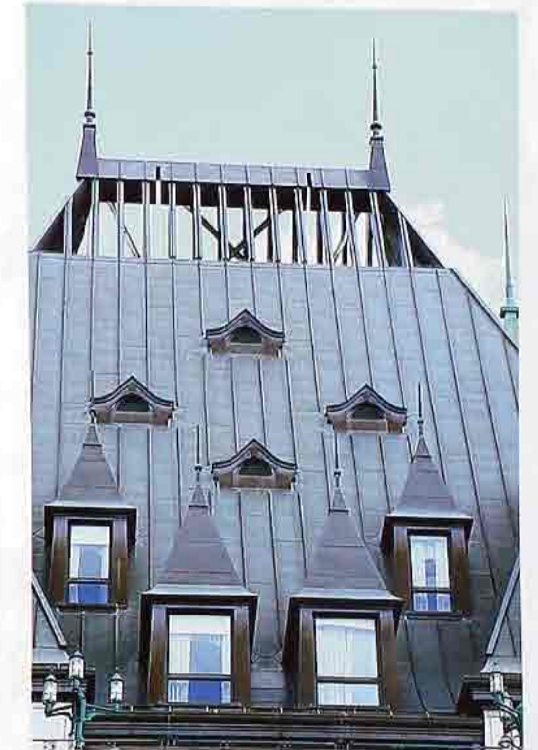
CR-100 Four flared-gable roof dormers above flared pyramidal roof dormers on metal hipped roof
