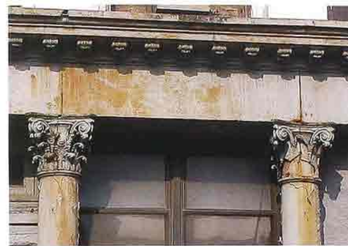
OM-92 Classical entablature: plain architrave, no frieze, modillion band on cornice on weathered tin facade. Weathered tin Corinthian capitals
