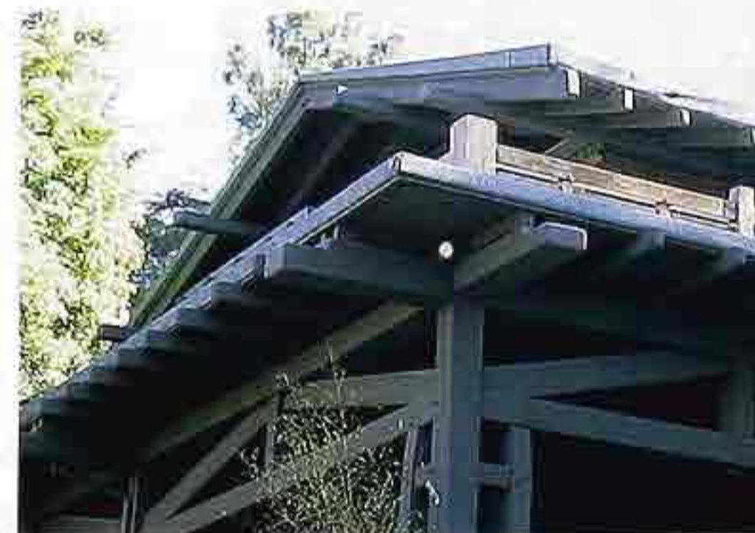
CR-111 Eaves of hipped roof on notched cross-beams, Arts and Crafts house
