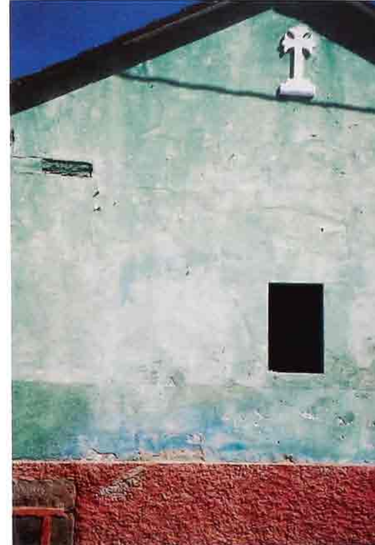
WA-251 Painted stucco textures on gable-end wall
