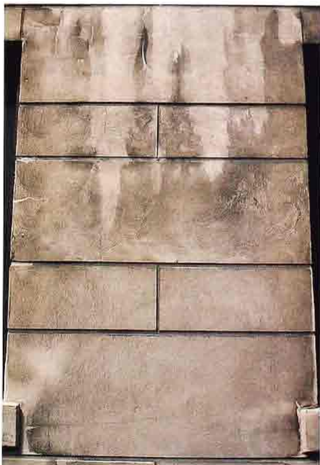
WA-75 Coursed ashlar limestone with sand finish, water-damage weathering
