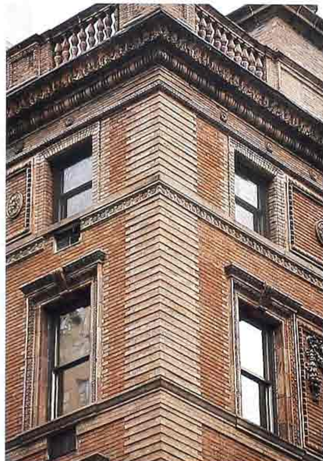
WA-192 Corner detail of brick and molded decorative brick or terracotta, 19th-c. apartment house
