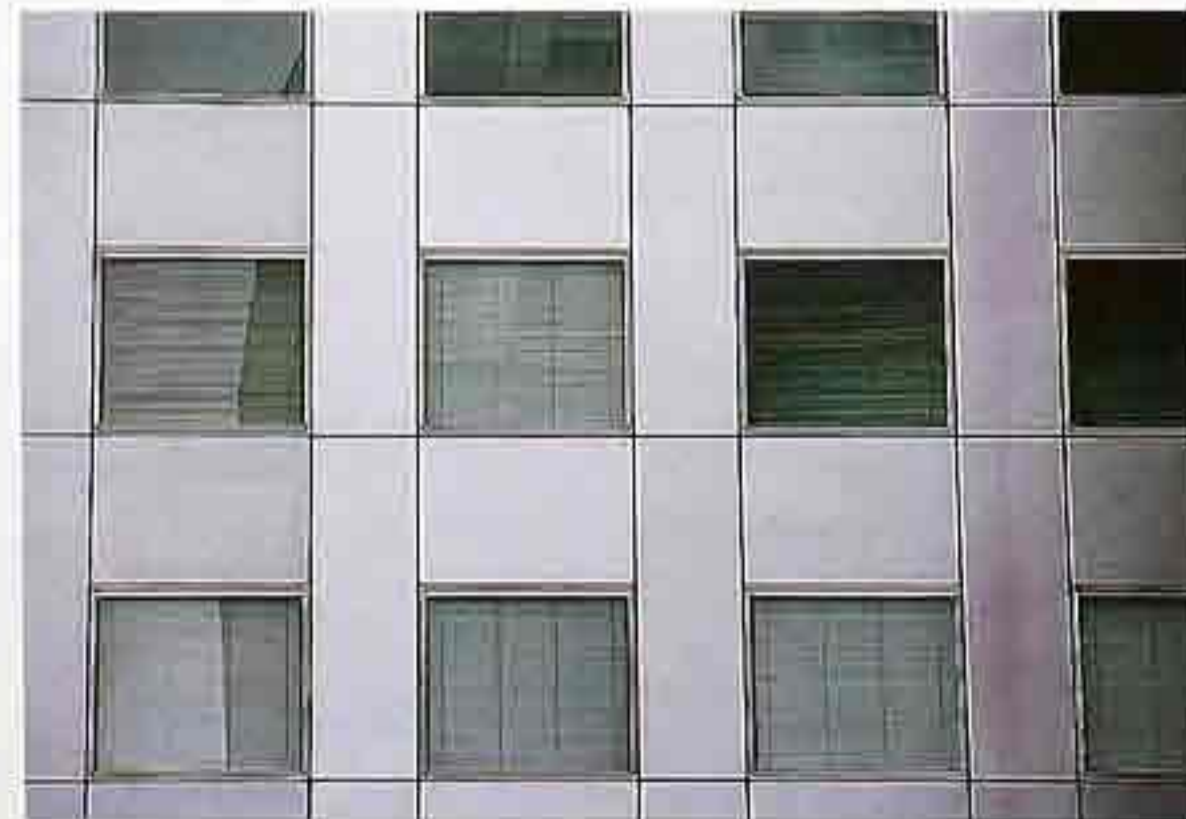
WI-162 Interlocking design of square windows with metal spandrels and surround, modern commercial building
