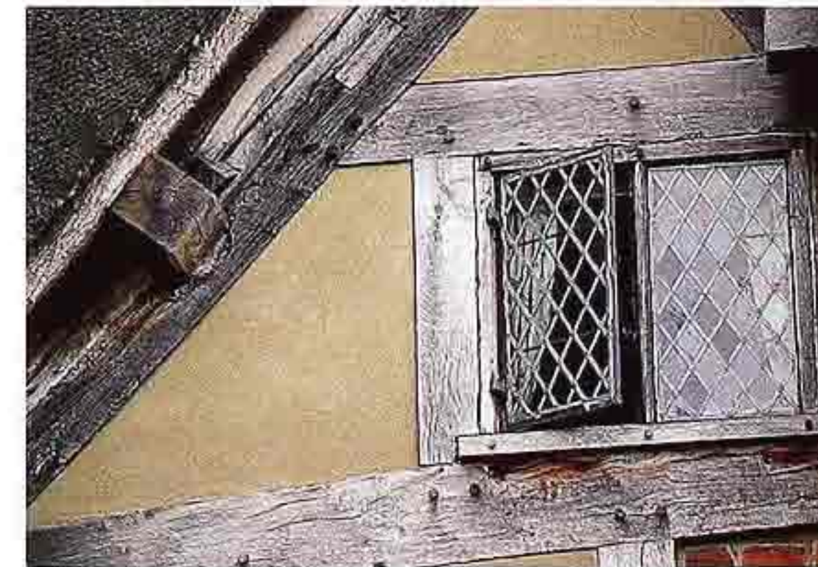
WI-27 Leaded double-casement windows with comes in a diamond pattern, 16th-c. half-timbered English house
