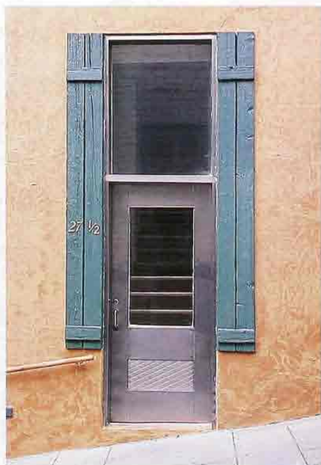
DW-61 Stainless steel door with single light and transom light; frame flanked by shutters, modern doorway in older urban building
