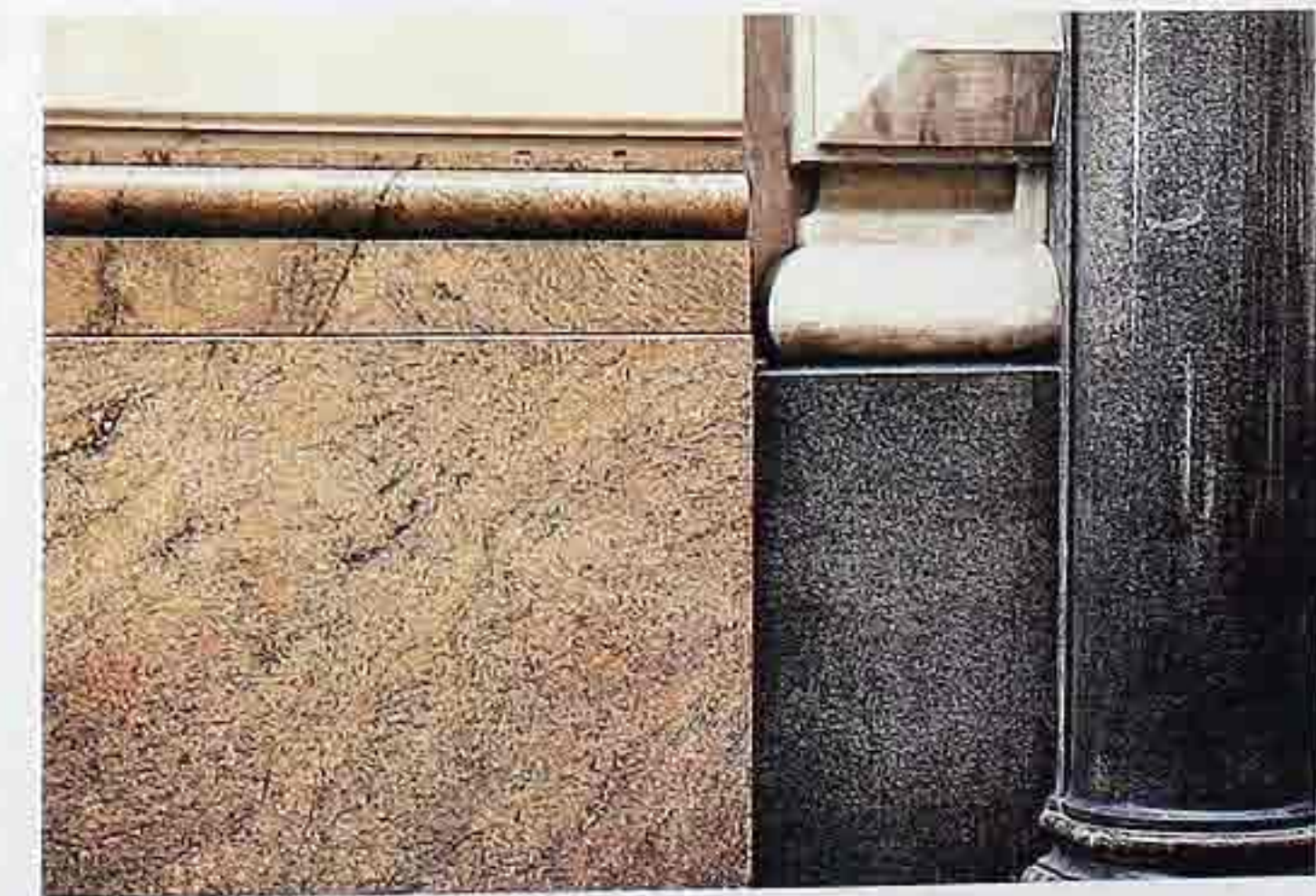
WA-88 Polished granite and marble. Left to right: granite-veneer base with bead molding; granite plinth with marble ovolo molding on base; polished granite engaged column
