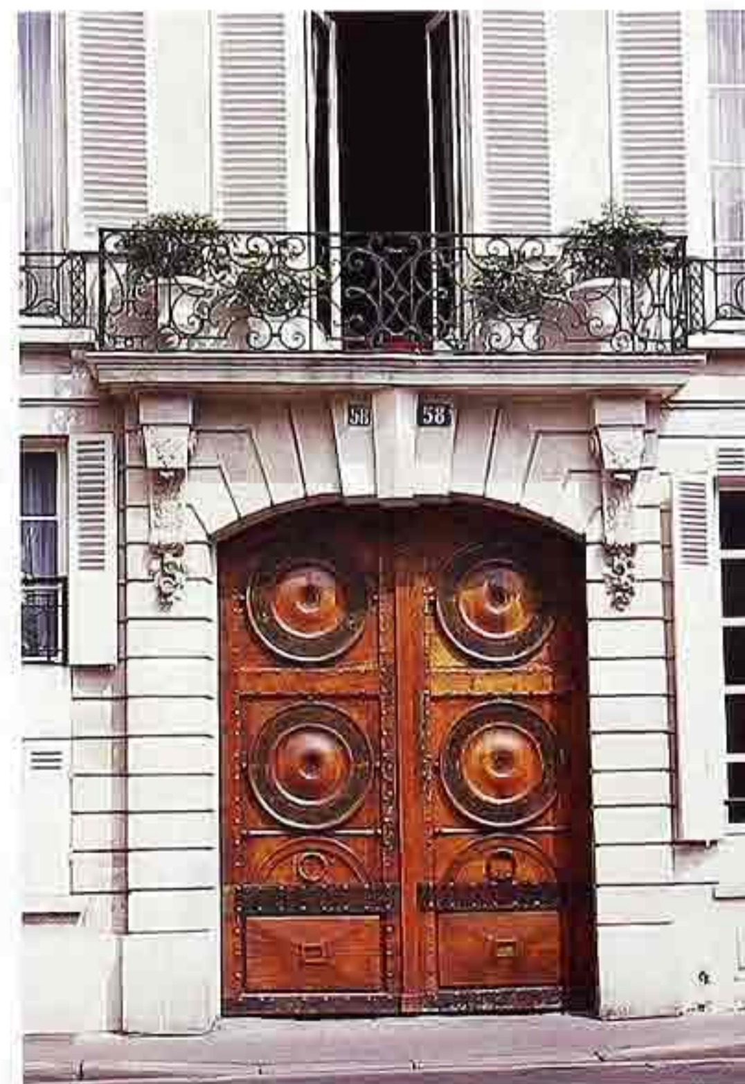
DW-75 Stone segmental arch with carved wood double doors; keystone and corbels supporting a balcony, Parisian apartment house
