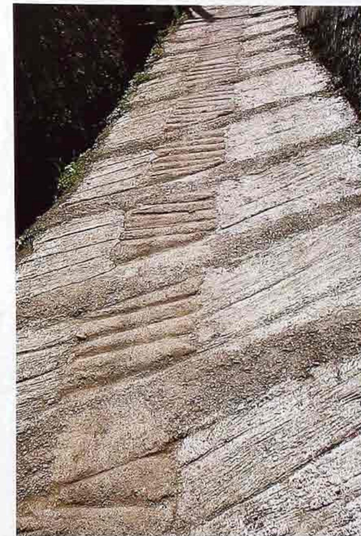
FP-79 Concrete textured to resemble rough wood planks, possibly cast-in-place, with texture produced by forming materials
