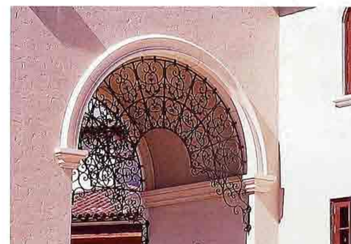
CP-143 Semicircular arch in stucco wall with molded impost blocks, archivolt, and inset wrought-iron tracery
