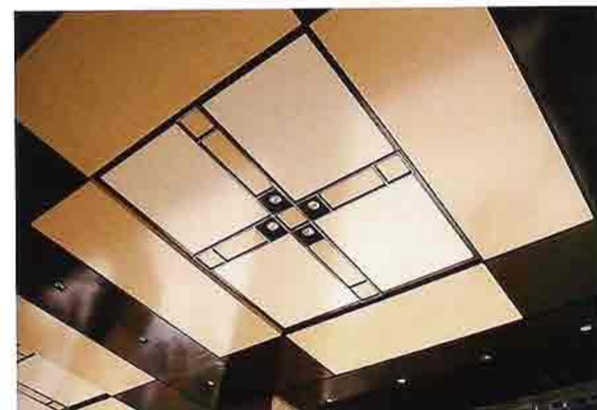
CR-13 Ceiling of contrasting colored enameled panels in Art Deco design on portico
