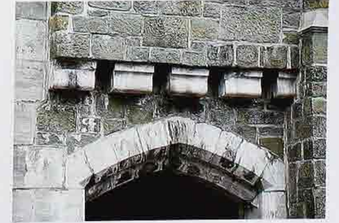
CP-155 Two-centered surbased arch (arch rising less than half its span) in castle entry under corbelled jetty
