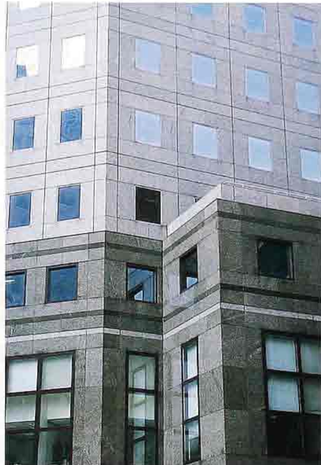
WA-141 Polished granite veneer with flush-mounted fixed windows in polychrome curtain wall, modern commercial building
