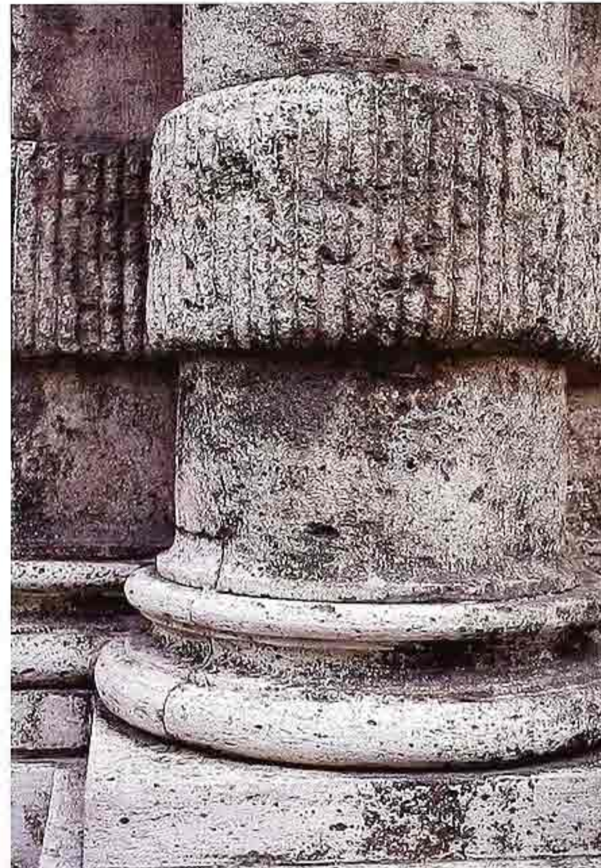
CP-32 Attic base of weathered column in volcanic stone with banded rusticated shaft
