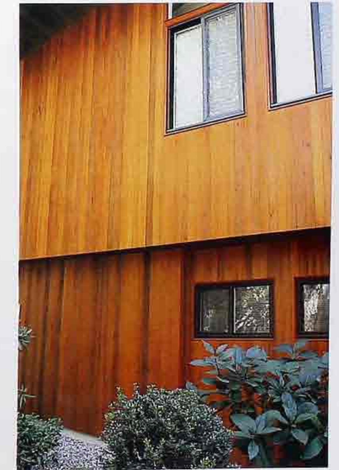
WA-50 Stained and sealed vertical siding with second-floor jetty and sliding metal-framed windows, modern house
