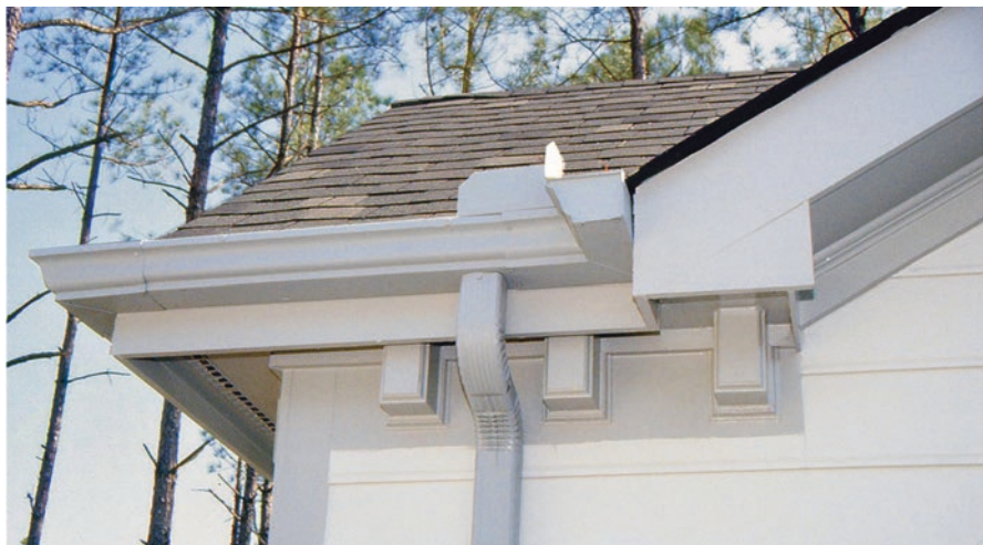
Fig. 7.8 Roof overhangs, trim, and fascia boards at the intersection of the roof and walls are often overlooked detailing opportunities, and builders of modest houses may only be able to justify these more elaborate transition details on a front gable or wall
