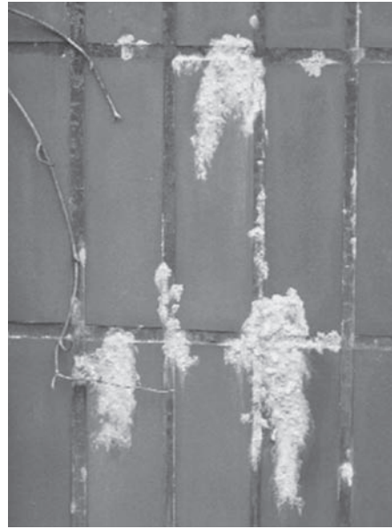
Fig. 37.6 Lime staining of brickwork.
