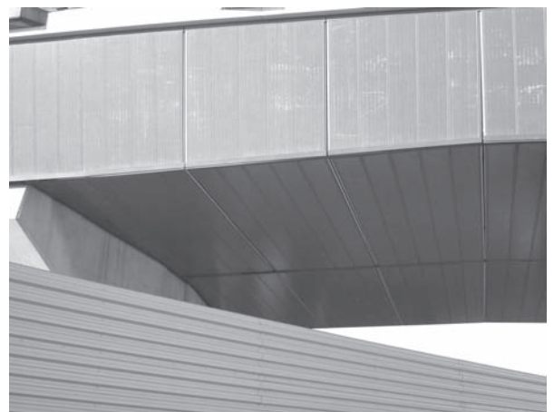
Fig. 43.3 Photograph of the enclosure on the approach span of the Dartford River Bridge (QE2) where it passes over the CTRL (before the train rails were laid) (Courtesy of AECON).
