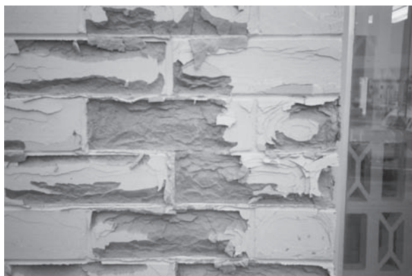
Fig. 37.4 Erosion due to frost attack.
