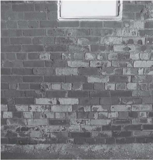
Fig. 37.5 Salt crystallisation damage to masonry together with associated soluble salt crystals (efflorescence).
