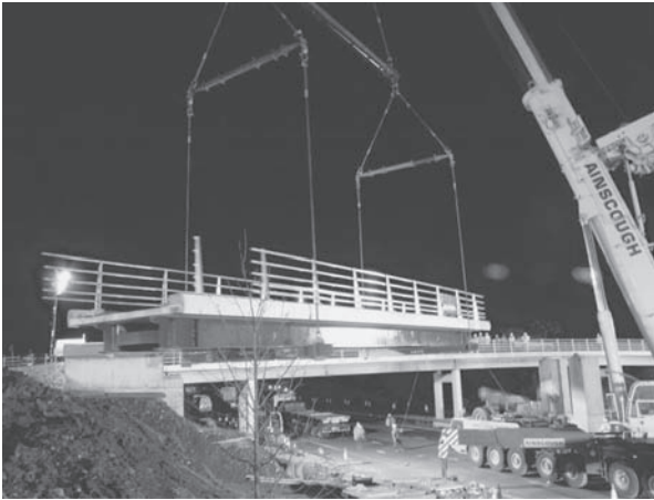
Fig. 43.5 Craning in the 100-tonne FRP deck onto the supports of the bridge over the M6 (Courtesy of Mouchel).
