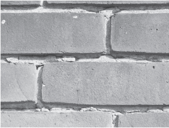
Fig. 37.2 Sulphate attack on mortar.
