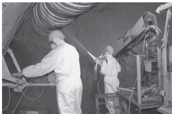
Fig. 50.3 Tunnel lining (steel-FRC) spraying equipment. Note the segmental extendable arm (top right, in partially retracted position) and computer control systems for laser guidance and monitoring (left). (Reproduced from the presentation accompanying Eddie and Neumann, 2004, by kind permission of the authors and Morgan Est Ltd/Beton-und Monierbau.)
