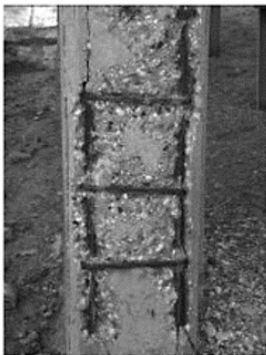
Figure 22. Pier reinforcement corrosion.
