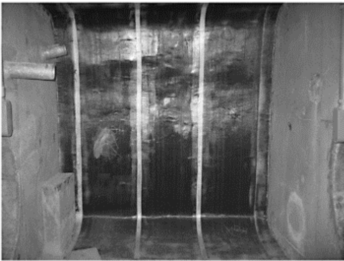
Figure 12. CFRP reinforcement of pier table web. Note 2-inch wide inspection strips between panels.
