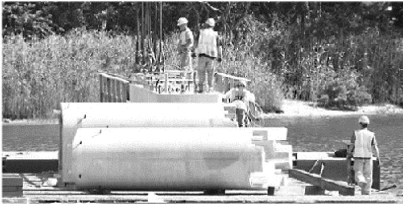
Figure 5. Precast pier columns and a cap beam have been loaded on a barge and are being prepared for erection.
