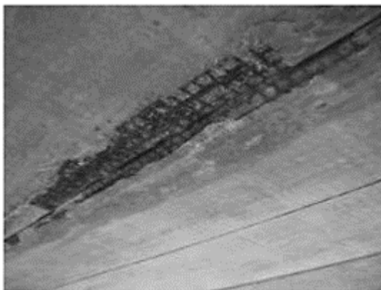
Figure 19. Cracks in slab.
