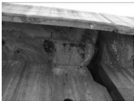
Figure 18. Leakage through Expansion joint.
