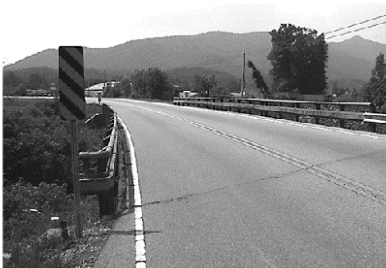
Figure 1. Above bridge before rehabilitation.
