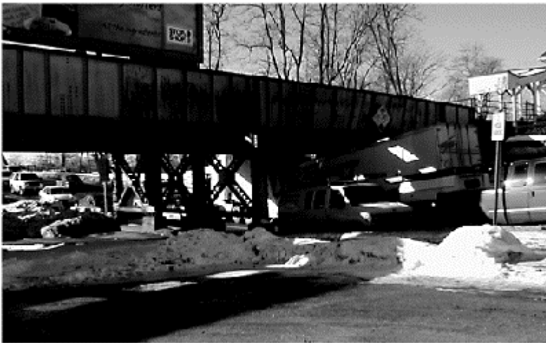
Figure 4. Substandard roadway clearance at Viaduct.
