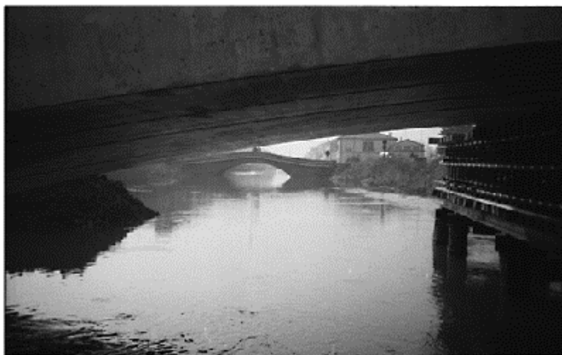
Figure 1. The erection of an arch bridge in the city of Padua; on the background an existing masonry bridge.
