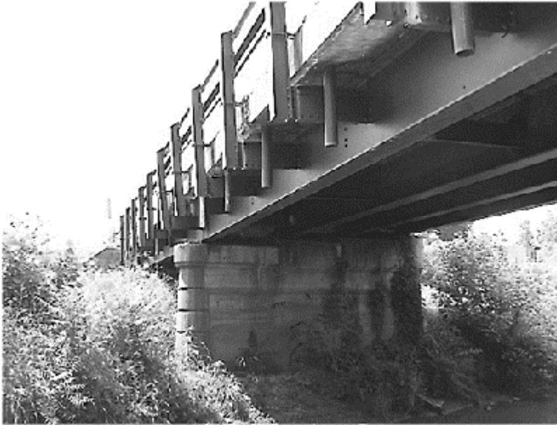
Figure 2. Below bridge before rehabilitation.
