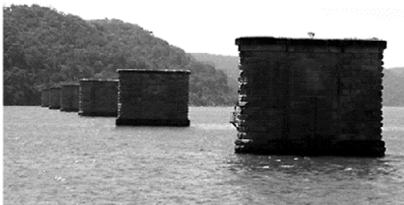
Figure 19. Original piers of the Hawkesbury Railway Bridge after the demolition of its superstructure in 1943 (Flickr, Penny T).
