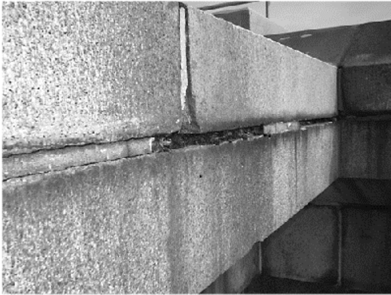
Figure 8. Mortar joint deterioration on Manhattan Tower.
