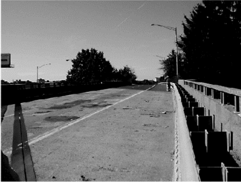
Figure 4. Deteriorated decks of the Route 1 Bridge over the Olden Avenue Connector.
