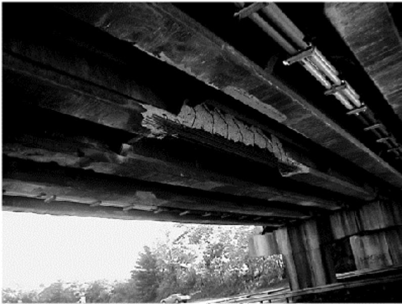
Figure 1. Exposed prestressing strands of damaged interior girder of Creek Road Bridge.
