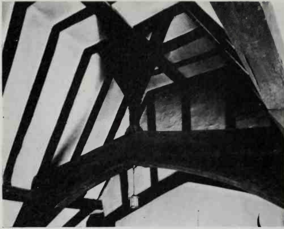
34. The 'king-post' introduced as a prop beneath the 'collars' of a 'close-couple' roof. The Old Parsonage, Marlow, Buckinghamshire
