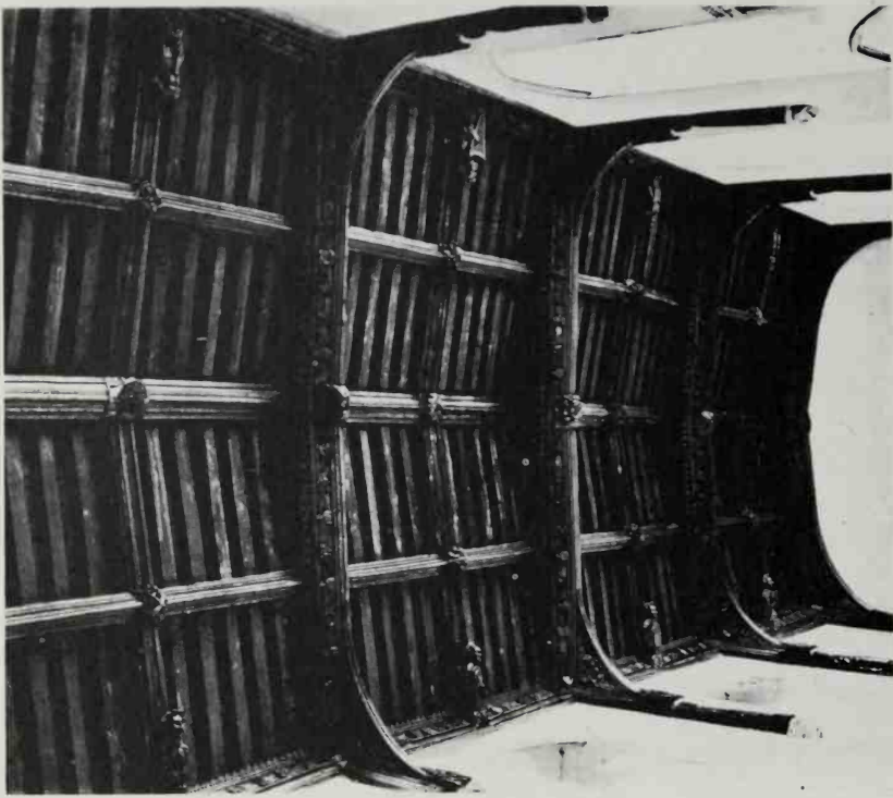
30. A Late Gothic roof of flat pitch having a lead covering. Harrow church, Middlesex
