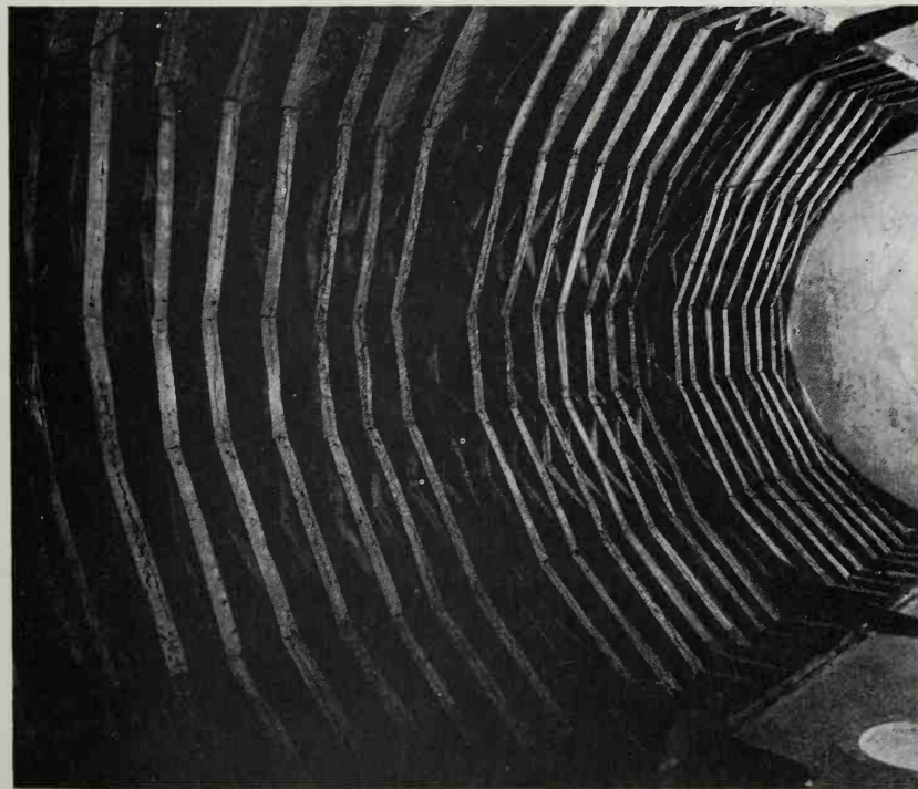
27. Typical mediaeval roof of closely-spaced 'couples', in this example well braced. Great Bentley church, Essex
