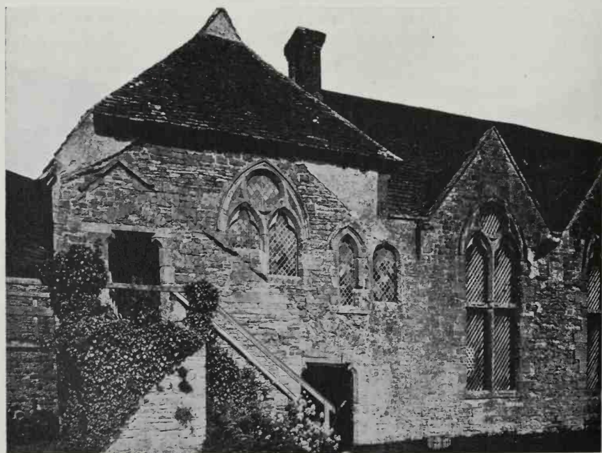
116. Traces of the roof of the chamber stair can be seen passing up the gable wall of this house attached to the end of a hall. Stokesay Castle, Shropshire
