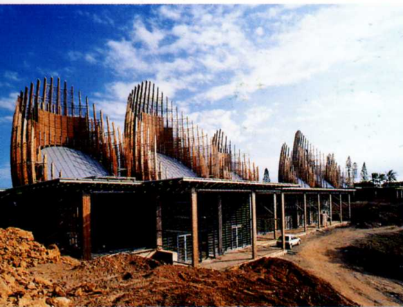
The enclave on its small peninsula permits the sea to be seen from the two main facades. The smaller one looks towards the interior of the island.
