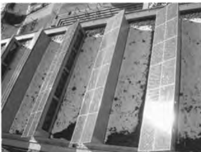
23.76 kW photovoltaic panels system. Academy of St. Francis of Assisi, Liverpool, Buro Happold
