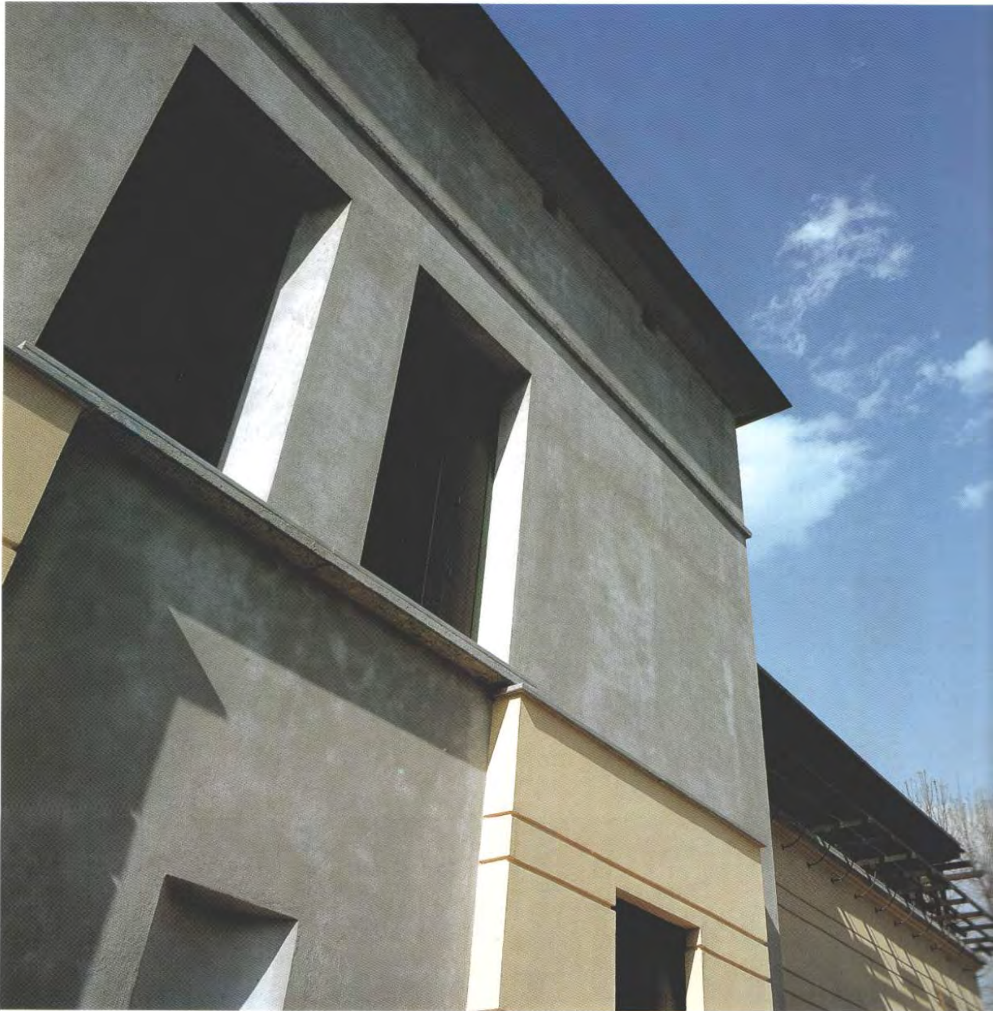
The photos reflect the traditional dichotomy in the treatment of details and finishes between the more public front portion, which overlooks the street, and the rear facade, which is more secluded and plainer.
