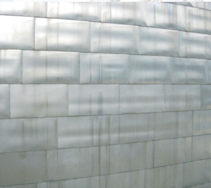
Frank Gehry, Guggenheim Museum, Bilbao, Spain, 1997 Titanium cladding of the museum envelope, acquiring patterns of use, atmosphere, climate and time.
