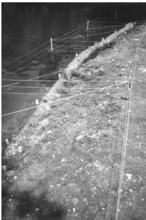
Figure I.16.15 Waterfowl exclusion fencing and netting in restoration areas.
