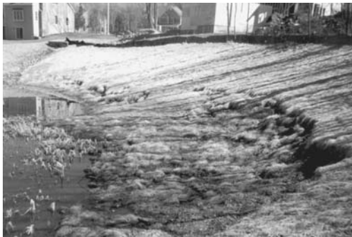
Figure I.2.4c A close look of the slumped slope.
