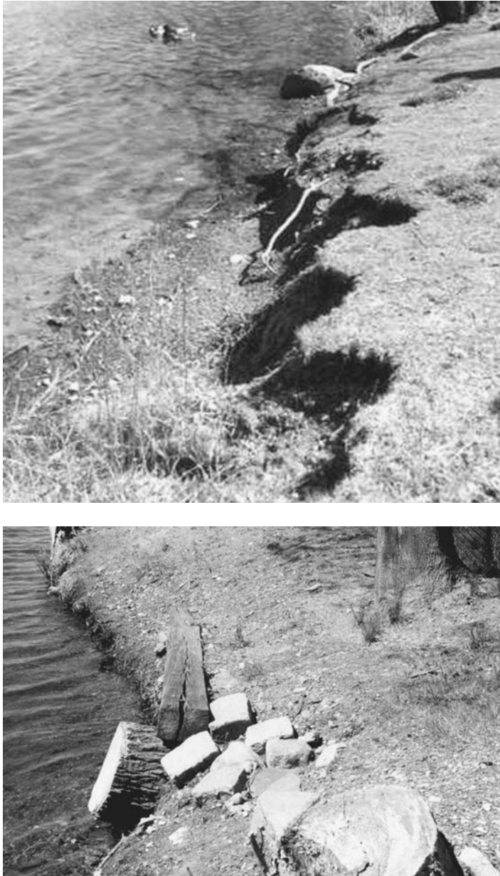
Figure I.16.4 Shoreline regions of Chandler Pond exhibiting substantial erosion.
