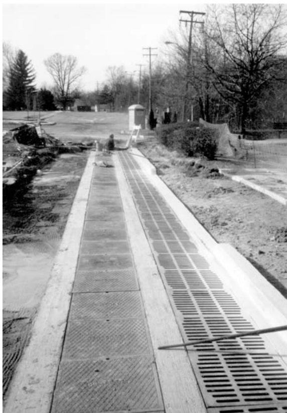
Figure II.9.6 Linear sand filter retrofit to urban area for stormwater management, Wayne, MI. (Courtesy of Rouge River National Wet Weather Demonstration Project, Detroit.)
