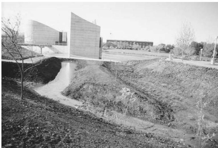
Figure I.12.3 Construction of the central berm designed to increase the flow path distance for nutrient removal in the treatment wetland. This area will also function as an avenue to bring students into the wetland for study. (Color version available at www.gsd.harvard.edu/watercolors . Password: lentic-lotic.)
