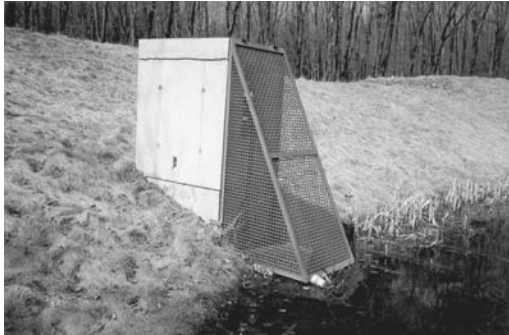
Figure I.2.4b A close look of the outflow control structure in Figure I.2.4a.
