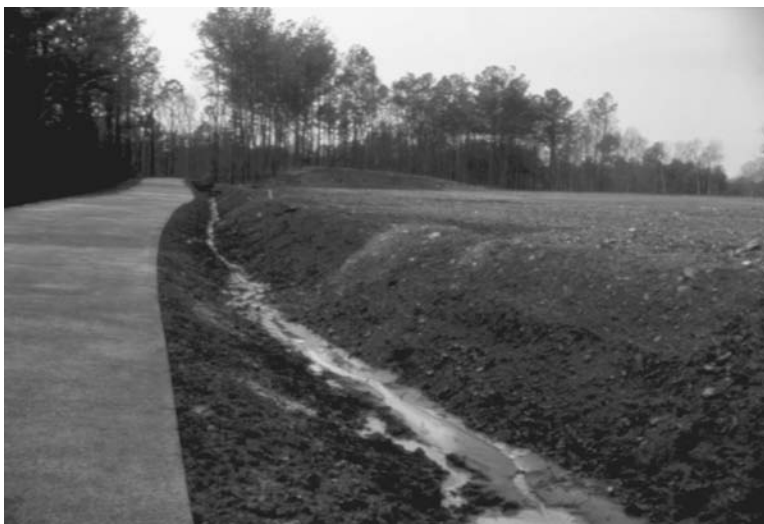
Figure I.1.19 A porous concrete road in Webb Bridge Park, Alpharetta, GA. (Color version available at www.gsd.harvard.edu/watercolors . Password: lentic-lotic.)
