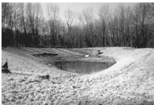
Figure I.2.4a Distant view of a detention pond with upper left slope slumped, Marlboro, MA.
