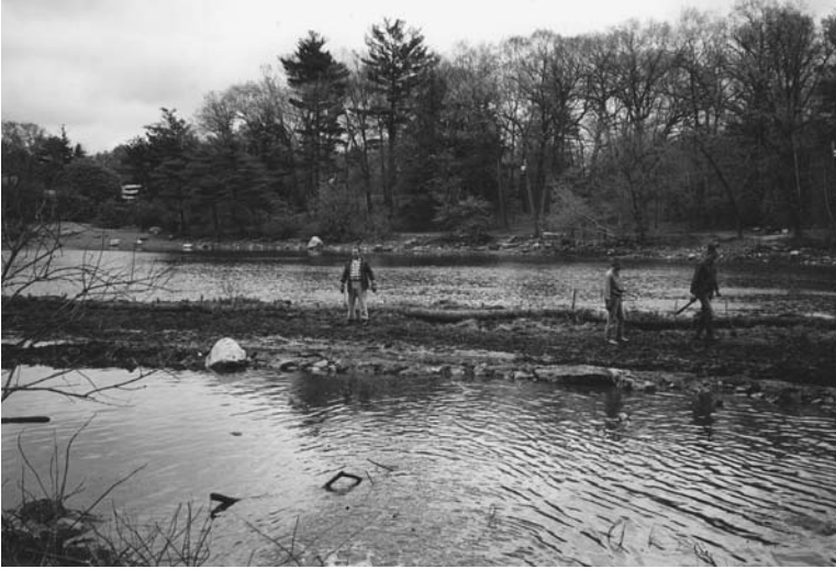
Figures I.11.17 Planting the wetland at Hill's Pond. (Photo by Clarissa Rowe.)
