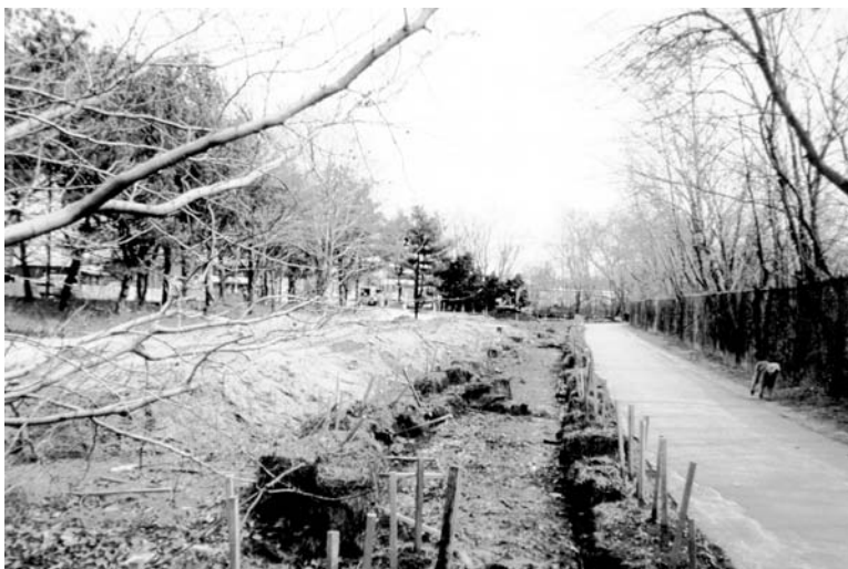
Figure II.4.19 Berm construction along new bikeway, April 2001. Perimeter Road on right along reservoir fence, bikeway on left (behind berm), and Fresh Pond Parkway on far left (behind trees and Jersey barriers).
