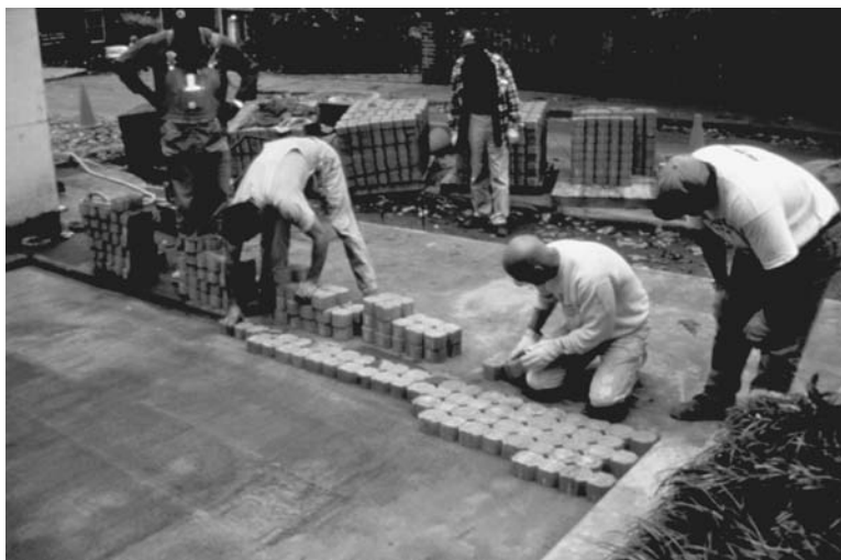
Figure I.1.17 Construction of a porous paver driveway in Athens, GA. (Color version available at www.gsd.harvard.edu/watercolors . Password: lentic-lotic.)
