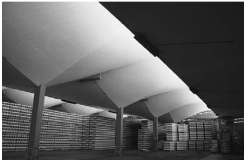
12.3 >The tilted HP umbrella shells of Candela's Bacardi storage space is based on a series of hyperbolic paraboloid shapes.
