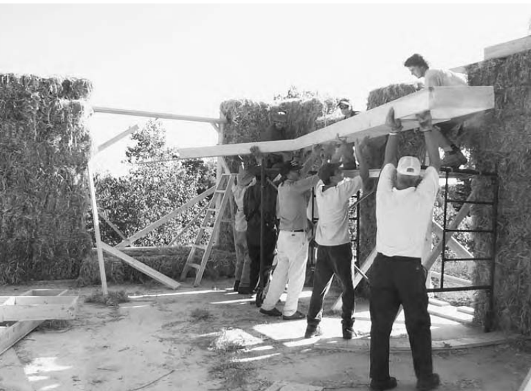
18.29: The top plate that was carefully laid out on the foundation is now raised onto the walls.
