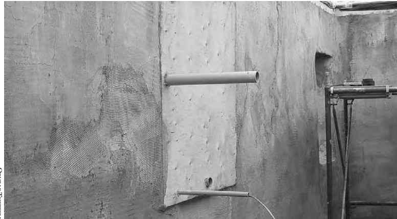
18.16: This plywood panel mounted to the wall allows conduit for wiring to pass through the wall, and will provide a mounting place for the electrical panel.
