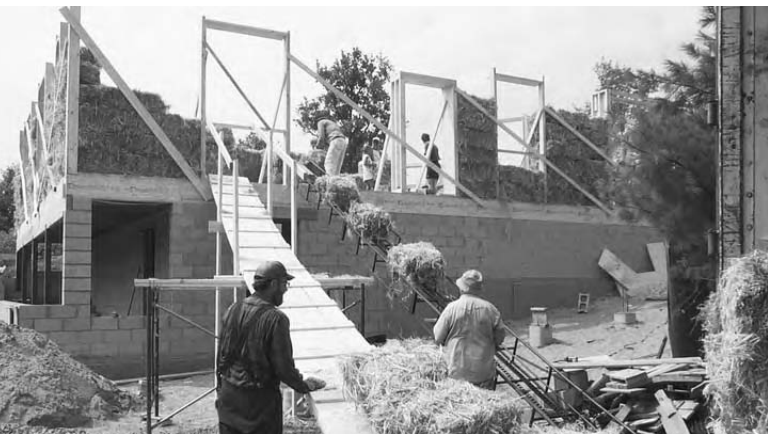
3.7: From the back of a transport trailer onto an elevator and immediately into the wall: the best way to do it!
