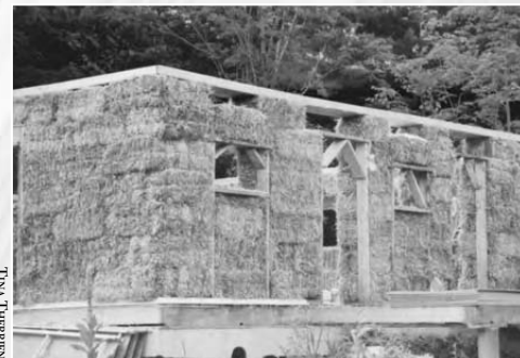
18.28: Leave voids over windows and doors until after the top plate is on and the walls have been compressed.
