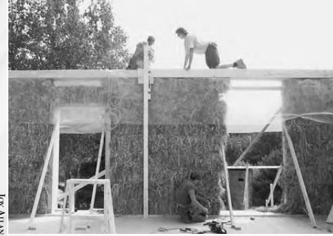
18.26: The tension wires are pulled with a come-along and fence stretchers. The height stick hooks over the top plate, providing you with a reference for both vertical plumbness and overall wall height. Notice how the walls are protected by a sheet of plastic over the top plate.
