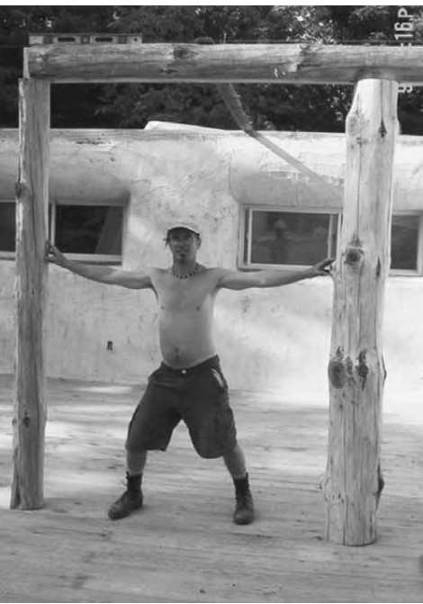
8.7: The load-bearing walls of this building are plastered, then the central post and beam structure is built to the finished height of the walls.
