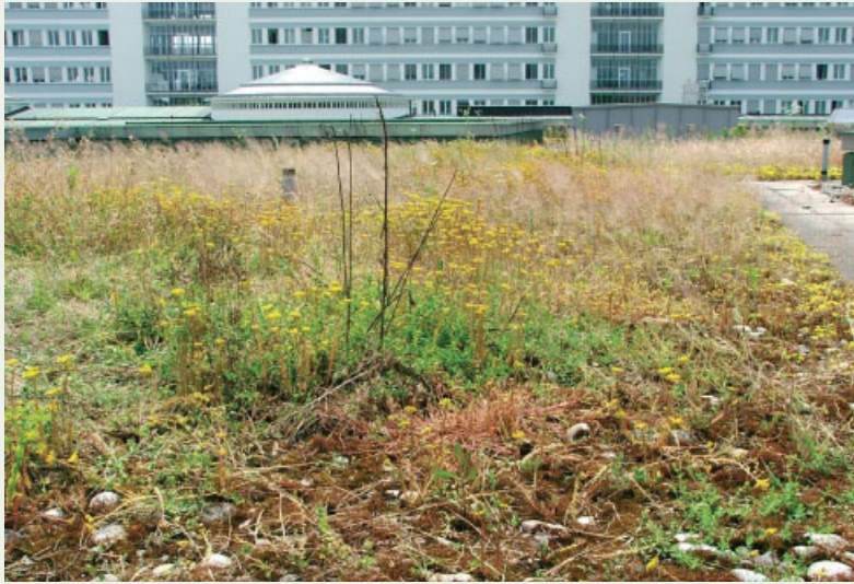
Living roof on the Rossetti Building of the Cantonal Hospital of Basel. The habitat is based on unusual riverine gravel grassland and is used by a diverse range of uncommon invertebrates and birds.
