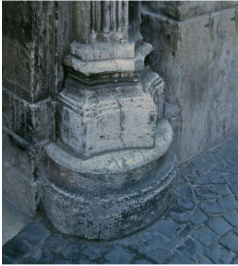
Francesco Borromini, Palazzo di Propaganda Fide, Rome, 1662 Detail of door post: concavity standing on convexity.
