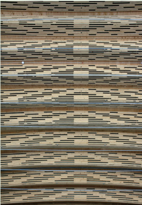
Wave-like forms of 2x4 timbers are located between the primary structural elements of the Oval's roof, providing a textured soffit and an acoustic baffle.
