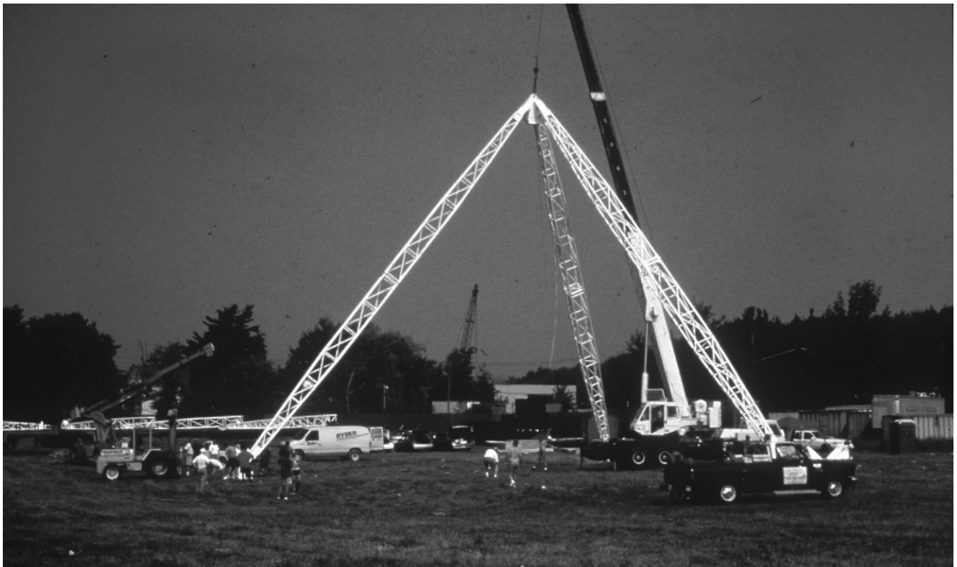
Fig. 12.9 Once in position the base of the leg is fixed onto its foundation which is located by helical ground anchors.
