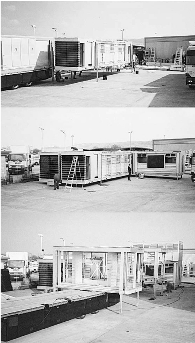
Fig. 5.13 Erection process. Top; pod 1 is in place and pod 2 is being placed alongside, middle; pods 1, 2 and 3 in place, bottom; pods 1-4 in place and pod 5 being positioned.
