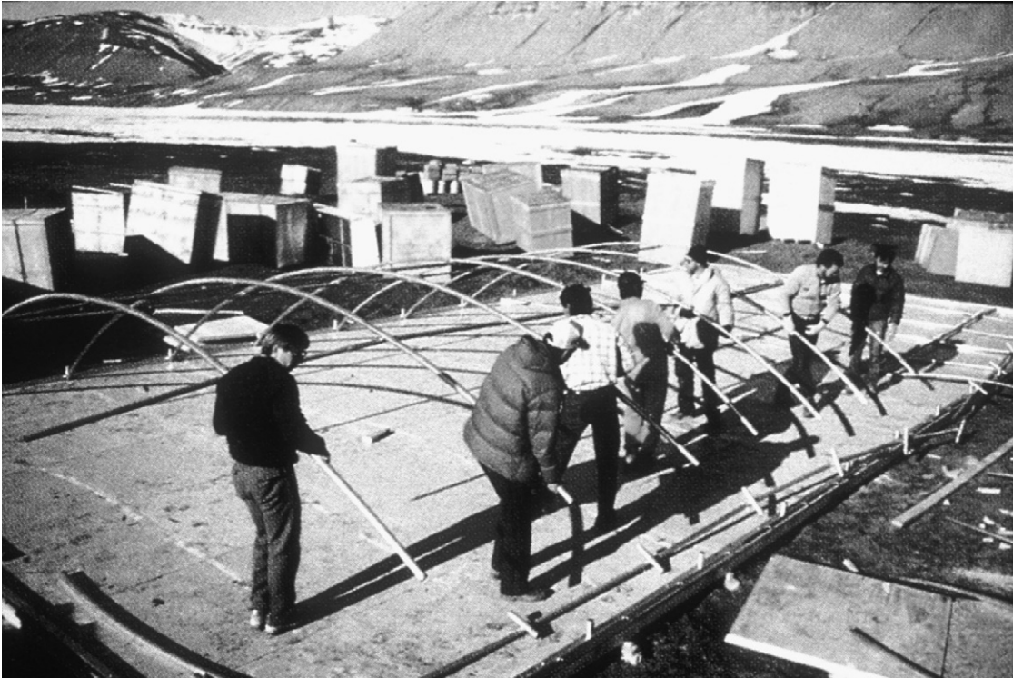
Fig. 16.2 ‘Series 4’ erection procedure. In this project an insulated prefabricated plywood floor has been laid. The floor level framing is in place and erection of the arched structure is underway.
