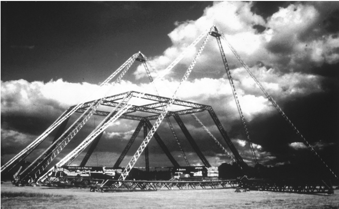
Fig. 9.3 The tripod structure that supports the apex tension membrane is erected separately from the main, heavier structure which supports the side membrane panels and the internal performance equipment.
