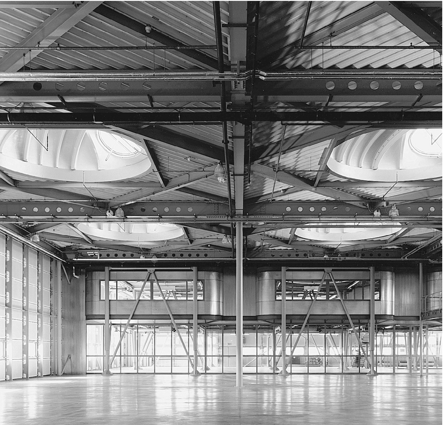
Fig. 8.9 Internal view. The factory floor is completely clear of services which are distributed at roof level.
