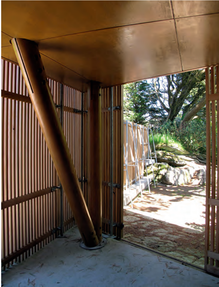
Feary + Heron, Plant Room, Eagle's Nest, Zennor, Cornwall, England, ongoing View along the timber screen to the courtyard beyond. The column is cantilevered to preserve access to the folding doors to the left that open onto the tank-top deck.
