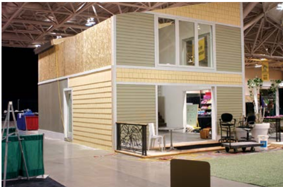
TOP AND BOTTOM: The house was initially erected at the Minneapolis Convention Center for a home and garden show. The first panels went up at 10:00 A.M. and the structure was complete by 1:30 P.M. The house was left unfinished so visitors could see the construction components.
