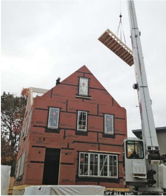
The Westport Beach House under construction. Photo courtesy of Sellars Lathrop, LLC.
