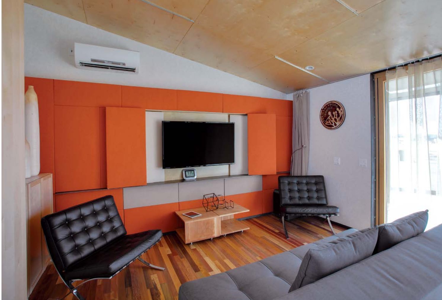
The wall that houses the media center doubles as a large storage area. The mini-split heat pump above the storage wall provides cool air when needed.
