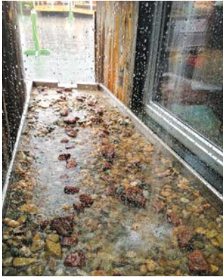
LEFT: The catch basin, where rainwater is collected, is located behind the entry. Photo courtesy of Eric Weber/UNLV Design Build
