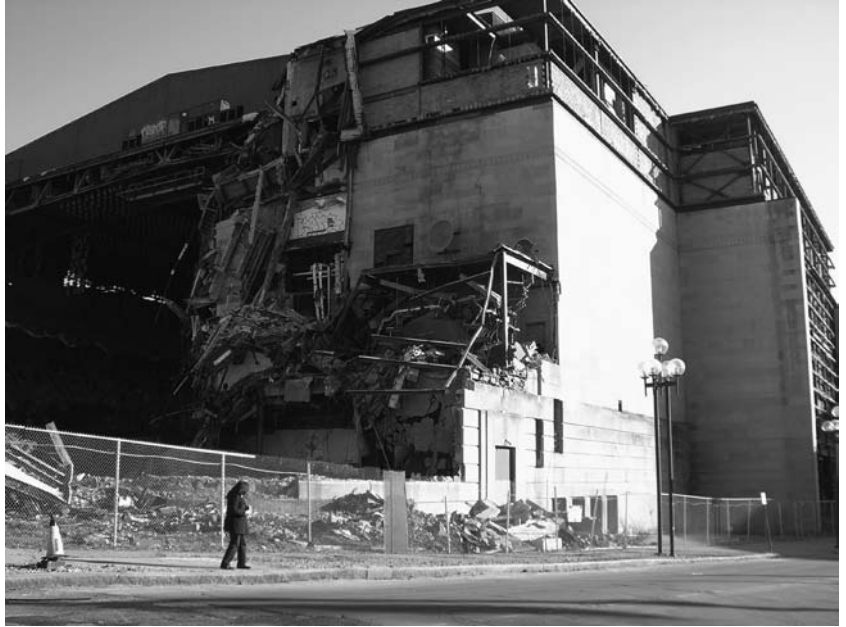
Figure 12.2 The unmaking of the Buffalo Memorial Auditorium. The Aud was built in 1938 and for years was home to the Buffalo Sabres. It is being demolished to create a potential development site. Photograph by author.
