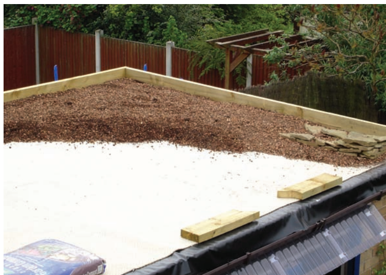
The green roof during construction, with waterproof liner, protective old carpet on top, and substrate. Photo by Jeff Sorrill
