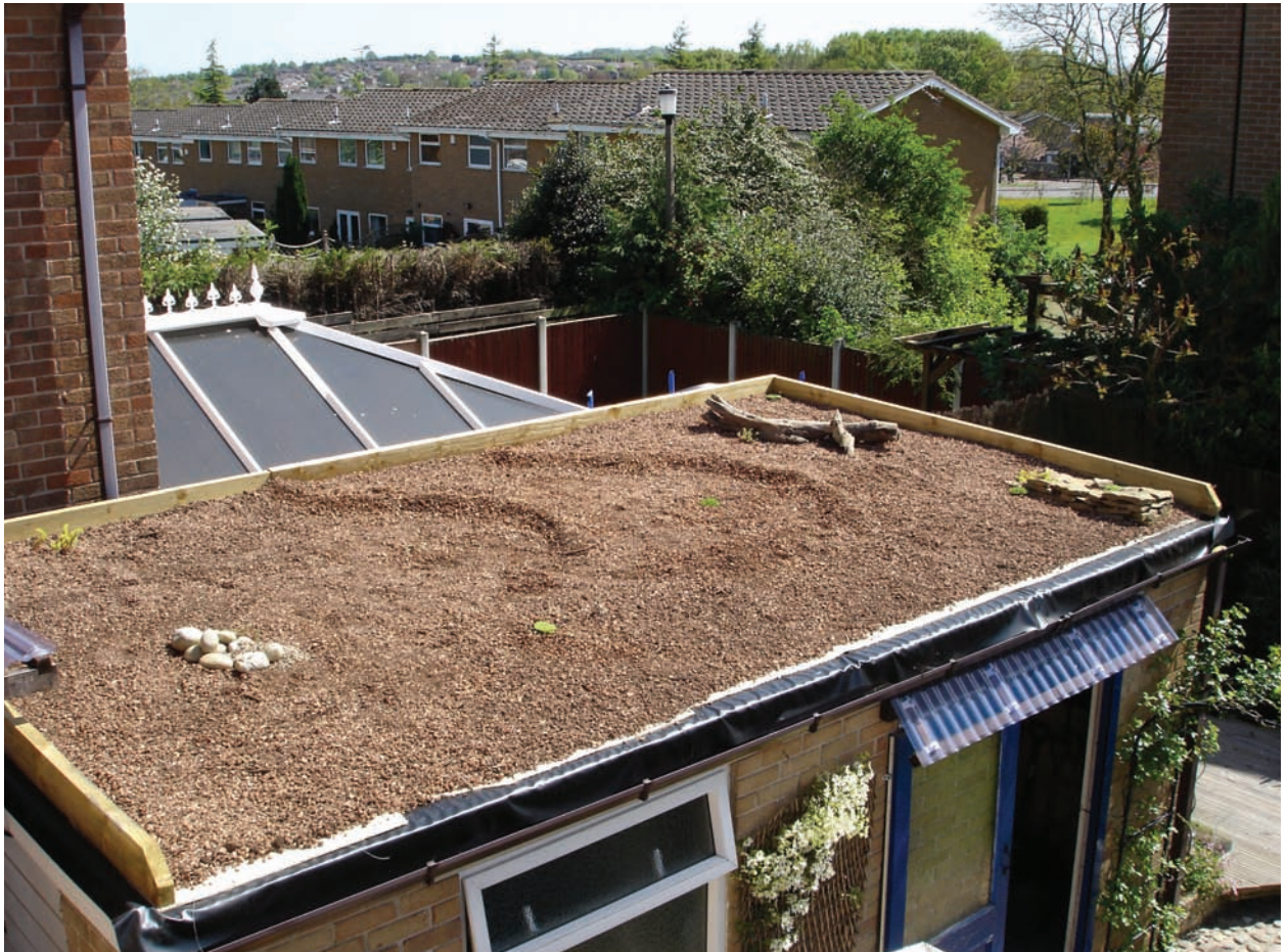
The completed roof, with mounding, logs, and stones. Photo by Jeff Sorrill
