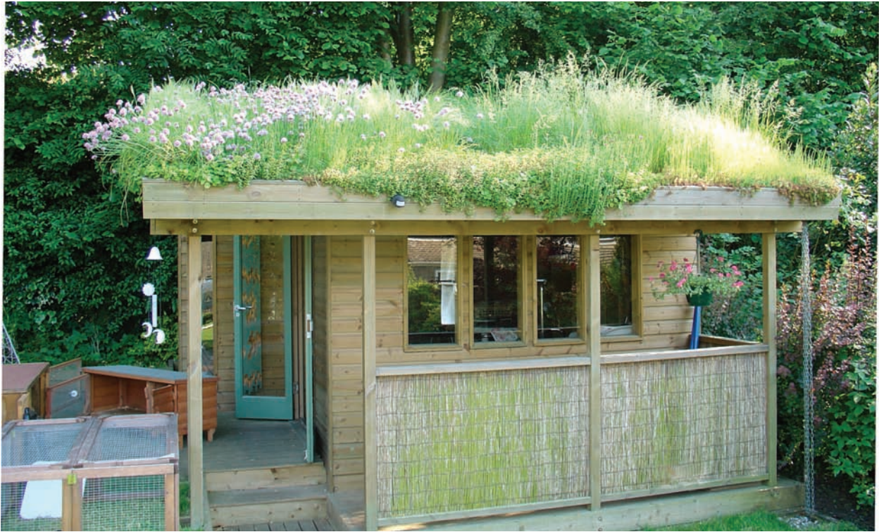
The roof vegetation is very lush as a result of feeding and watering. Photo by John Little
