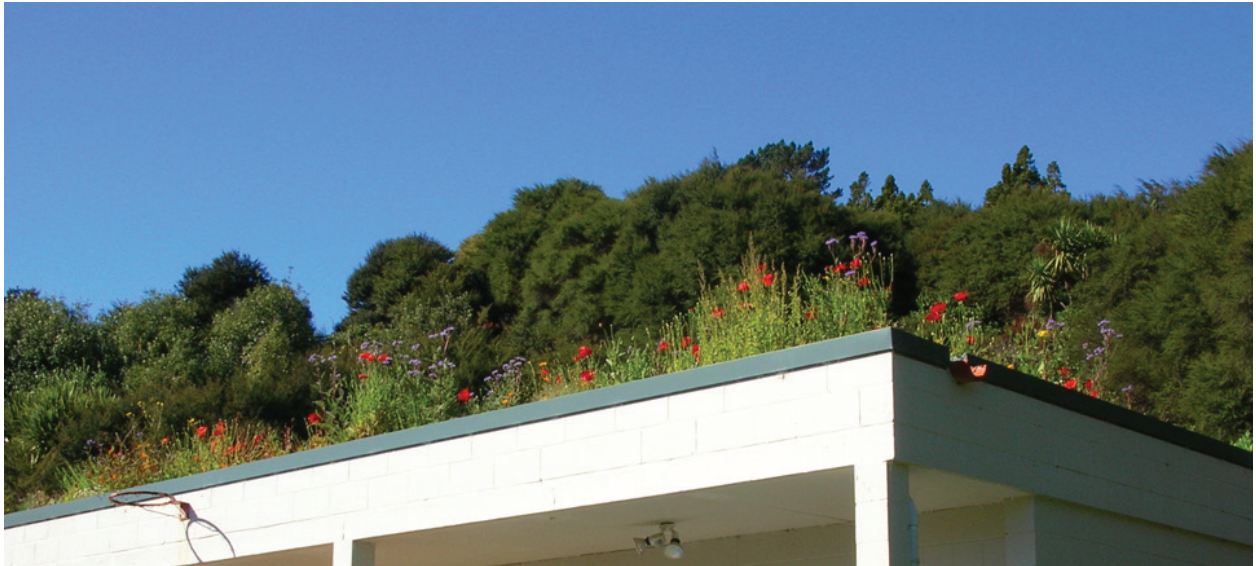
The green roof was planted with colourful flowering plants. Photo by Doug Johnson
