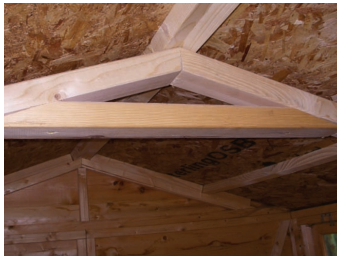
Top left: An existing typical lightweight garden shed can be strengthened to enable it to take a green roof. Each wall panel is braced with horizontal and diagonal batons. Photo by Green Estate Ltd.
