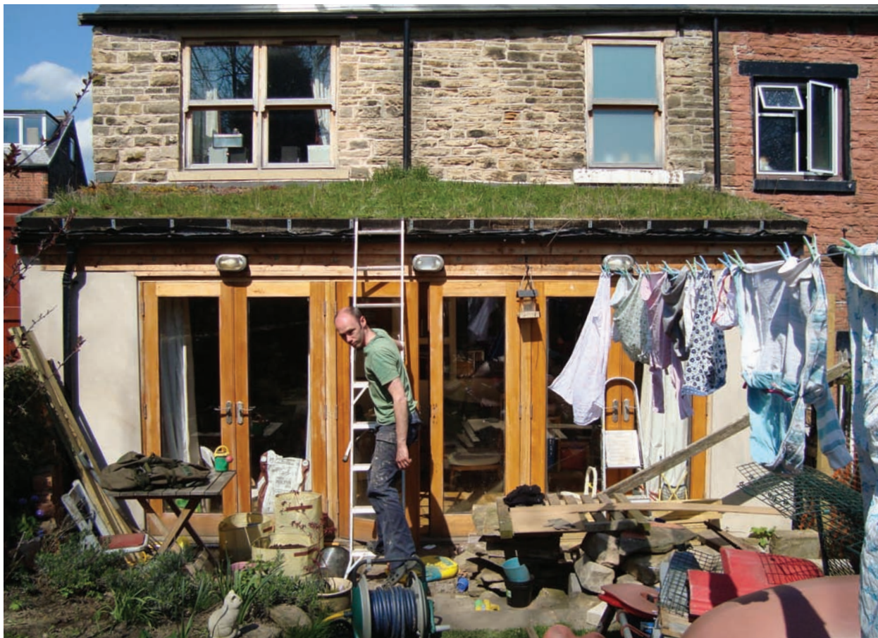
Ben with his extension roof. The downpipe from the roof gutter empties directly onto the green roof, providing additional water when it rains. Photo by Green Estate Ltd.
