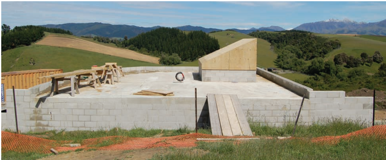
The poured concrete slab roof ready to receive the green roof. Photo by Rhys Taylor
