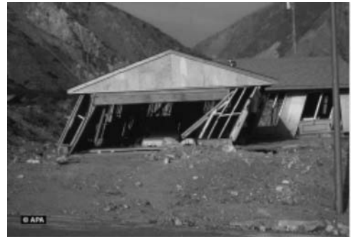
(c) Lack of adequate racking strength results in failure (photo courtesy of APA, The Engineered Wood Association)
