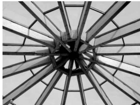
(f) A roof structure (photo courtesy of Lilleheden Ltd, a member of the Glued Laminated Timber Association, UK)
