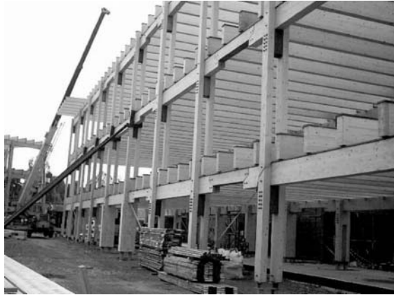
Fig. 8.5. Beam and post construction using beams inserted between spaced column shafts (photo courtesy of Constructional Timber Limited, a member of the Glued Laminated Timber Association).
