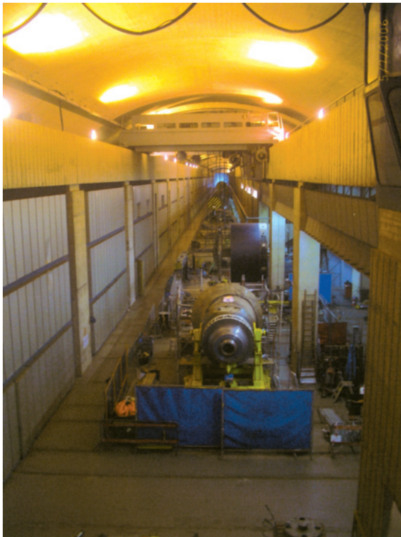
Figure 11.9 Tidal barrage and turbine hall, La Rance, Normandy
