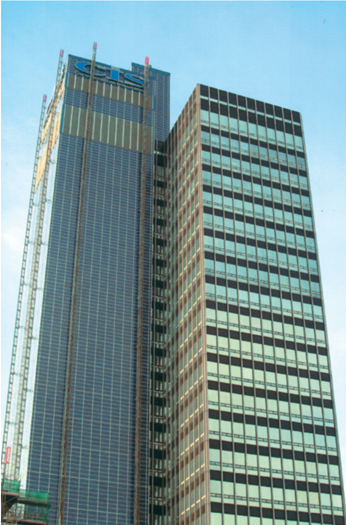
Figure 15.7 CIS Tower, Manchester with retro-fitted PVs (photograph: Pam Smith)
