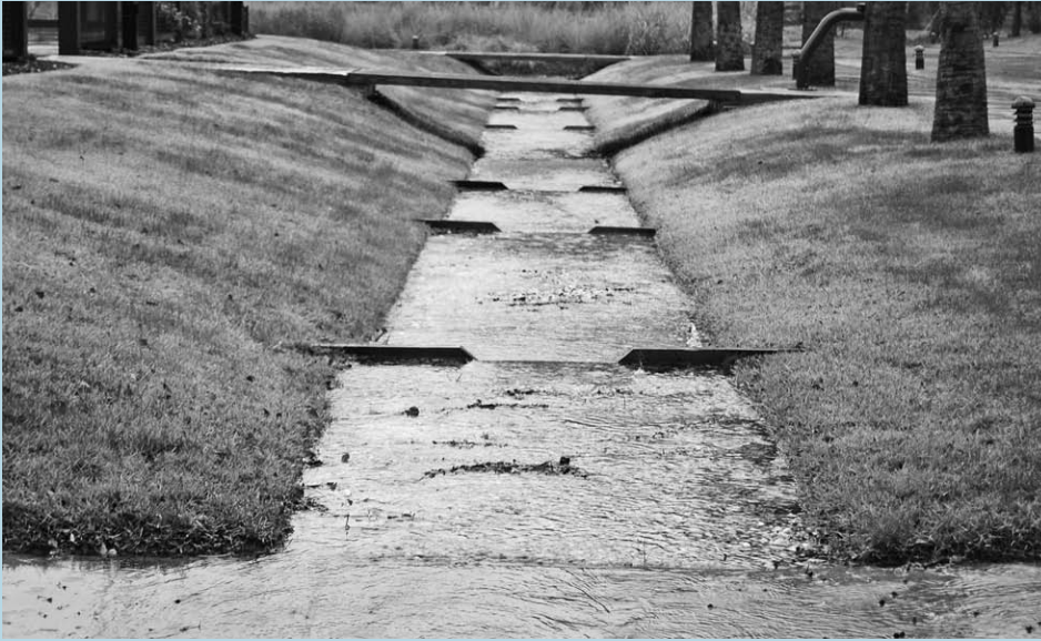
Figure 7-4 As a light imprint technique, this gravel swale channels runoff during a storm at Habersham. Duany Plater-Zyberk and Company, Charlotte, NC
