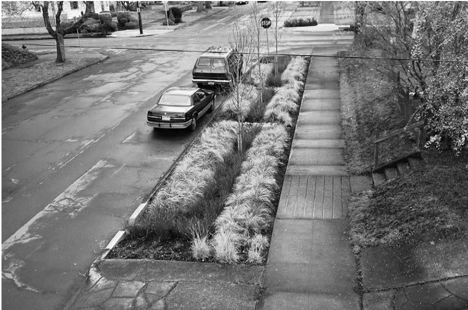
Figure 1-27 A Portland, Oregon, “green street” rainwater garden captures runoff and allows a gradual discharge into the ground. However, the rainwater infrastructure still partly connects to the sanitary waste piping, which degrades the performance of both systems. Paul Crabtree
