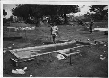
Septic tank used as water tank for building supply.
