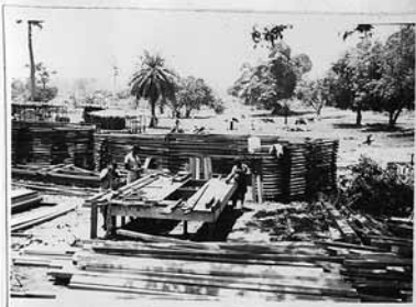
Jigs for cutting rafters before assembling with stocks of completed trusses in background.
