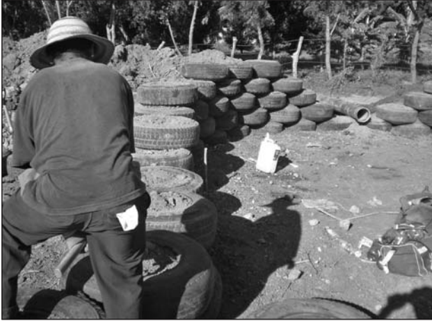
Bryan Roberts of Eco-Tech Construction is in the middle of building an earthship in Manatee County, Florida.
