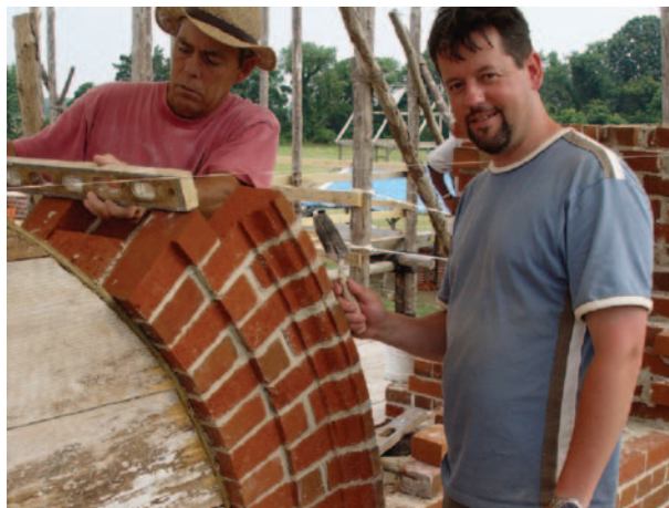
Figure 56 Constructing the upper half of a large bullseye window, of cut-molded voussoirs, to the west elevation of St. Mary’s Chapel. (Courtesy of Price Masonry)
