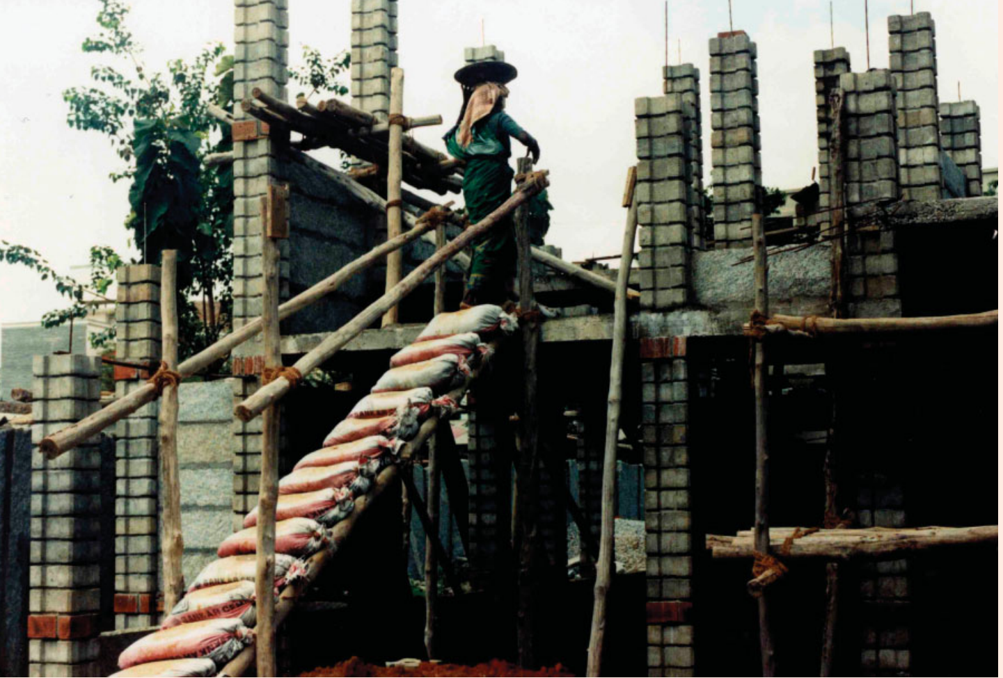
Shilpa Sindoor building site. Coordination of curing times and phased building with alternating masonry and concrete systems creates complex project management conditions, overcome by the abundance of migrant labour. Workers are often employed as entire families, with women (at lower pay rates) constituting the bulk of the work force. Construction sites are often playgrounds for labourers' children, places where their parents forge an ironically domestic realm.
