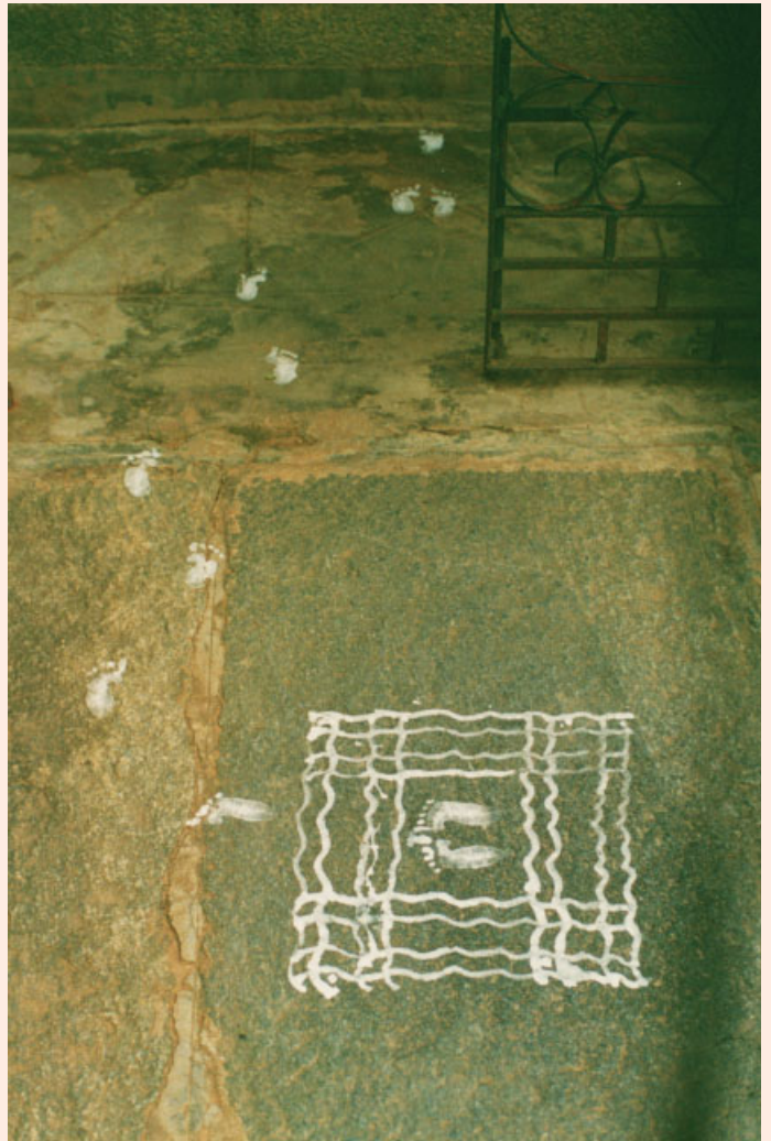
Locally quarried granite slabs span ditches dug for water and waste lines. Like ice in the tundra and sand in the desert, the abundance of stone in this region inspires structural experimentation, in this case setting a building material in tension that is typically used in compression.
