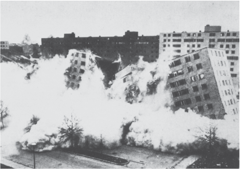
Partial demolition of Pruitt-Igoe housing complex (Leinweber, Yamasaki & Hellmuth, 1950–54), St. Louis, Missouri, 1972. Photograph by Lee Balterman.
