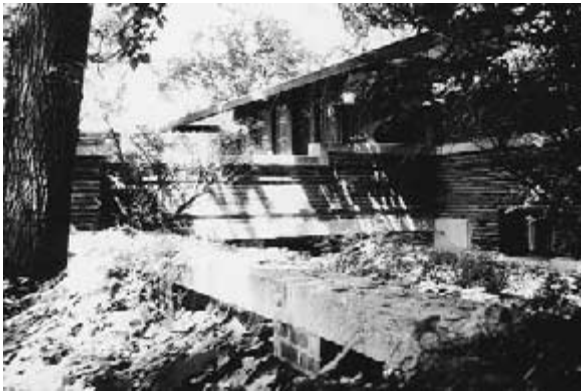
Figure 3-35 A 1996 photograph at the Cheney residence shows exposed brick piers and masonry base, prepared for privacy walls that were never completed. (Photograph by Charles E. Aguar. © 2002 by Berdeana Aguar.)
