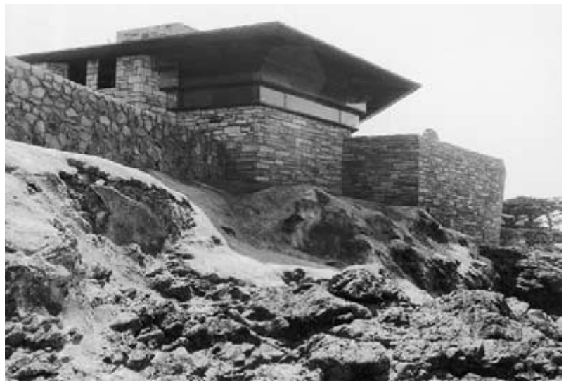
Figure 8-34 Oceanside view of Walker House shows extensive erosion of rocks that serve as its foundation. (Photograph by Charles E. Aguar. © 2002 by Berdeana Aguar.)
