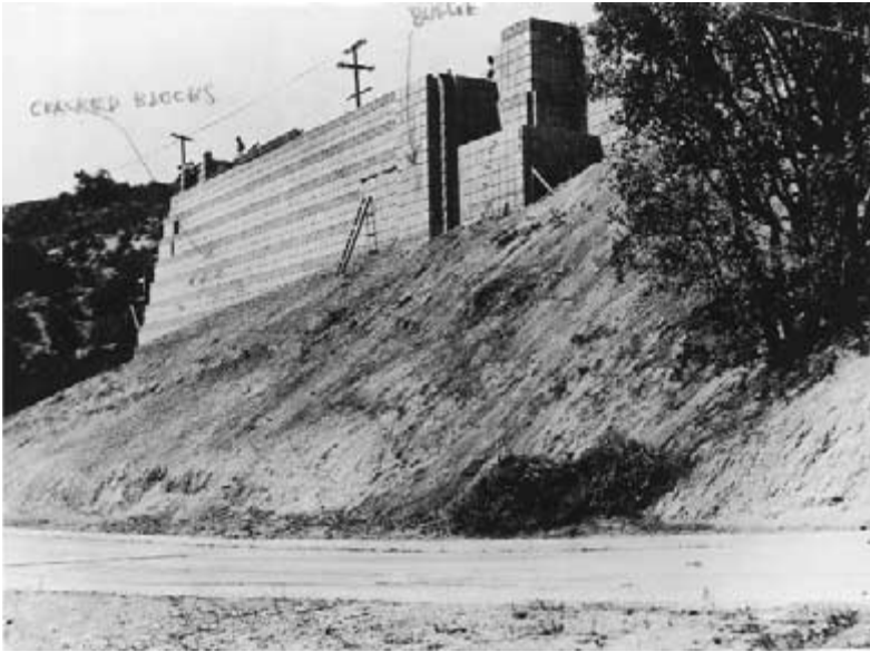
Figure 5-21 A photograph from the Frank Lloyd Wright files showing the Ennis retaining wall before the project was completed was marked with the notations “cracked blocks” and “bulged.” (Courtesy of The Frank Lloyd Wright Archives, Scottsdale, Arizona. )
