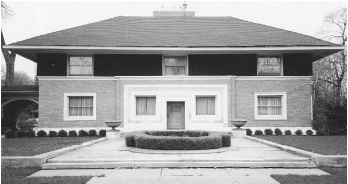
Figure 2-13 A 1992 photograph of the Winslow House reflects the negative effect of deviating from Wright's design intent. (Photograph by Charles E. Aguilar. © 2002 by Berdeana Aguilar.)
