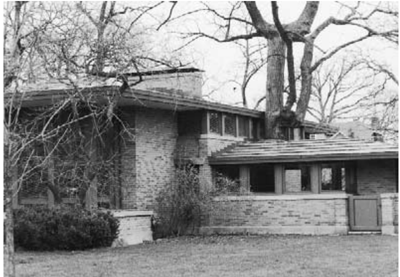
Figure 3-79 A view of the Isabel Roberts House (1908) in River Forest, Illinois, shows a specimen English Elm tree still growing through the roof of the porch almost a century after construction. (Photograph by Charles E. Aguar. © 2002 by Berneana Aguar.)
